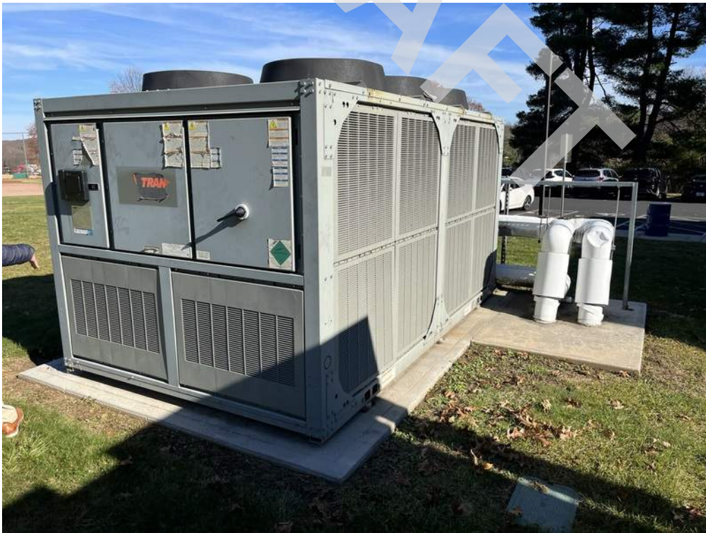
26 - A pad mounted air-cooled chiller located on the exterior of the building provides chilled water to the building.
