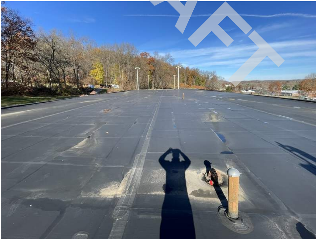
8 - The roofing system consists of an EPDM (ethylene propylene diene terpolymer) membrane.
