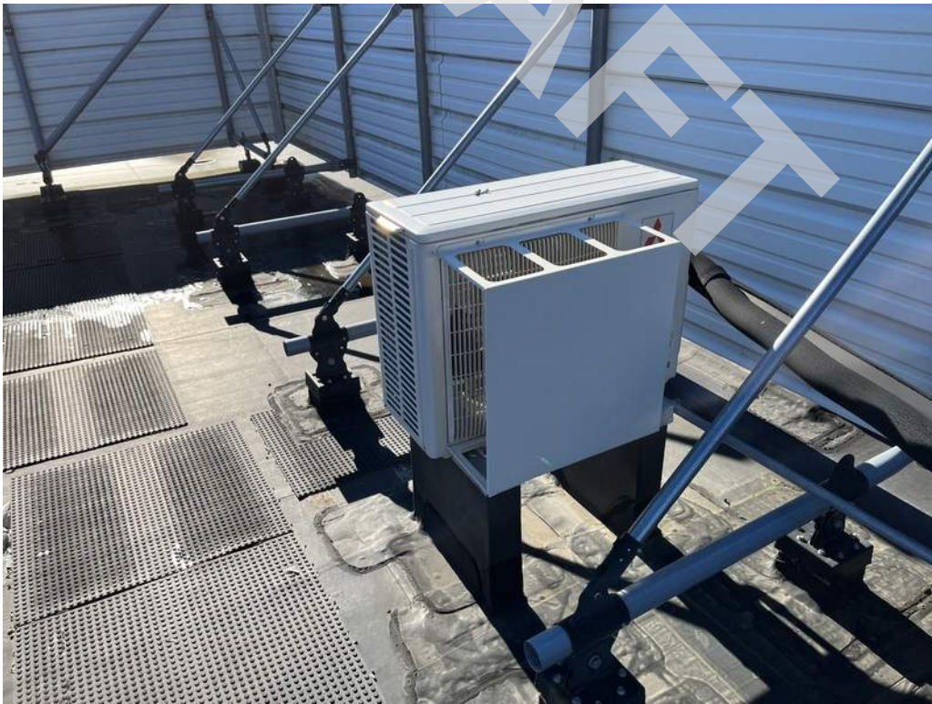
24 - Split system air conditioning units are located on the roof and provide cooling to portions of the building.
