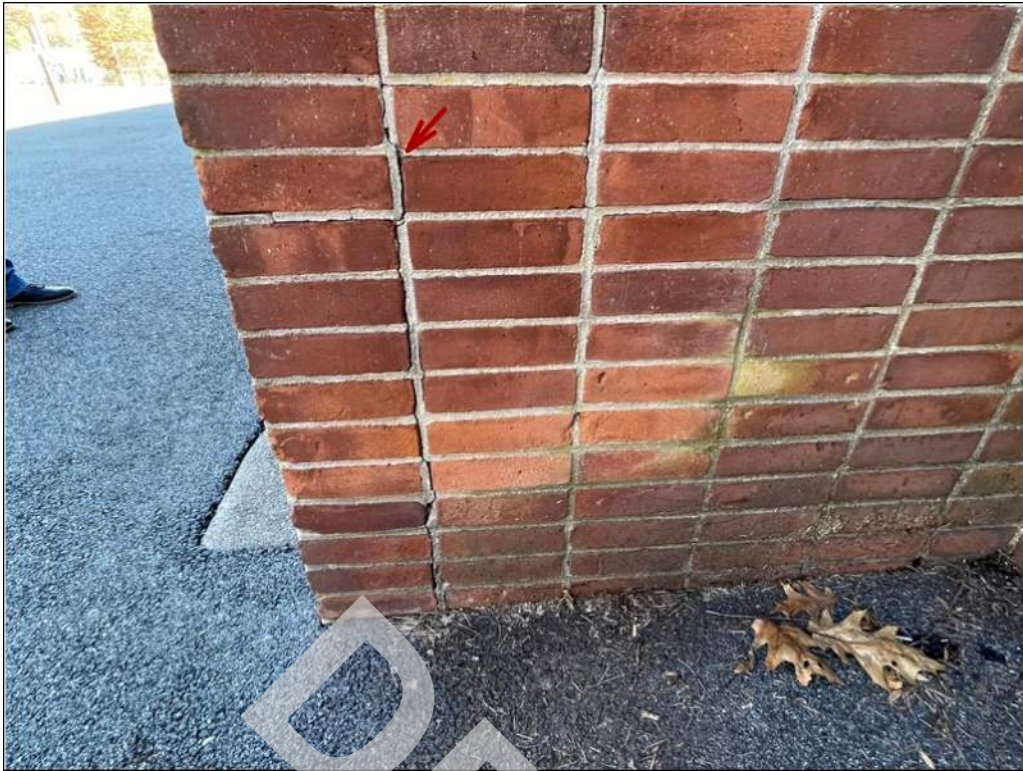
15 - Brick masonry unit mortar joints have cracked.
