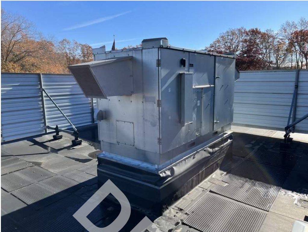
23 - An energy recovery ventilator provides conditioned ventilation air to portions of the building.
