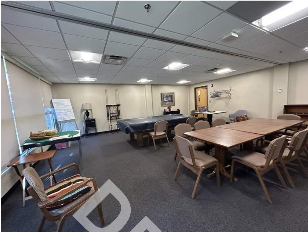
35 - At the Senior Center Game Room, the pool table and seating tables do not provide knee and toe clearance.
