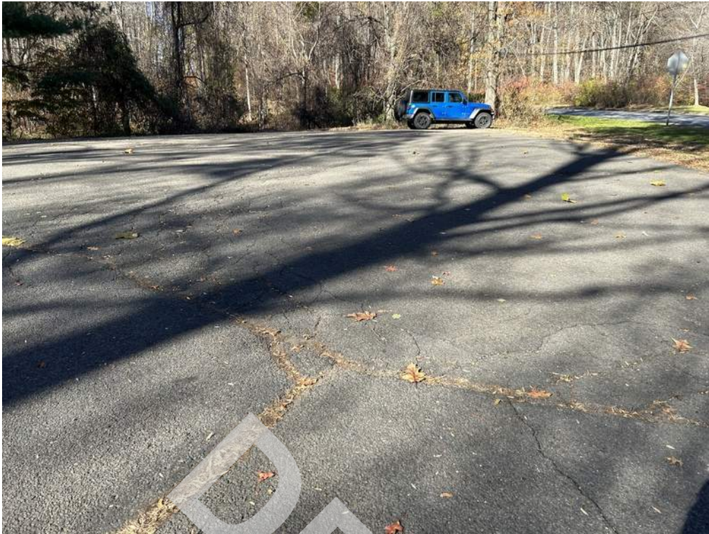
5 - Longitudinal and alligator cracking was observed at the second additional parking lot provided.
