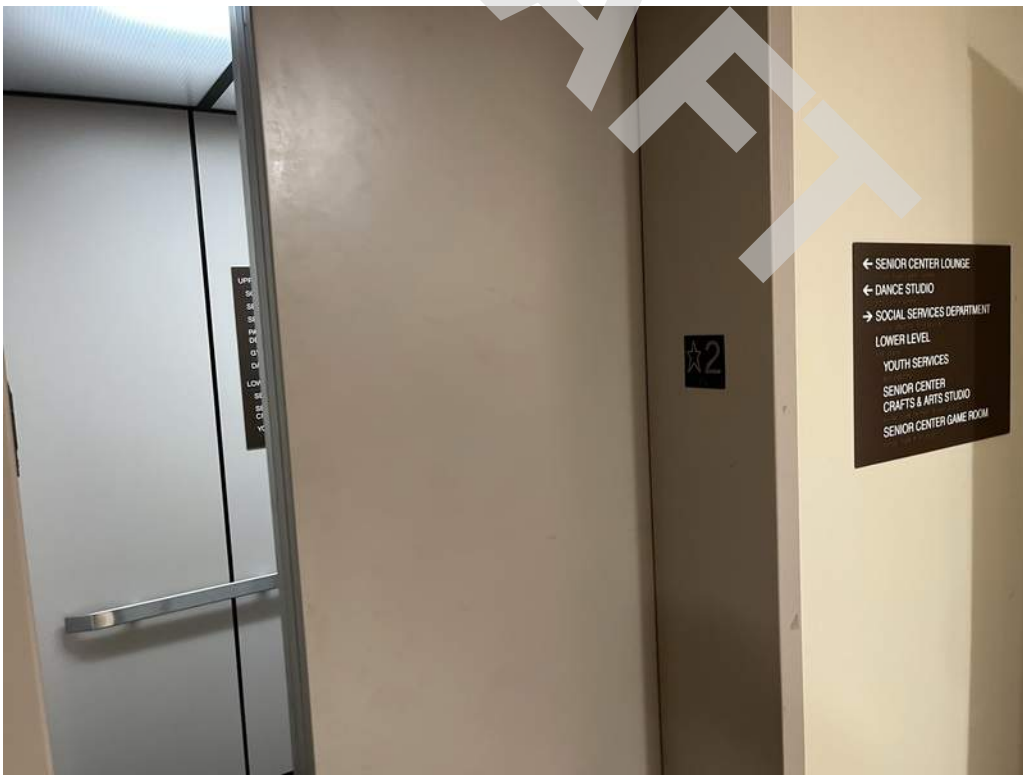
30 - The building is provided with a Kone hydraulic passenger elevator located in the east wing of the building.
