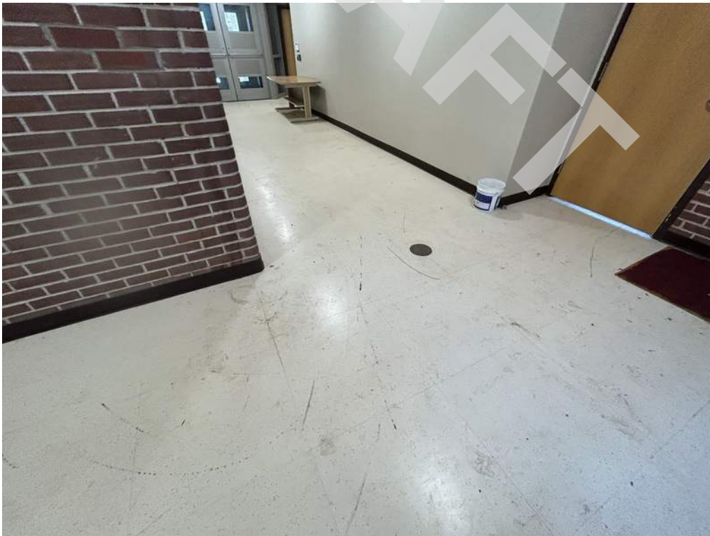
20 - Stained vinyl composite tiles were observed at the public corridor, on the south wing of the building.
