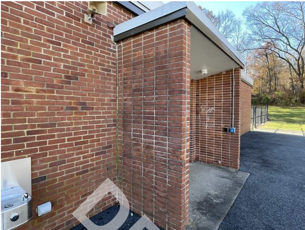
13 - Areas of the brick masonry unit wall have organic growth and deterioration at the mortar joints.
