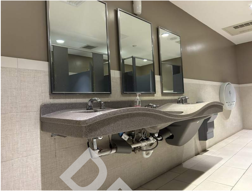
39 - Scald guard protection is not provided under the sinks.
