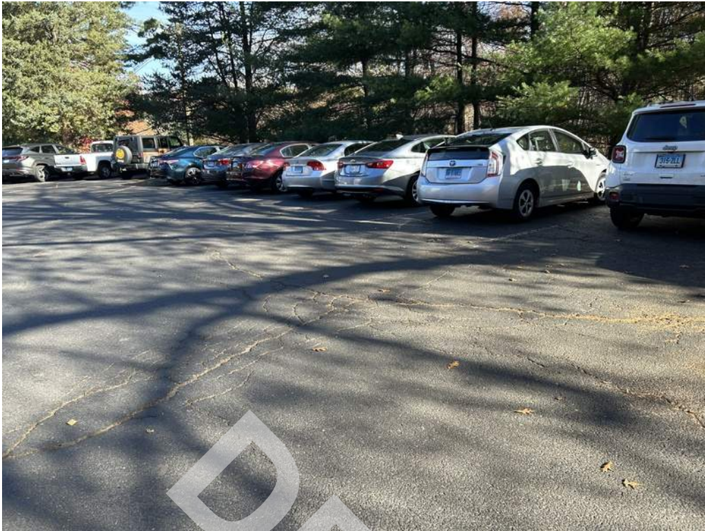
3 - The asphalt paved parking provided at the side of the building exhibits alligator and longitudinal cracking.
