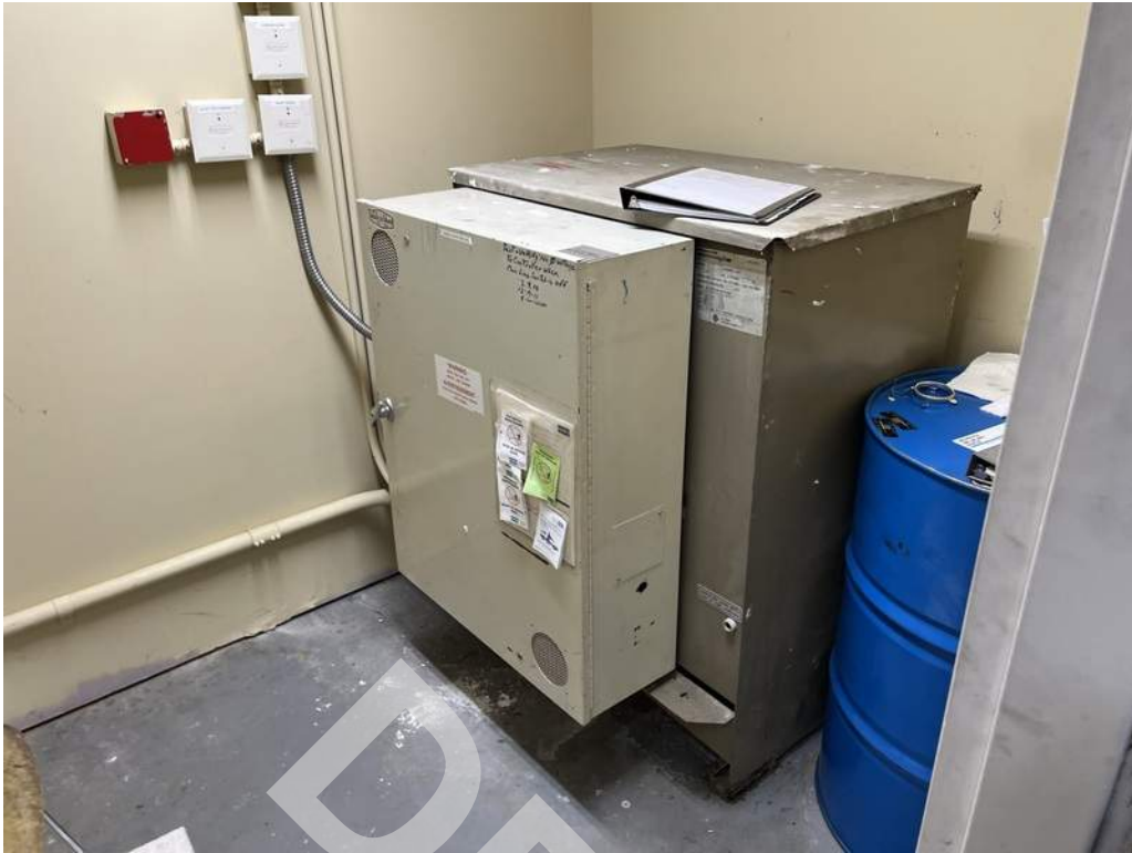
31 - Elevator equipment is located in the elevator equipment room on the lower level.
