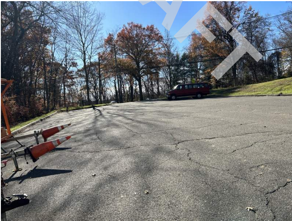
4 - One of the two additional parking lots exhibit cracking and damaged curbing.
