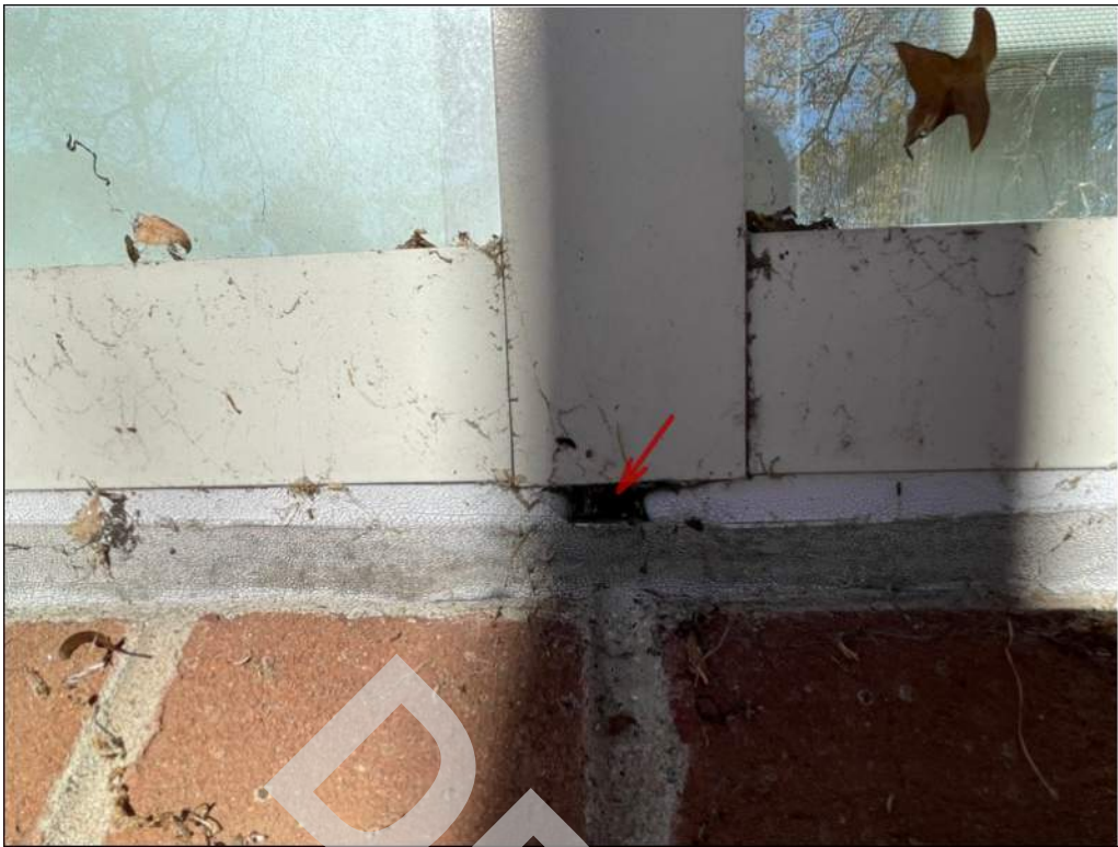
17 - Perimeter joint sealant along windows is in poor condition. Deficiencies include ruptured and crazed sealant.
