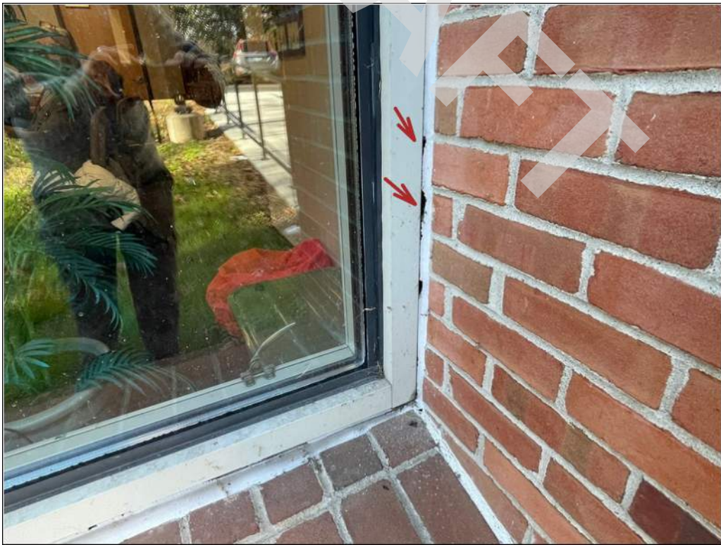
16 - Most perimeter joint sealant around windows has failed.
