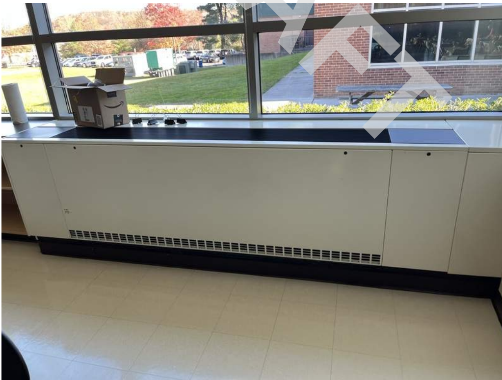
22 - Unit ventilators provide heating and cooling to individual classrooms.
