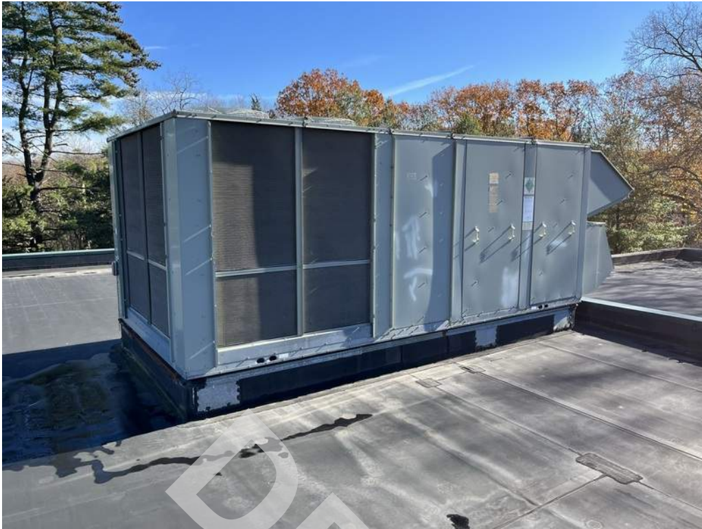
25 - Two rooftop packaged units (RTU) provide heating and cooling to portions of the building. One RTU is natural gas fired and the other is provided with a hot water coil that is fed from the boilers.
