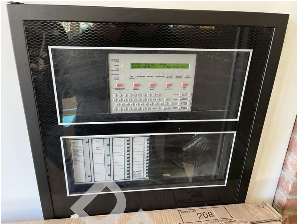
29 - The building is provided with a fire alarm panel which is located in the vestibule of the main entrance.
