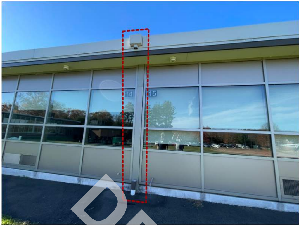
11 - The roof leader is missing.
