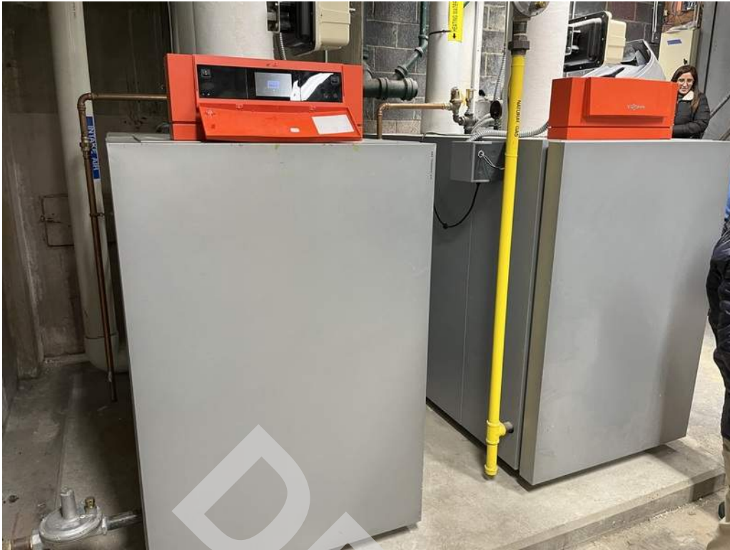
21 - Two natural gas fired boilers located in the lower level provide heating hot water throughout the building.
