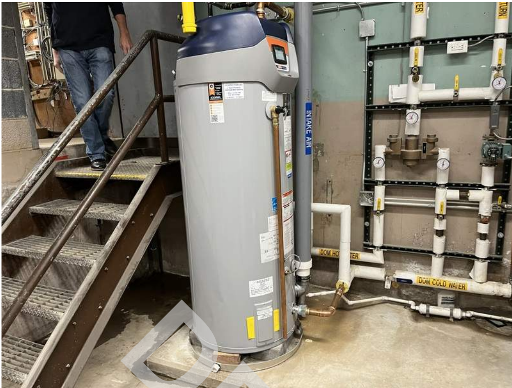
27 - A natural gas fired storage-type water heater is located in the lower level and provides hot water throughout the building.
