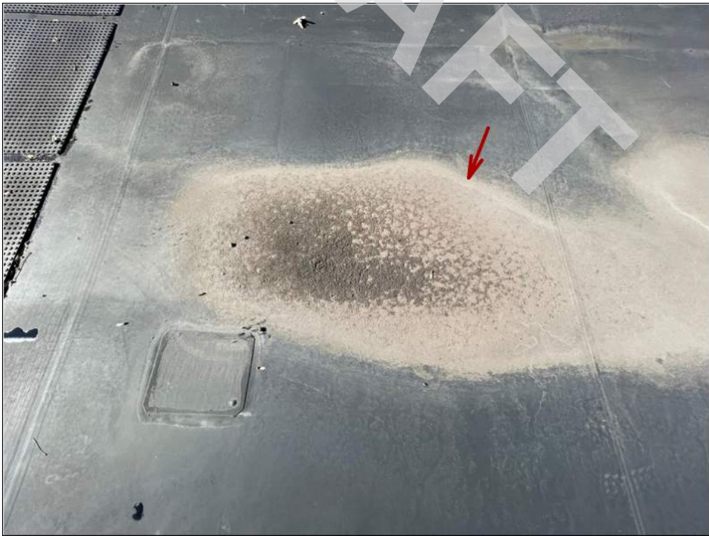
10 - Debris accumulation in a soft spot area of the roof.
