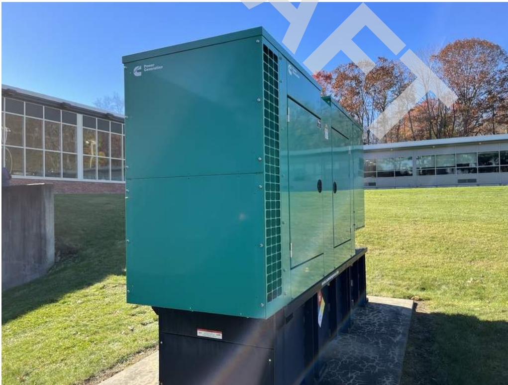
28 - A diesel-fired emergency generator located on the exterior of the building provides emergency power to the building.
