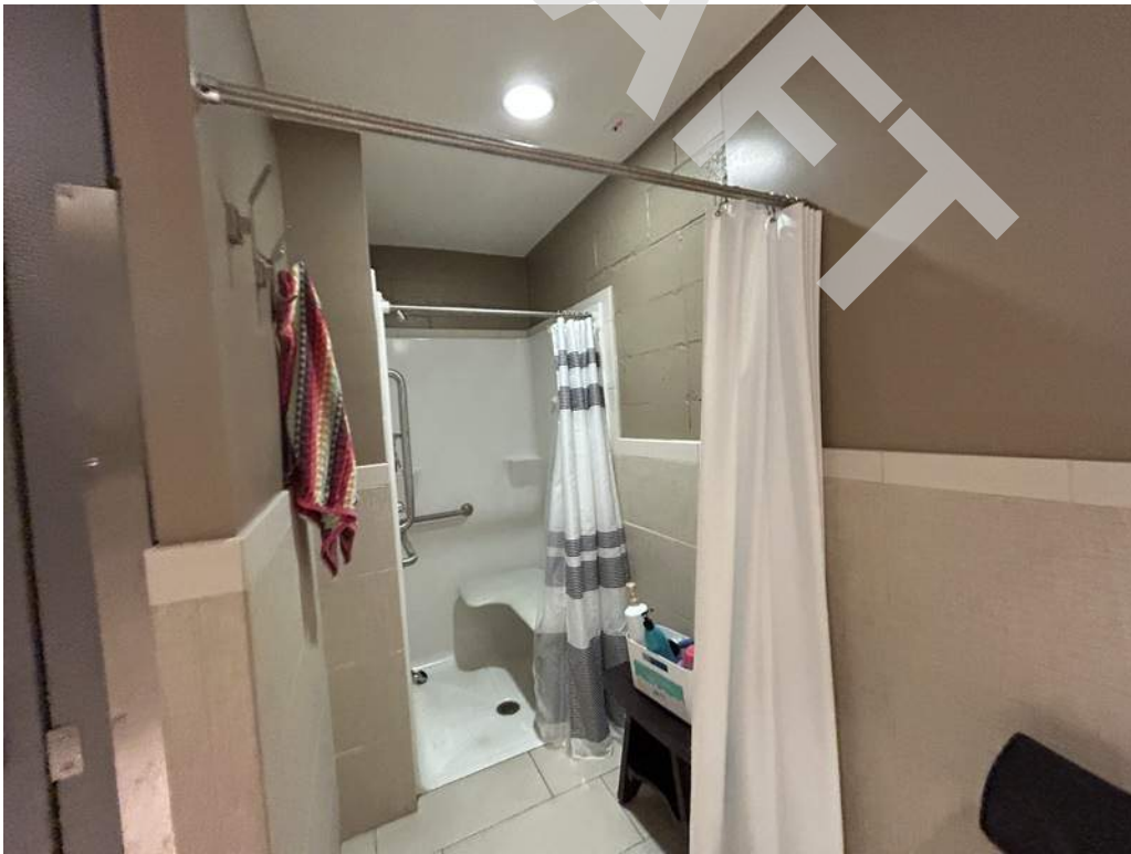
38 - The minimum required clearance measured from the transfer shower control wall is not provided.
