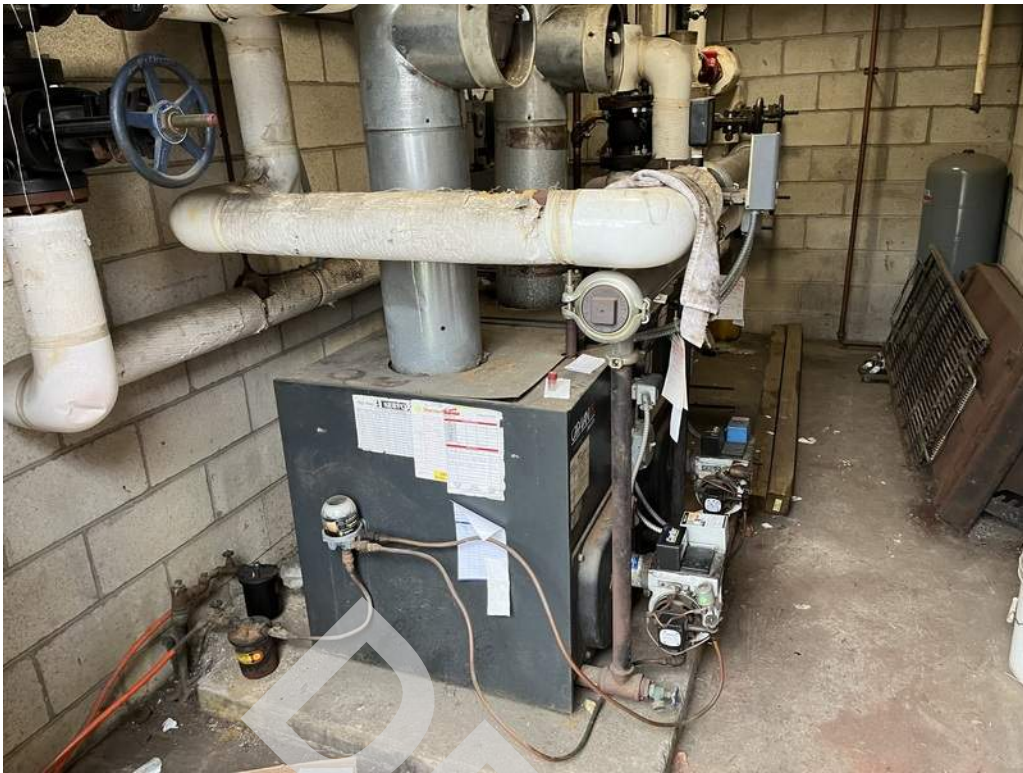
21 - Two oil fired boilers provide heating hot water throughout the building.
