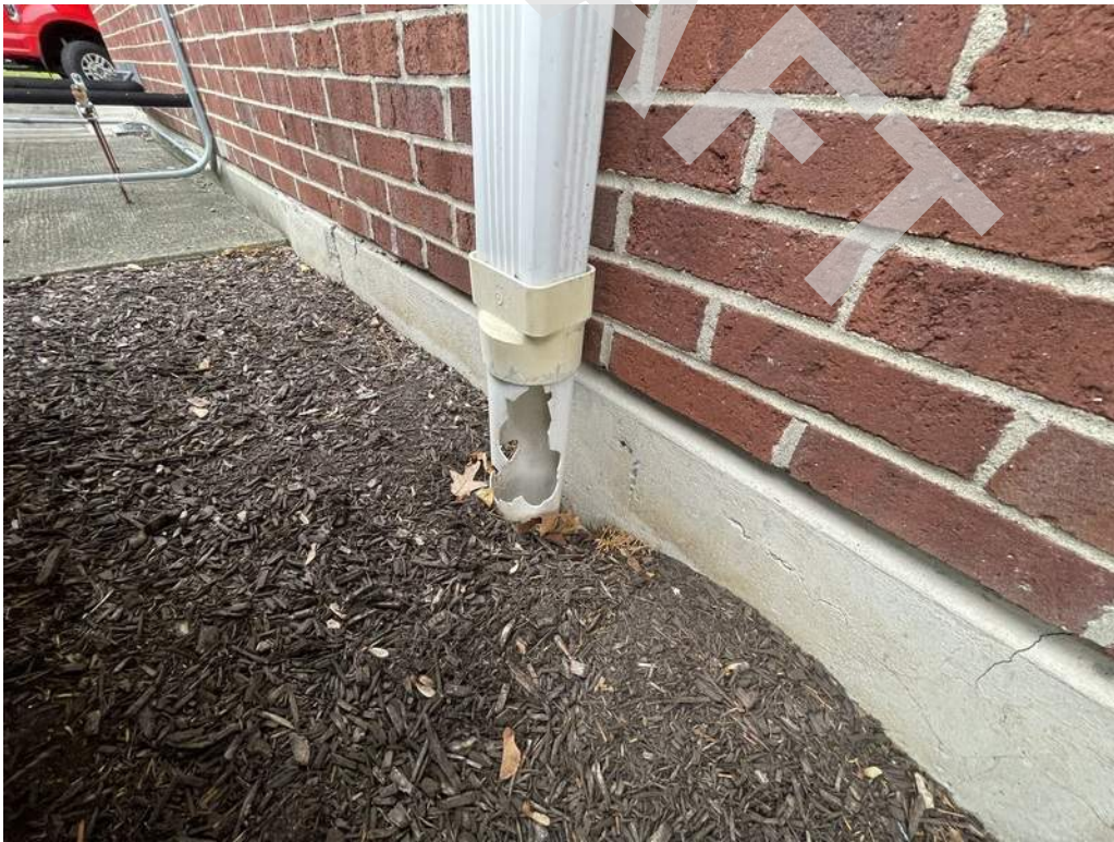
10 - Instances of the roof leader connection to the building's stormwater system are broken.
