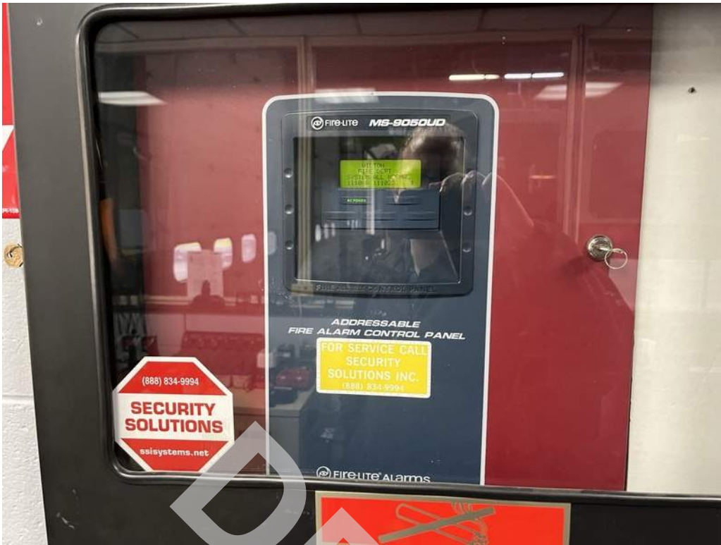
25 - The building is provided with a MS-9050UD Fire Alarm Panel.
