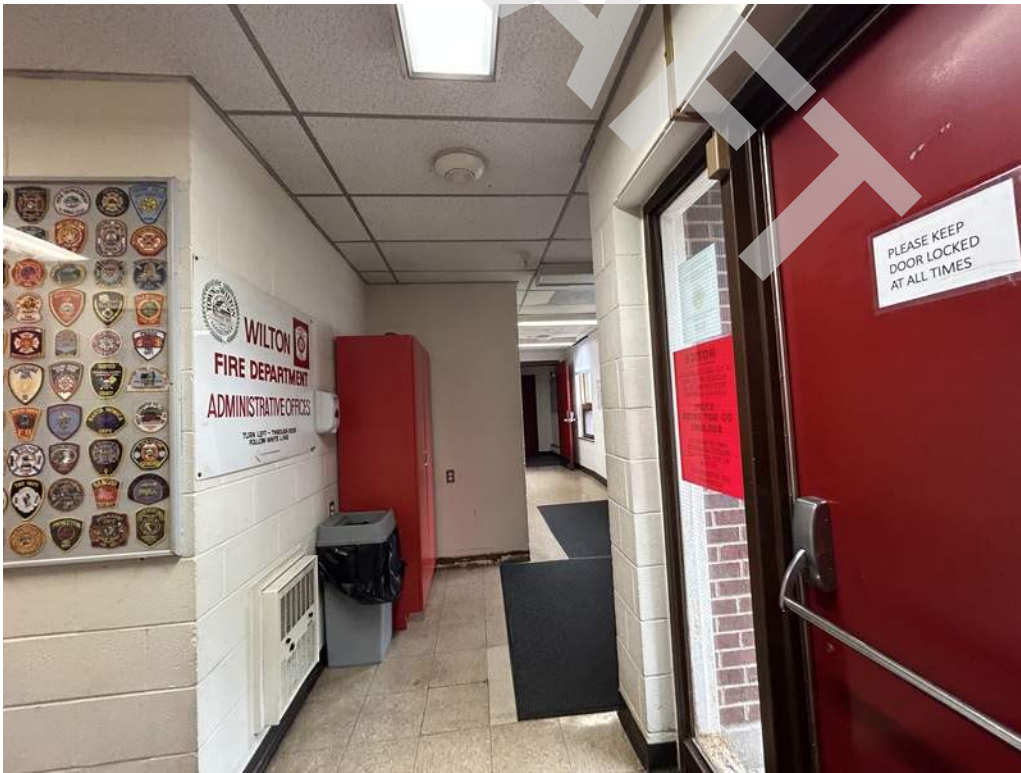
18 - Interior corridor finishes generally consist of painted gypsum walls boards or masonry, suspended ceilings with acoustic tiles, and vinyl composite tile floors. Chipped floor tiles and missing baseboards were observed.
