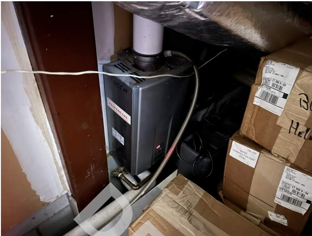
23 - A propane fired tankless water heater is located on the second floor and provides hot water throughout the building.
