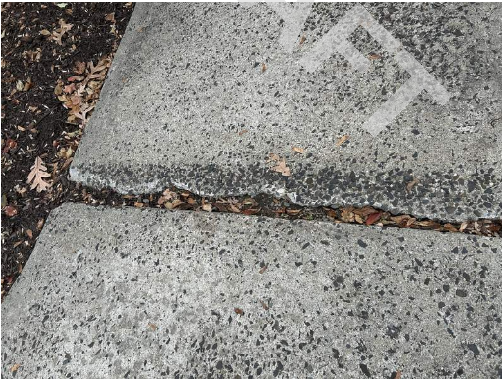
2 - Spalled concrete was observed at localized areas at sidewalks.
