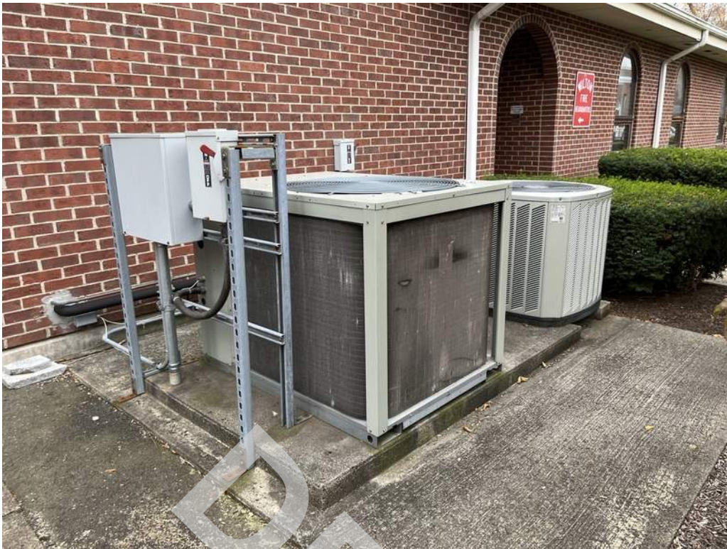
19 - Split system air conditioning units are located on the exterior of the building and provide cooling throughout the building.
