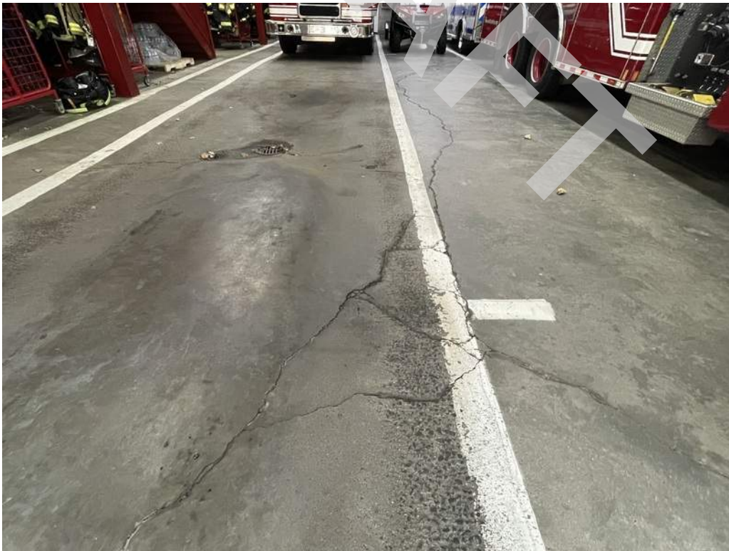
4 - The apparatus room slab on grade is uneven, has spalled, and has continuous cracks.
