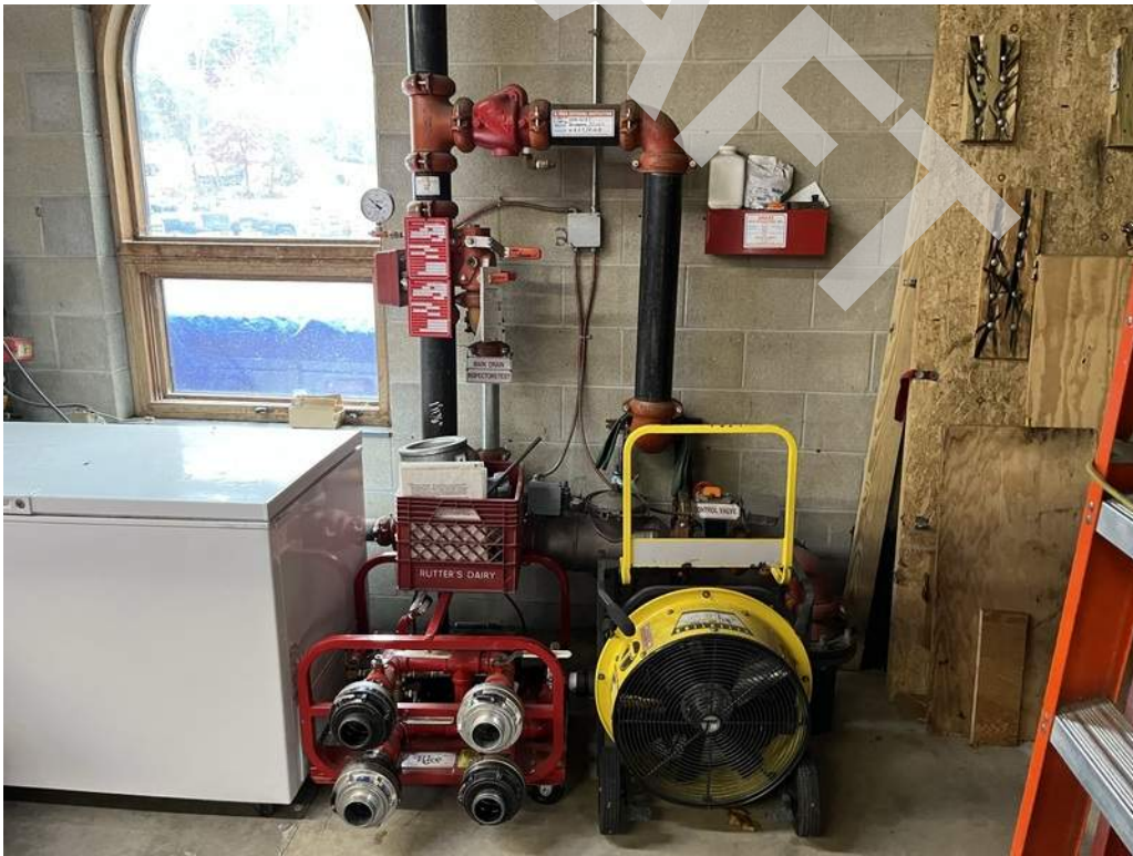
26 - The building is equipped with a wet sprinkler system.
