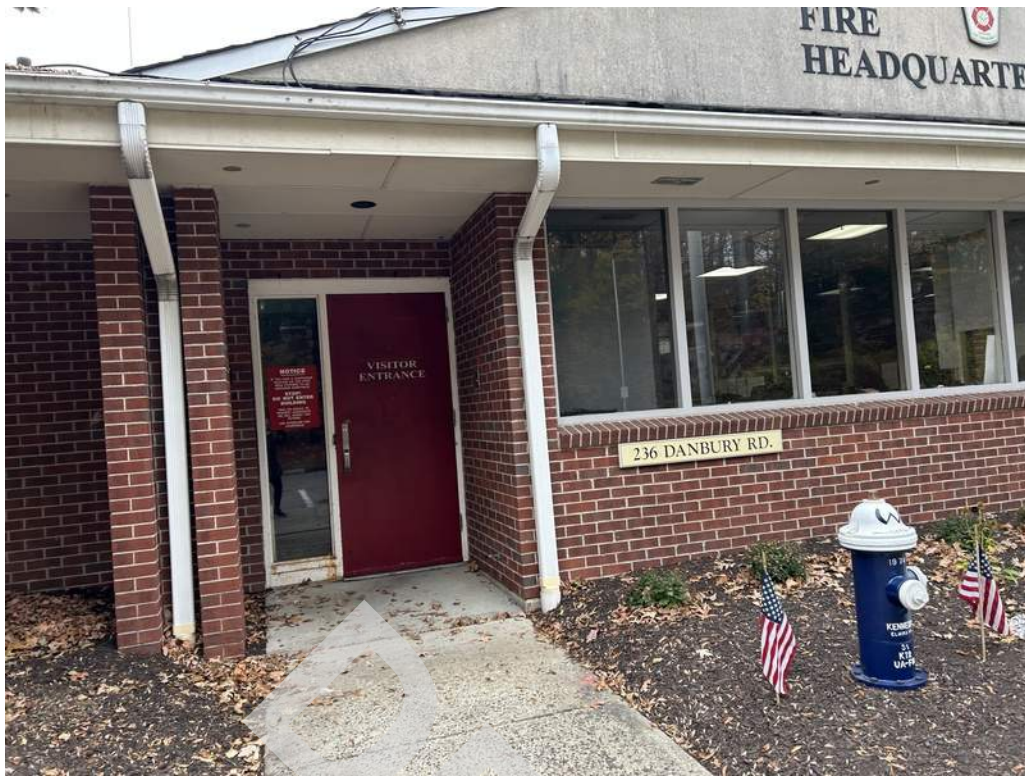
27 - The visitor entrance provided at the rear side of the building is non compliant as the threshold exceeds the allowable height.
