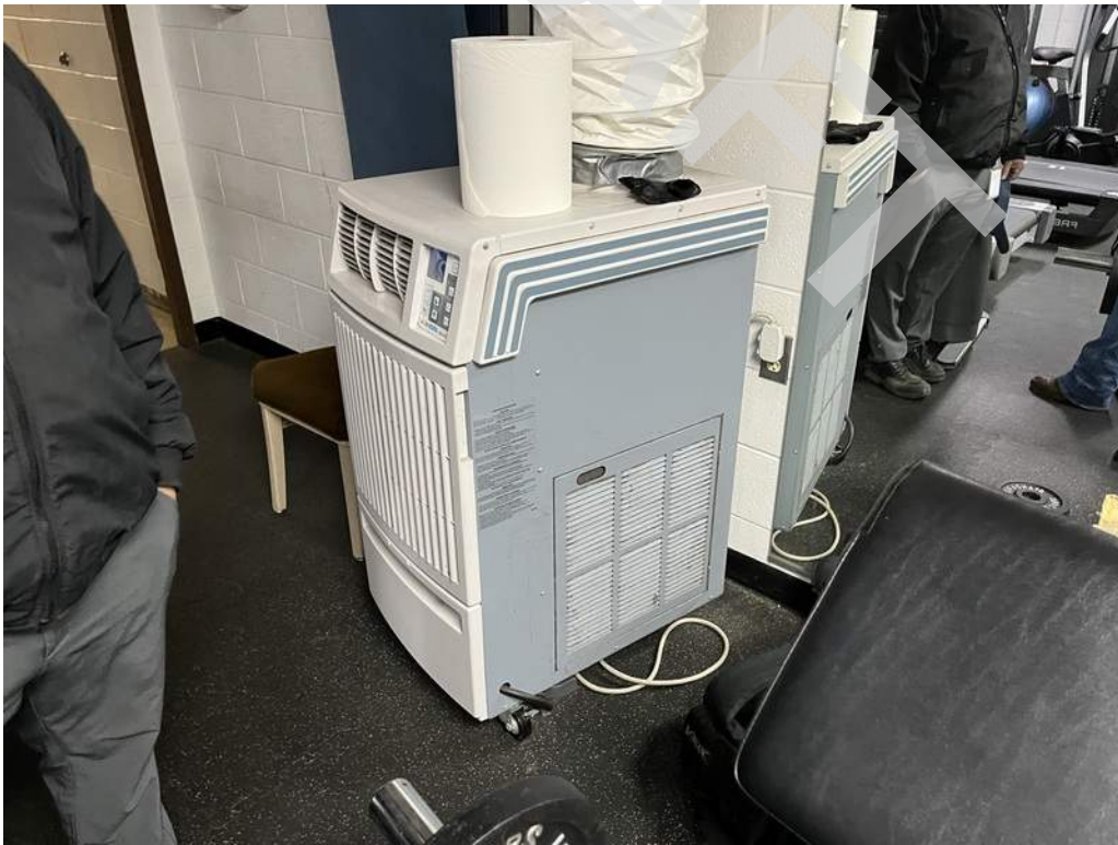
20 - A portable air conditioning unit is utilized for supplemental cooling in the gym.
