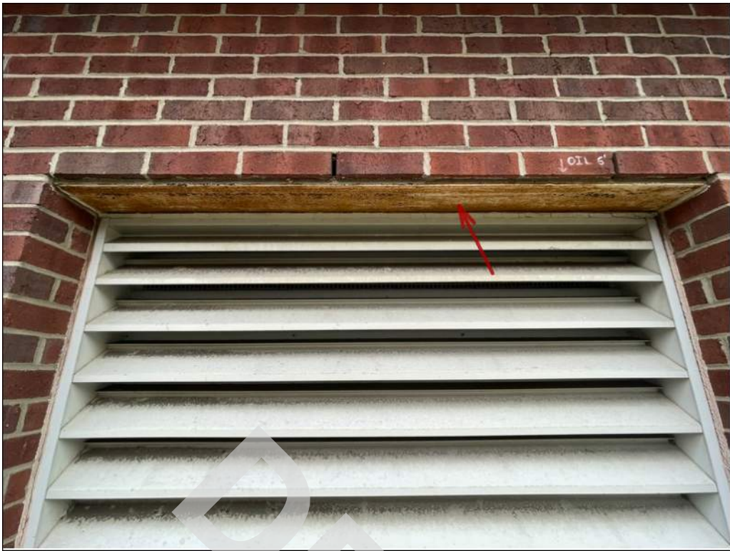
13 - Metal surface of the lintel at the louver opening has corroded.
