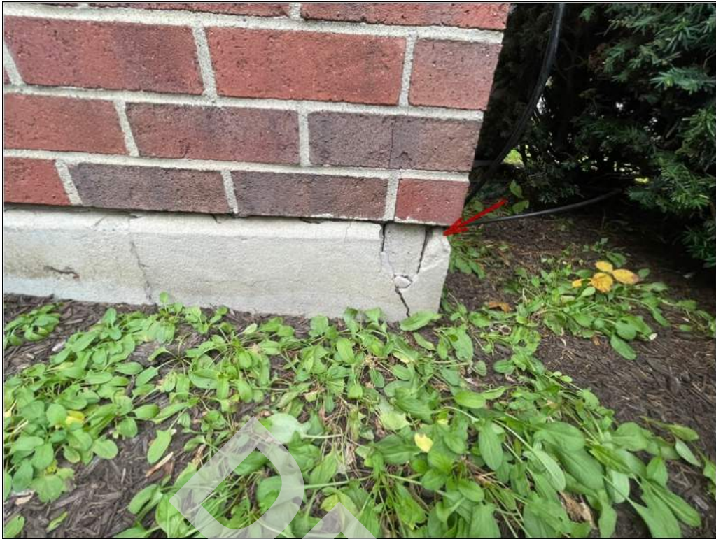
3 - Areas along of the cast-in-place reinforced concrete foundations walls have spalled and appear to have been previously repaired.
