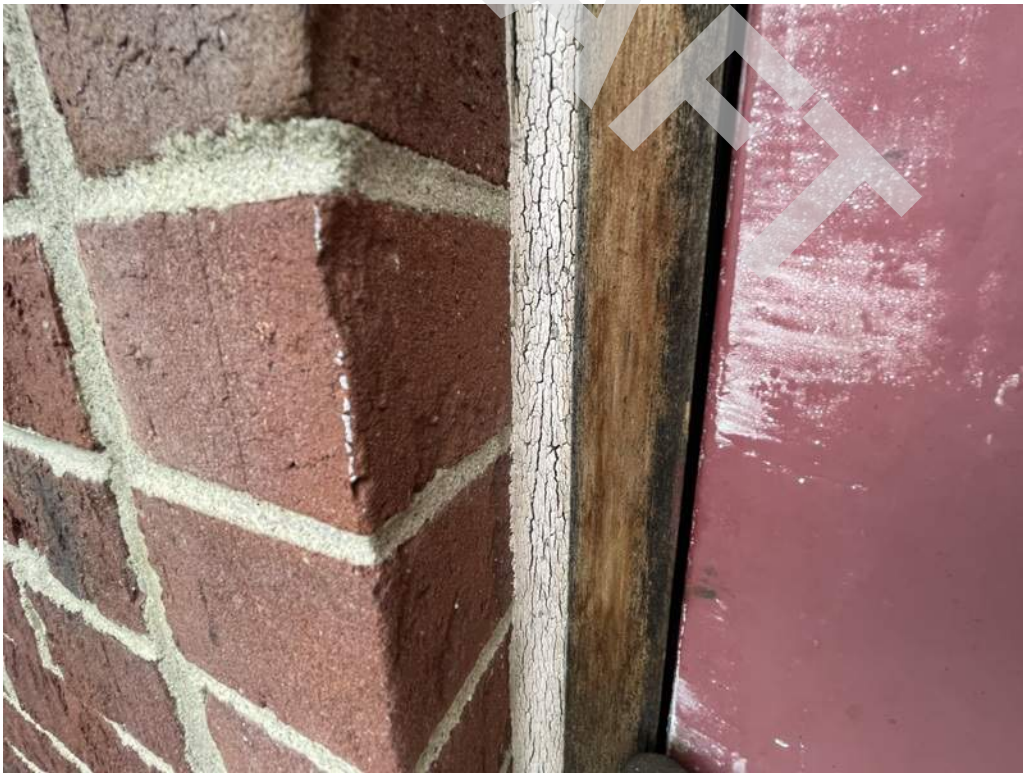
12 - Perimeter joint sealant has failed.
