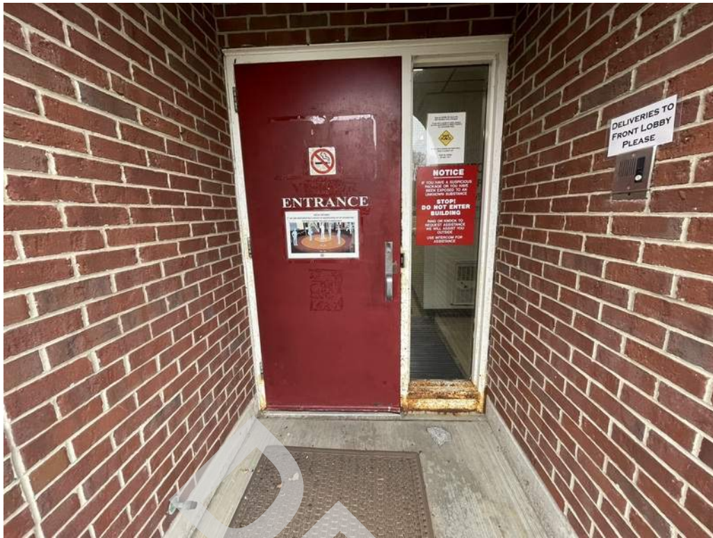
15 - Side light framing has corroded along the bottom. Hollow metal door surfaces are in fair condition.
