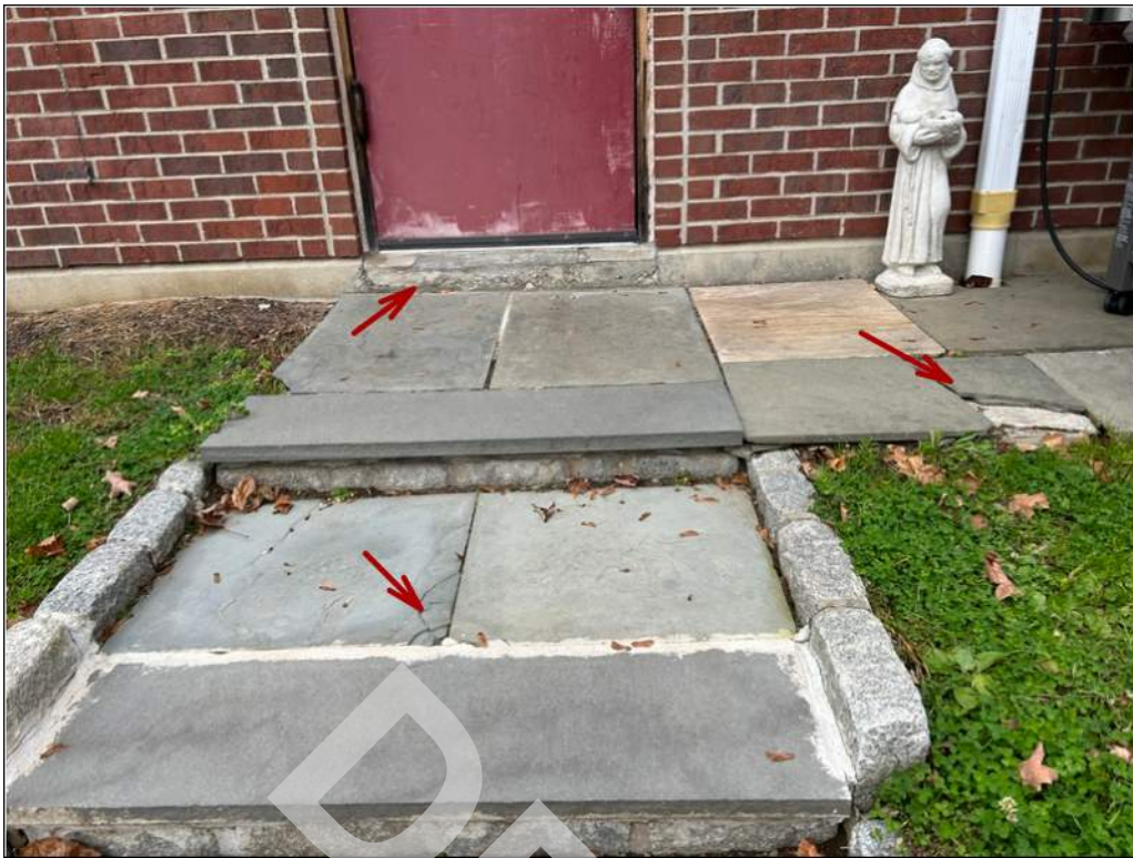
17 - Stone pavers have cracked and are missing pieces.
