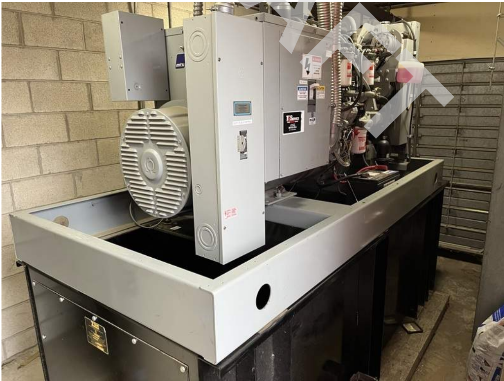
24 - A diesel-fired emergency generator located in a generator room in the Fire Headquarters provides emergency power to the Fire Headquarters and Garage buildings.
