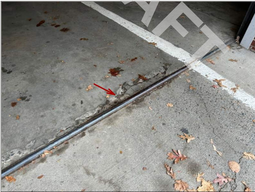
6 - Spalling along the base of an overhead door.
