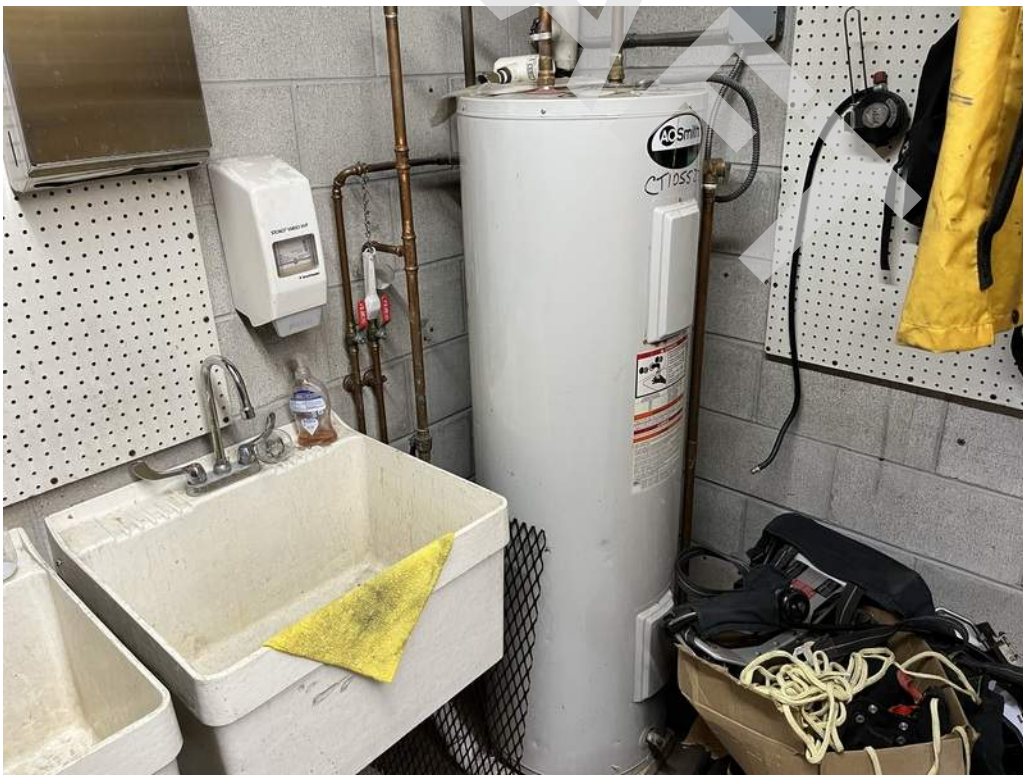
22 - An electric storage-type water heater located on the first floor provides hot water throughout the building.
