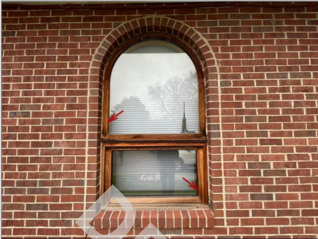
11 - Wood framing surfaces at the operable and fixed windows throughout the building have worn out and are in fair condition.
