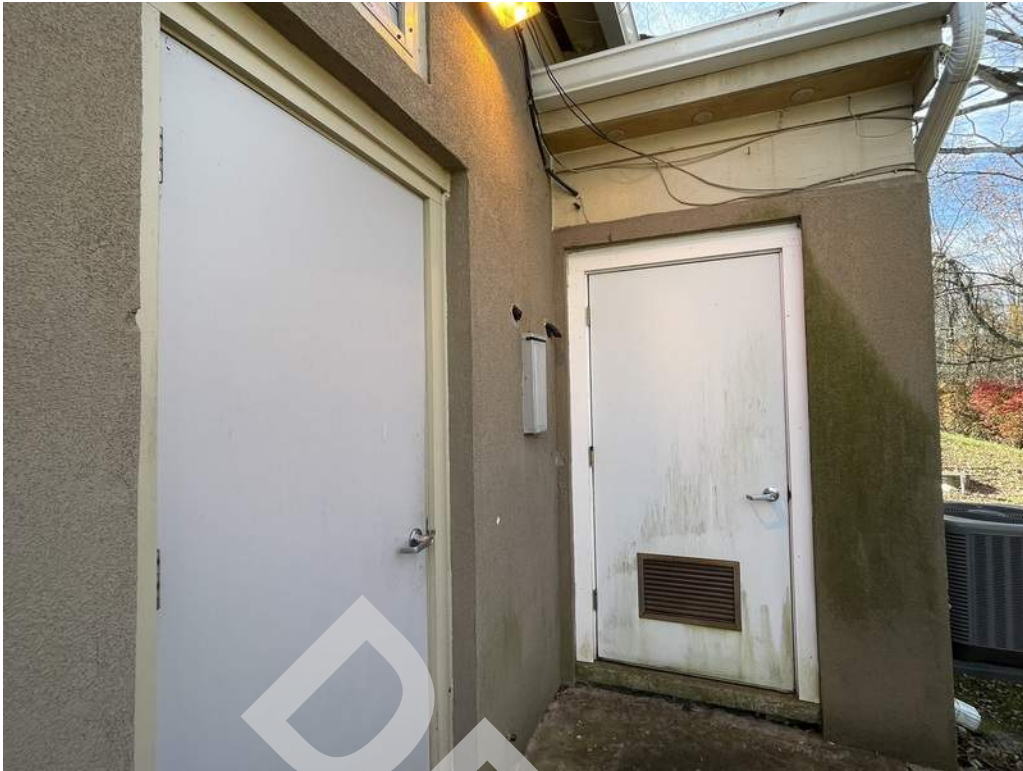
9 - Areas of the EIFS and doors have organic growth.
