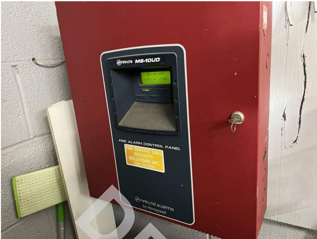
19 - The building is provided with a Fire-Lite MS-10UD fire alarm panel.
