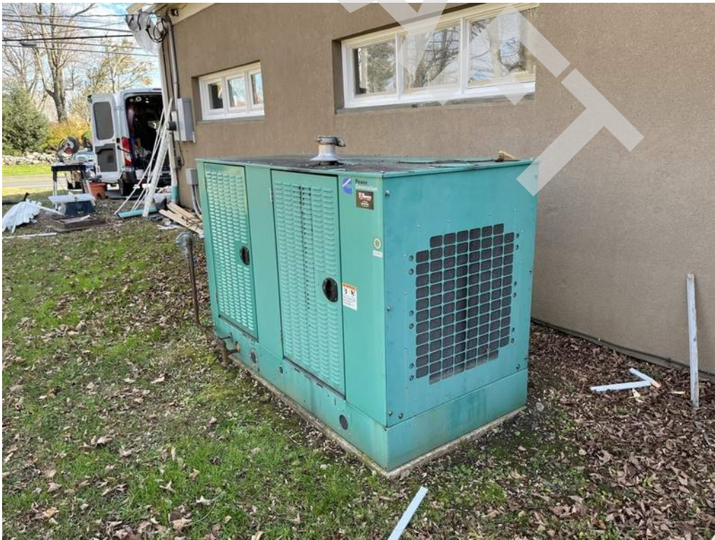
18 - A propane-fired emergency generator provides emergency power to the building.
