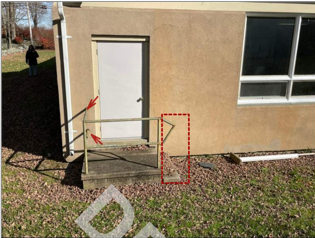
11 - Metal pipe handrail along the steps located at the west façade has corroded and does not extend beyond the last tread.
