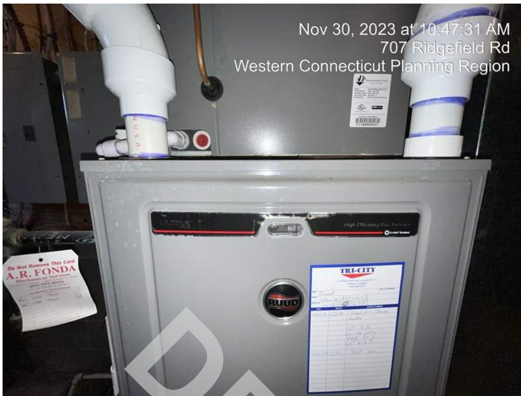
15 - Two propane fired furnaces located in the mechanical room provide heating to the building.
