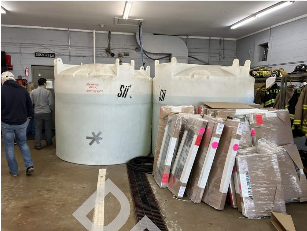
17 - Two water storage tanks located in the garage currently provide the building with domestic water.
