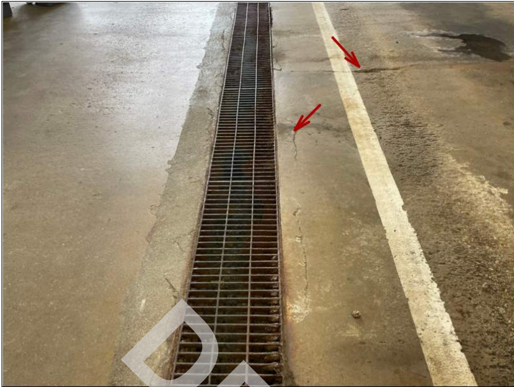
5 - Areas of the slab on the southern apparatus bay have cracked.
