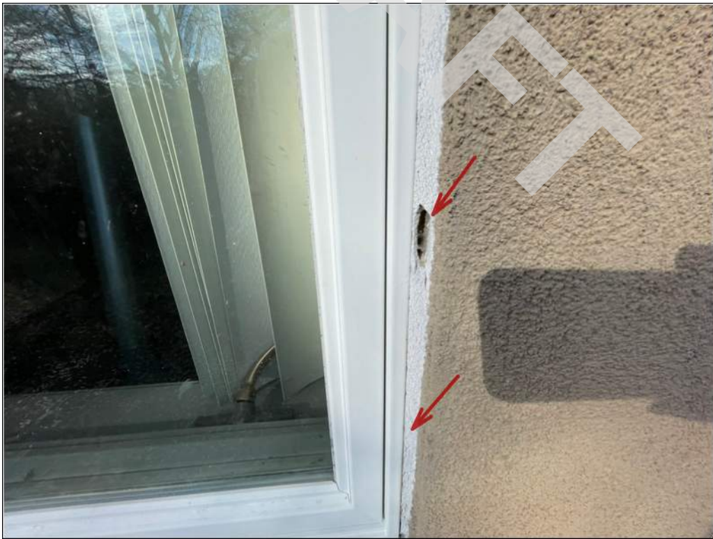
10 - Window perimeter joint sealant has failed. Surface is crazed and ruptured.
