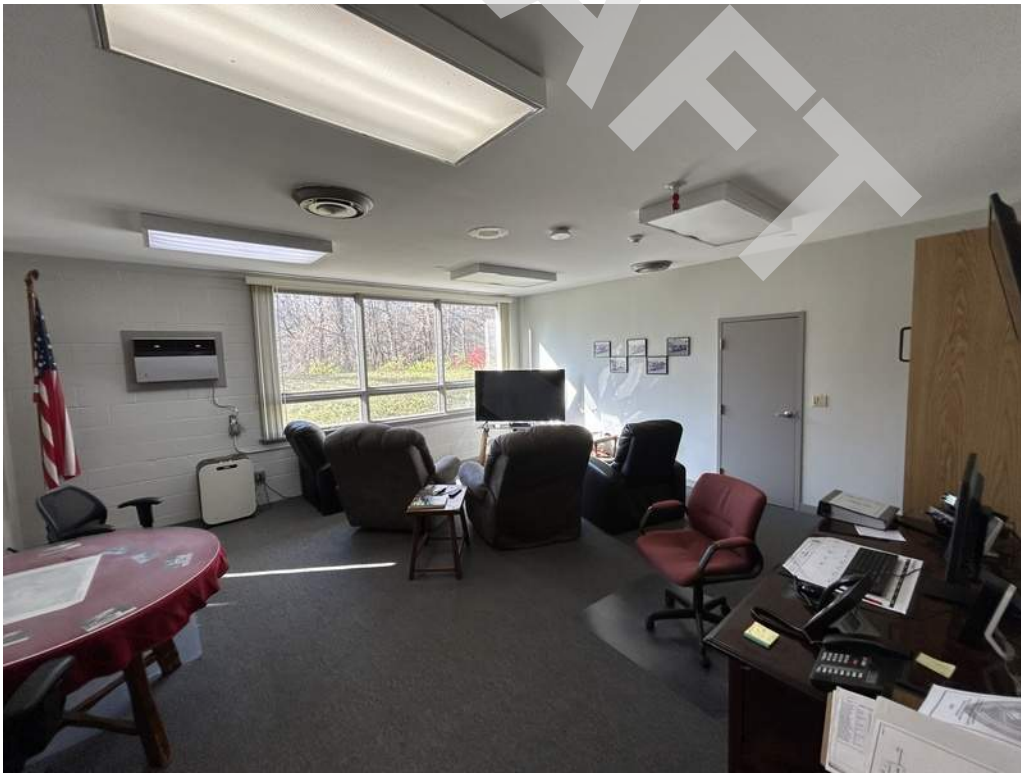
12 - Interior common space finishes consist of painted gypsum ceiling and wall boards and carpet floors. Exit signage directing occupants to the egress door along the west side of the building is not provided.
