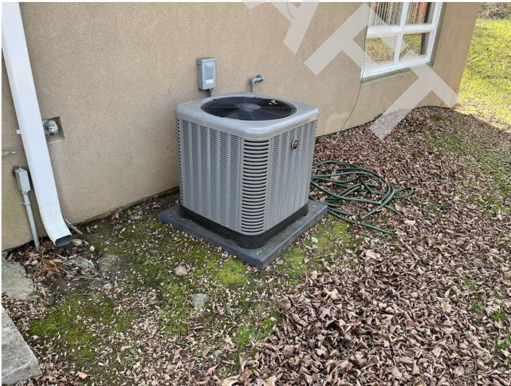
14 - A split system air conditioning unit located on the exterior of the building provides cooling.
