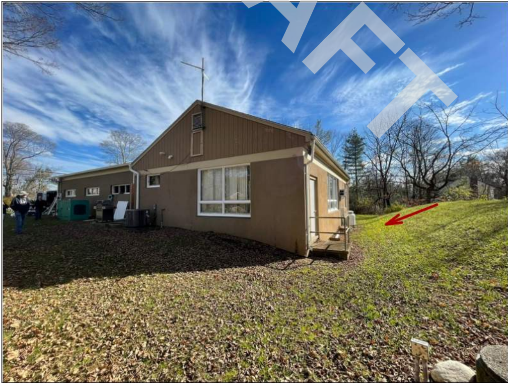
2 - Mound septic system is sloping towards the building's structure.
