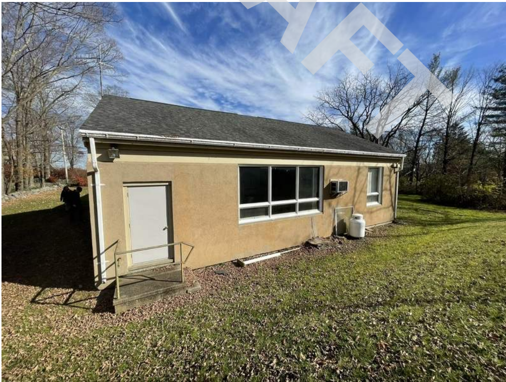
6 - Exterior walls consist of painted EIFS (exterior insulation finishing system). Windows consist of wood framed assemblies and the roof is covered with asphalt shingles.
