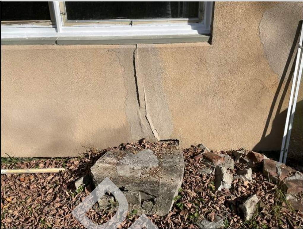
7 - Localized areas of the EIFS have cracked.
