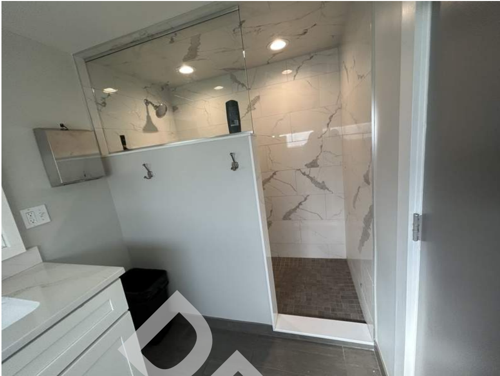
13 - Restrooms finishes consist of painted gypsum wall and ceilings boards and tile floors. The shower is fully tiled.
