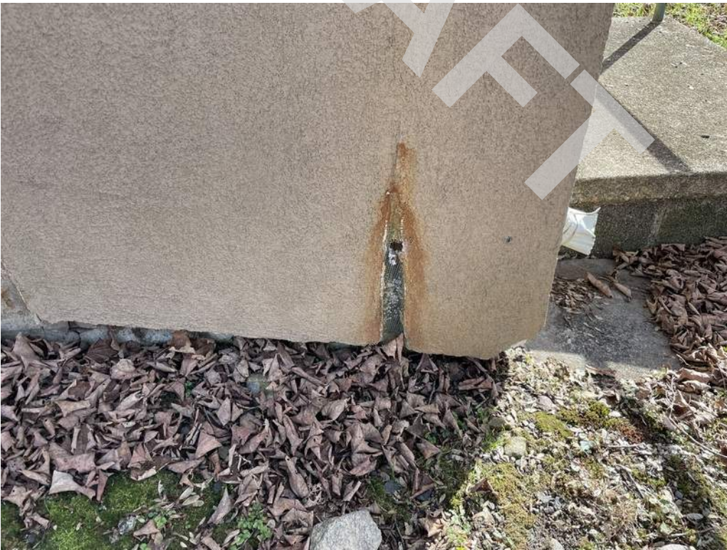
8 - Localized areas of the EIFS have eroded.
