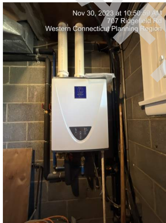
16 - A propane fired tankless water heater is located in the mechanical room and provides hot water throughout the building.
