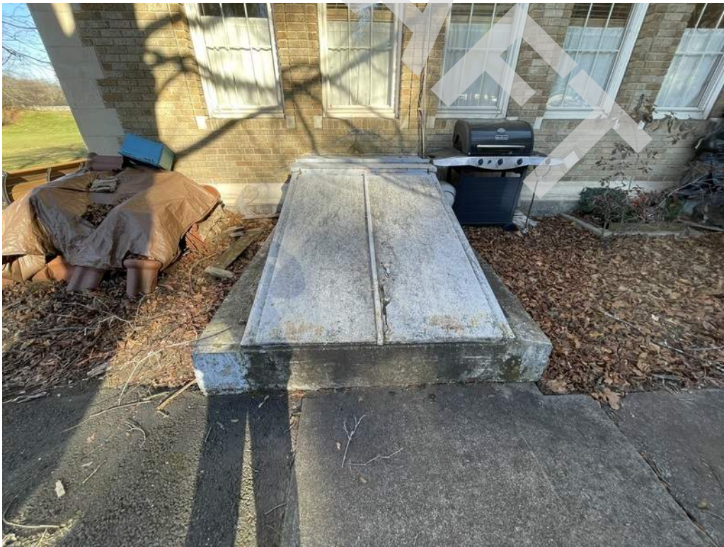
20 - Metal basement hatch door is in poor condition.
