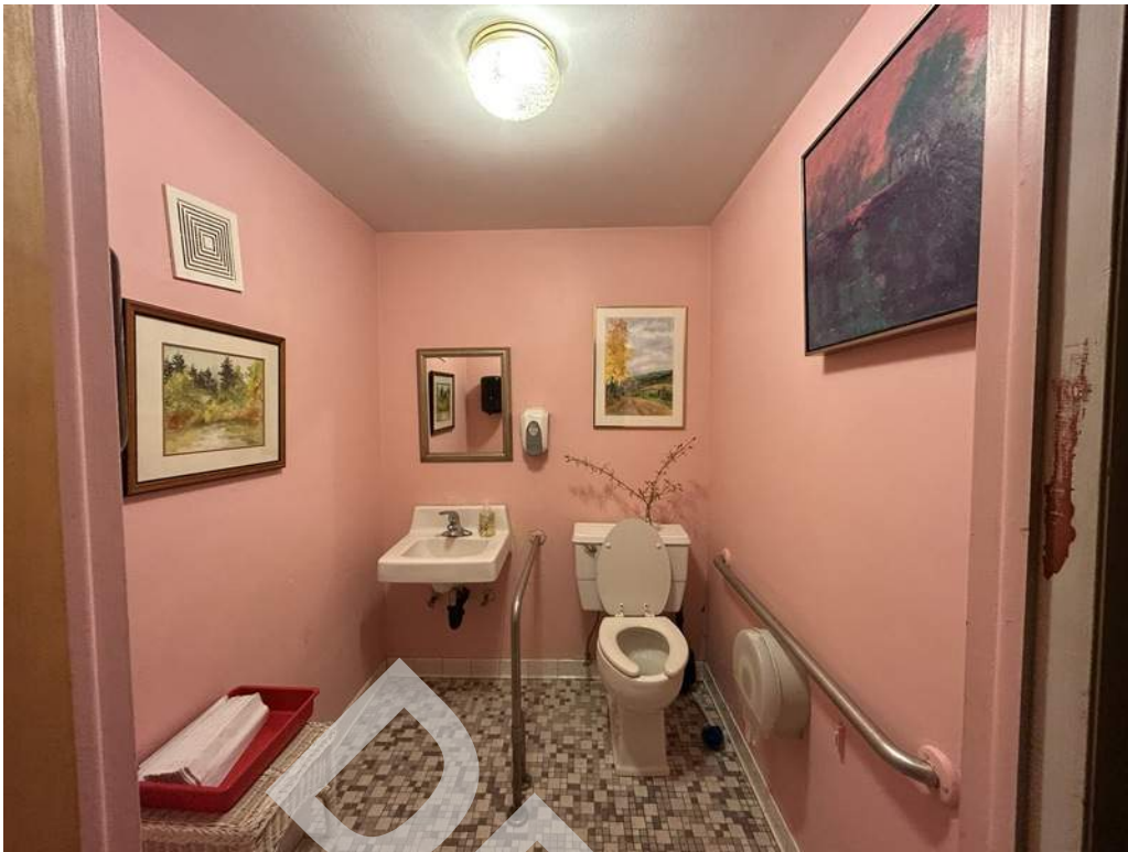
31 - The designated accessible single-user restroom is non compliant.
