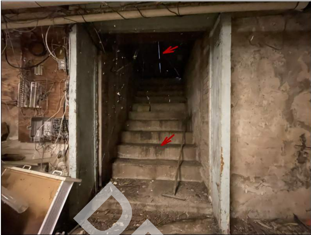
21 - Basement hatch door doesn't close properly and steps have signs of water intrusion.
