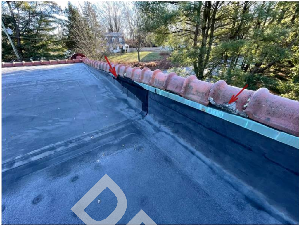
5 - Parapet coping consists of clay roof tiles with EPDM flashing and metal counterflashing. Clay roof tiles are in poor condition, some units are displaced and the EPDM parapet flashing is poorly installed.
