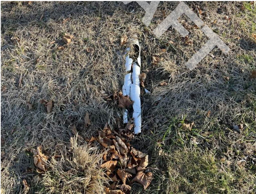
10 - Roof leader drain pipe extensions have failed.
