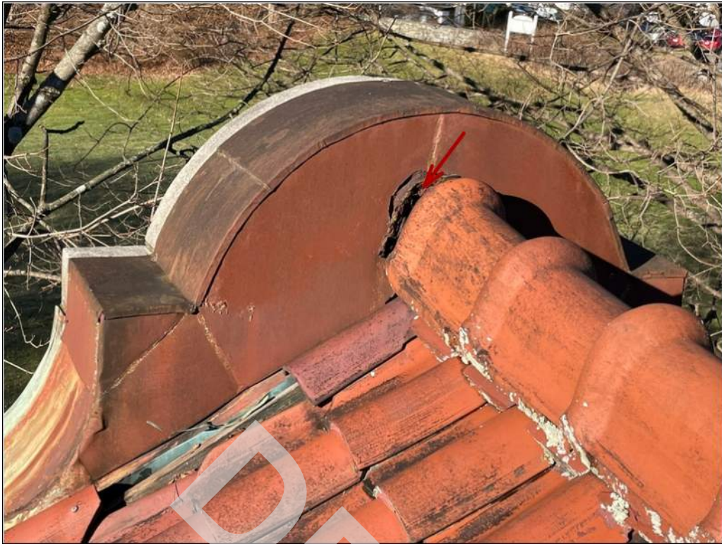
7 - Metal surfaces along the roof have corroded and have openings.
