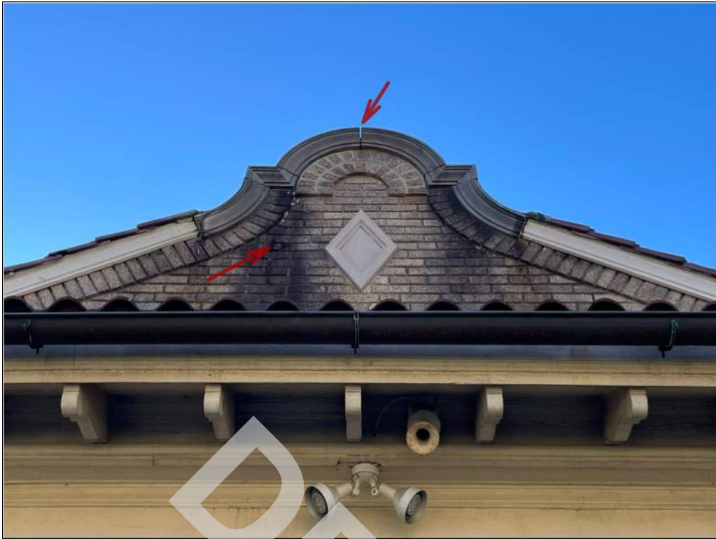
15 - Localized areas of mortar joints are missing or are in poor condition along the masonry brick and stone facades. Areas of the stone and brick masonry have organic growth and debris accumulation.
