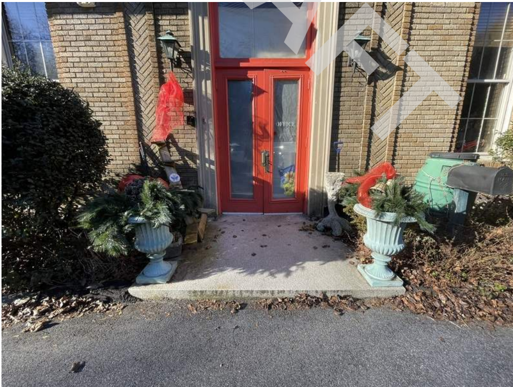
18 - Main entry door consists of a wood framed single pane glass assembly.
