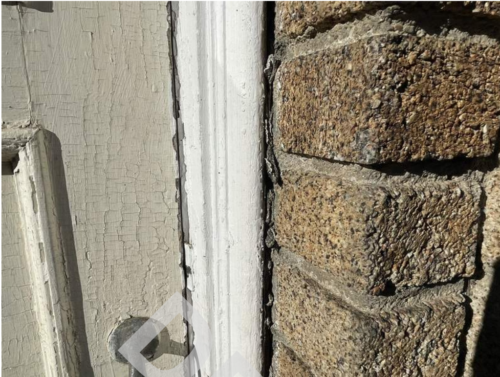
13 - Joint sealant along brick masonry openings has failed.
