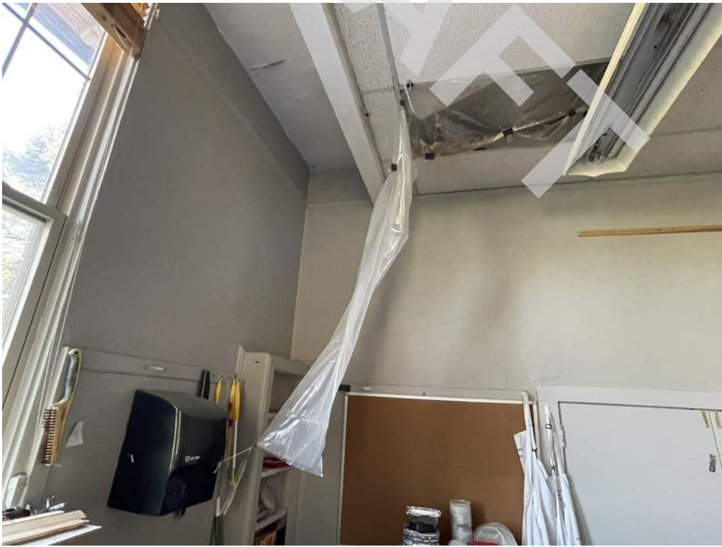
12 - Signs of active roof leaks coming down from the ceiling at one of the art studios.
