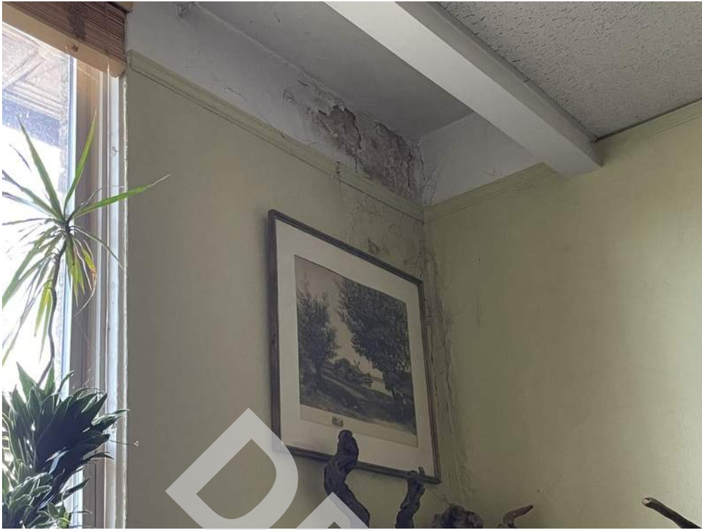
11 - Water intrusion through the roof has damaged the interior surfaces.
