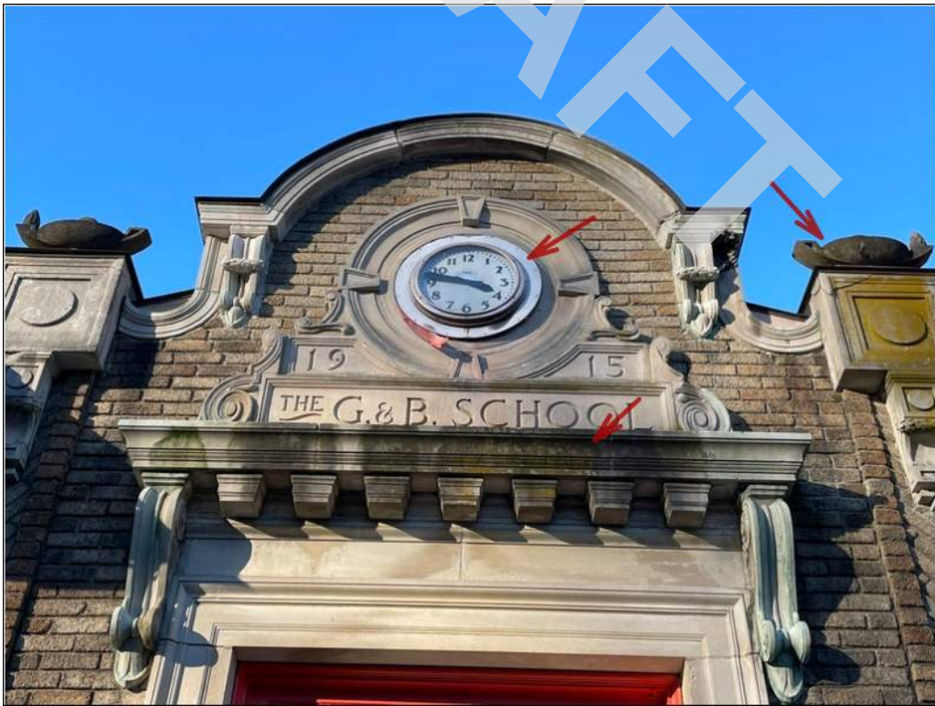
14 - Building clock is not working properly and appear to be in poor condition. Organic growth and build up stains are in the front facade stone.
