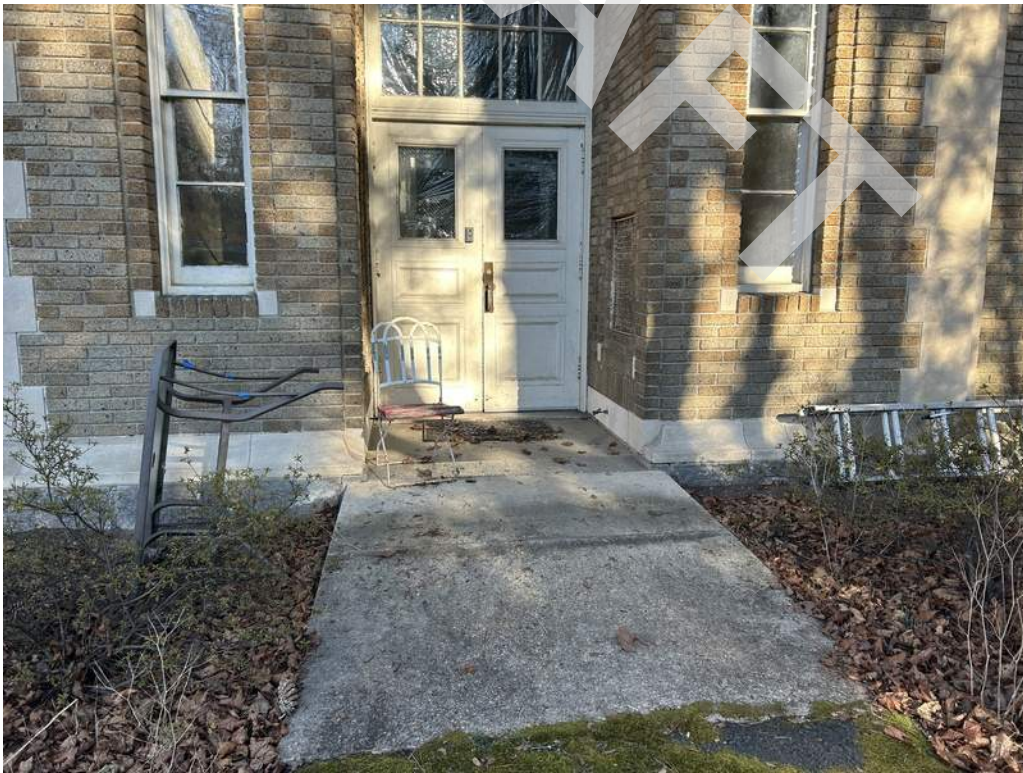
30 - The minimum clear width is not provided at the accessible entrance door.
