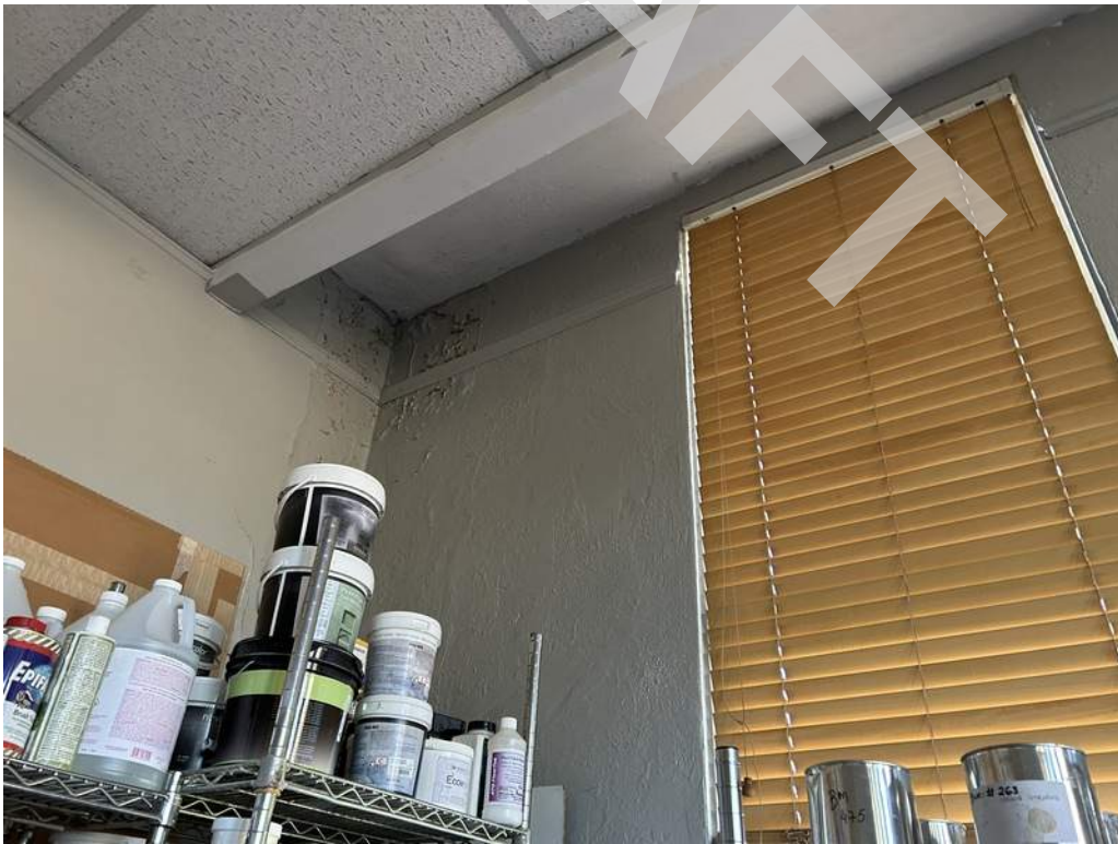
24 - Deteriorated paint was observed at the corner of Classroom 1AA.
