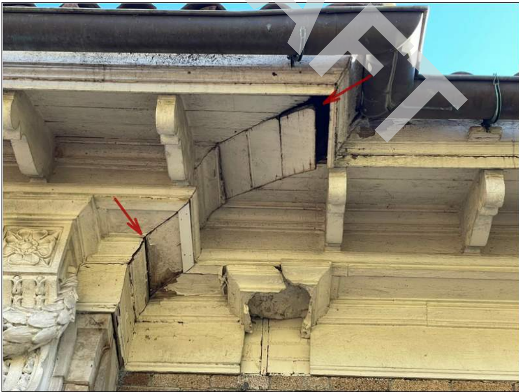
22 - Wood soffits and trim around the roof have displaced and open joints; paint finishes are peeling; wood surfaces are rotting and have missing pieces.
