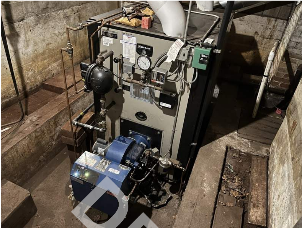
25 - An oil fired boiler located in the basement provides heating and domestic hot water throughout the building.
