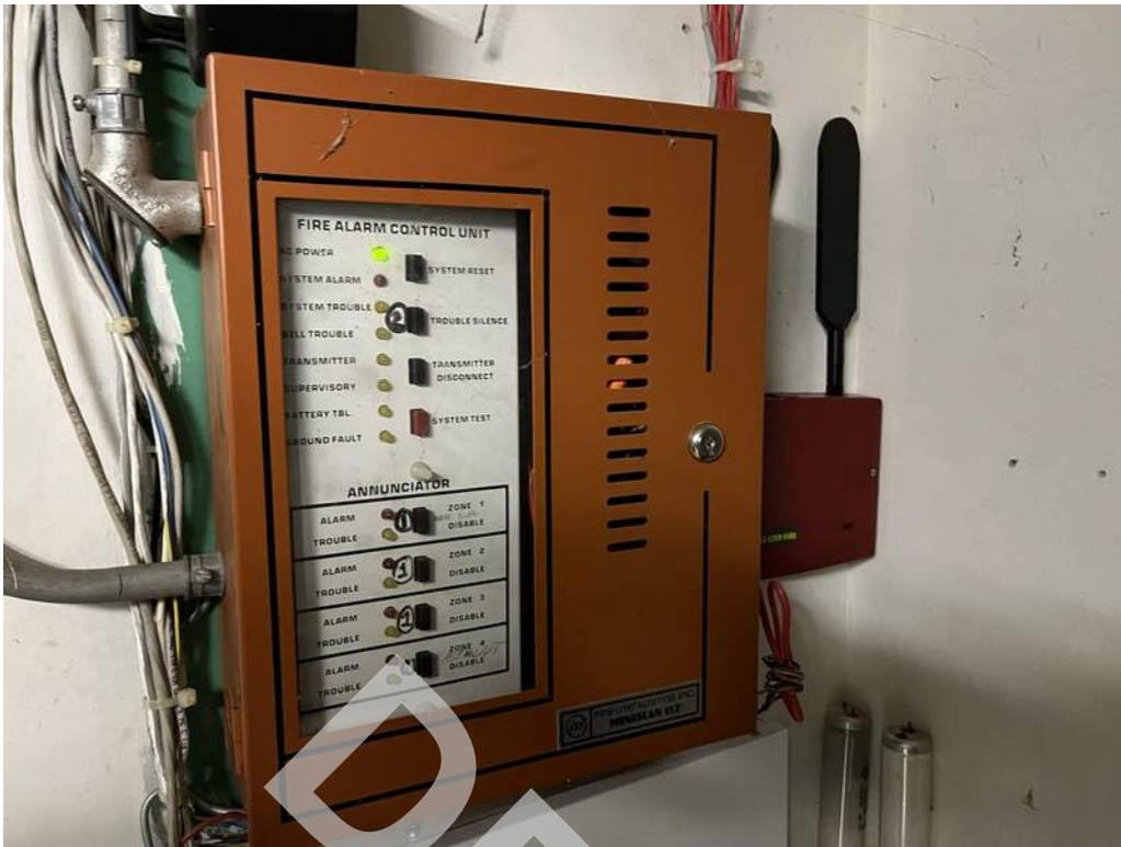
27 - The building is provided with a Miniscan 112 fire alarm panel.
