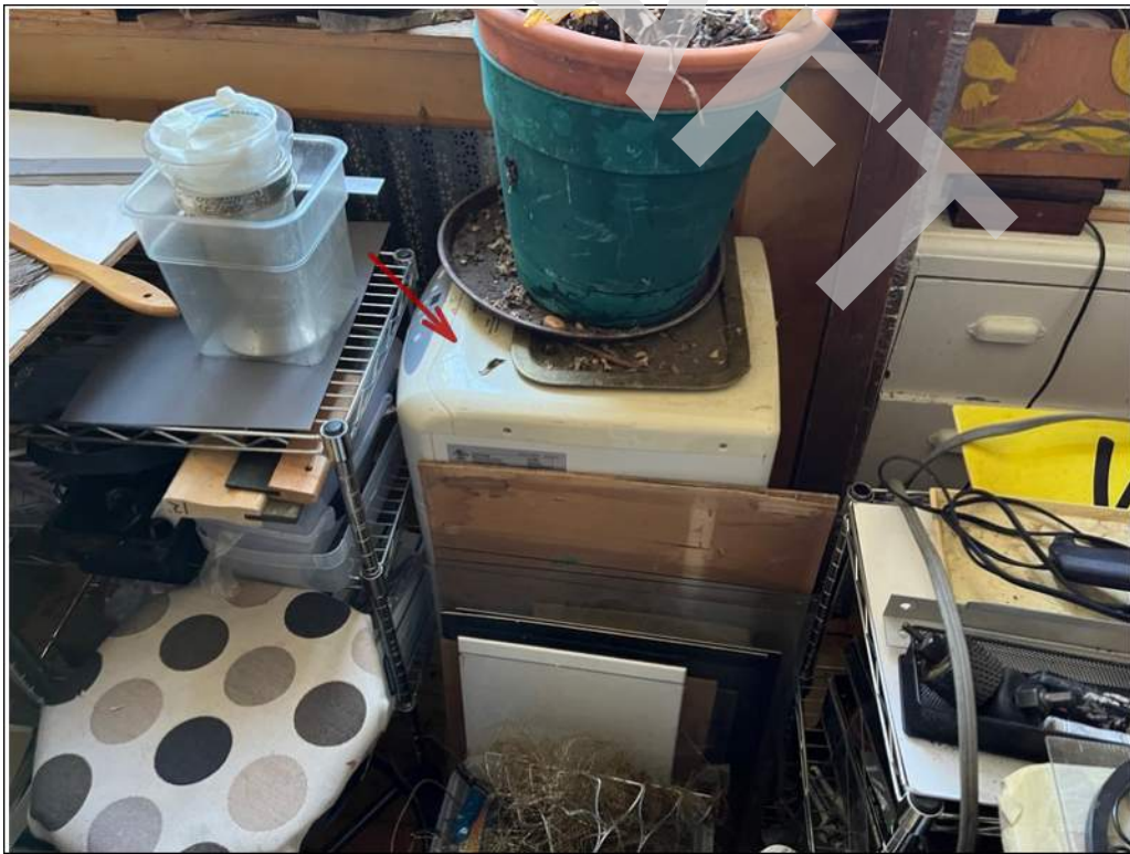
26 - Portable air conditioning units serving individual rooms provide cooling to portions of the building.
