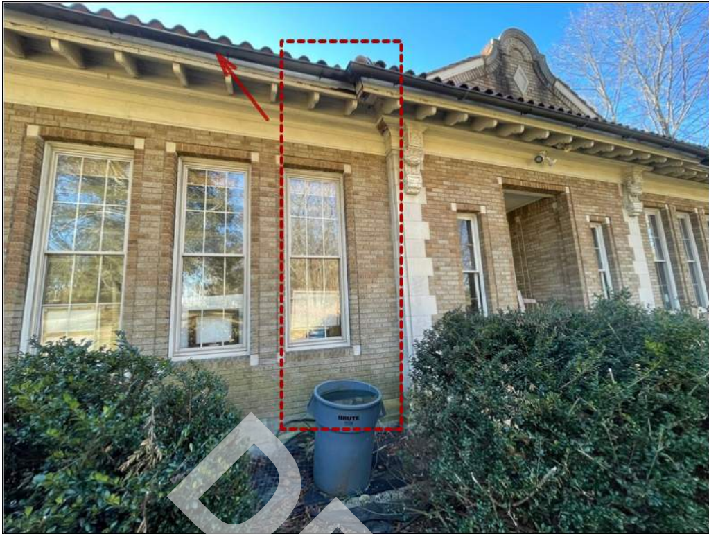
9 - Sections of the roof gutters are in poor condition and appear to be overflowing.
