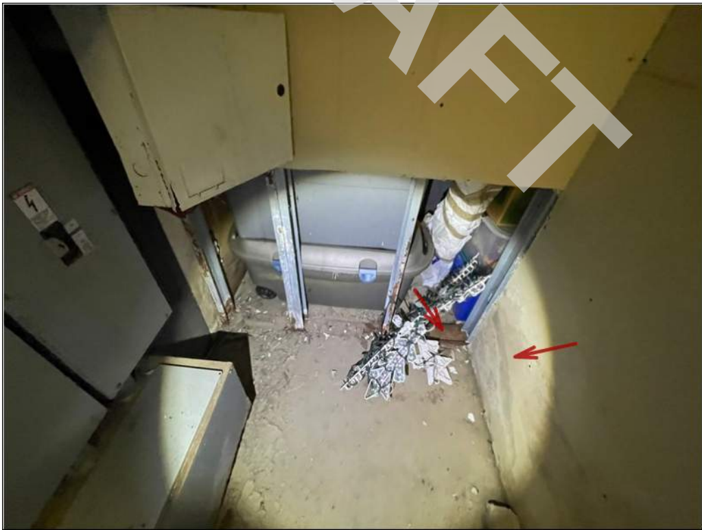
16 - Basement wall surfaces and wall framing metal components have water stains and corrosion due to water intrusion instances.
