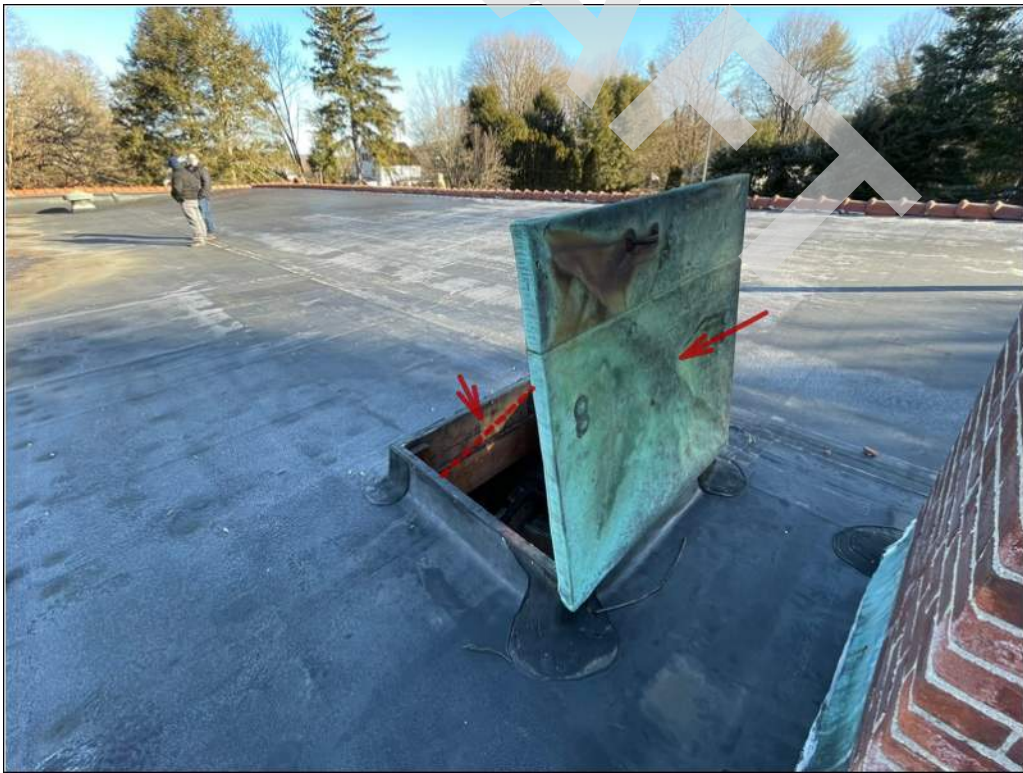
8 - Roof hatch is missing one hold open hardware and is in poor condition.
