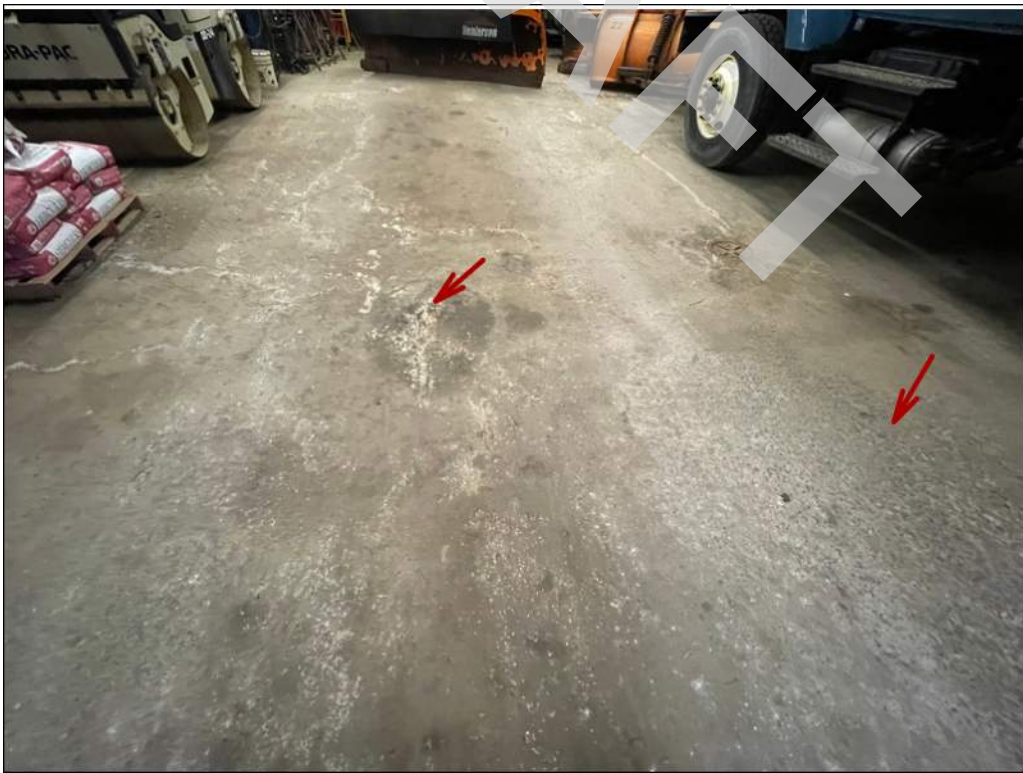
8 - Localized spalling and cracking has occurred along the concrete slab-on-grade.
