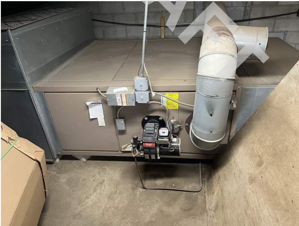
22 - Three oil fired furnaces located throughout the building provide heating throughout the building.
