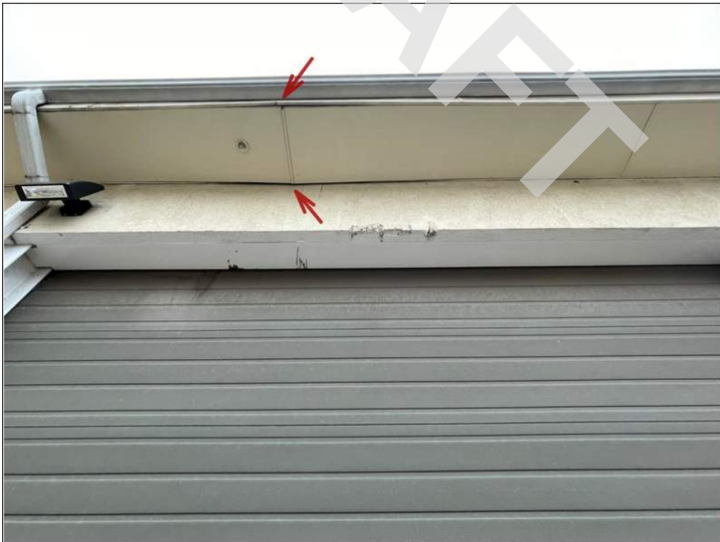
20 - Soffit and fascias are displacing.
