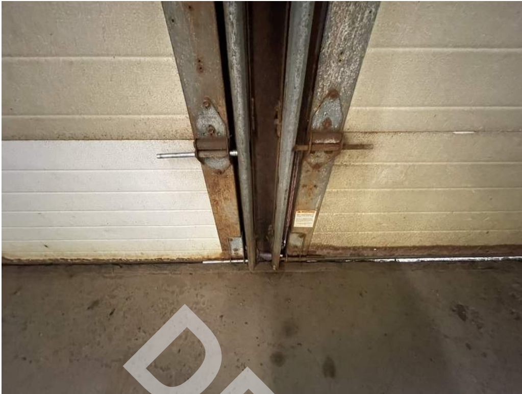
19 - Sectional overhead door metal components have corroded.
