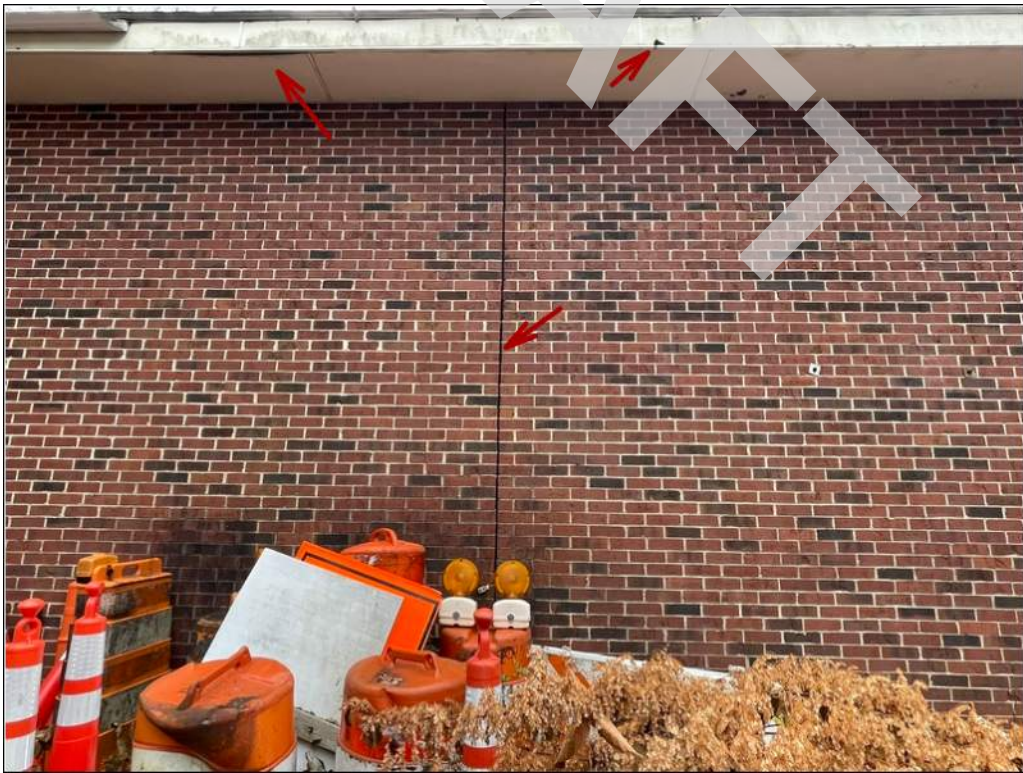
14 - Brick masonry unit wall control joint sealant is in poor condition. Soffit and fascia panels are aging.
