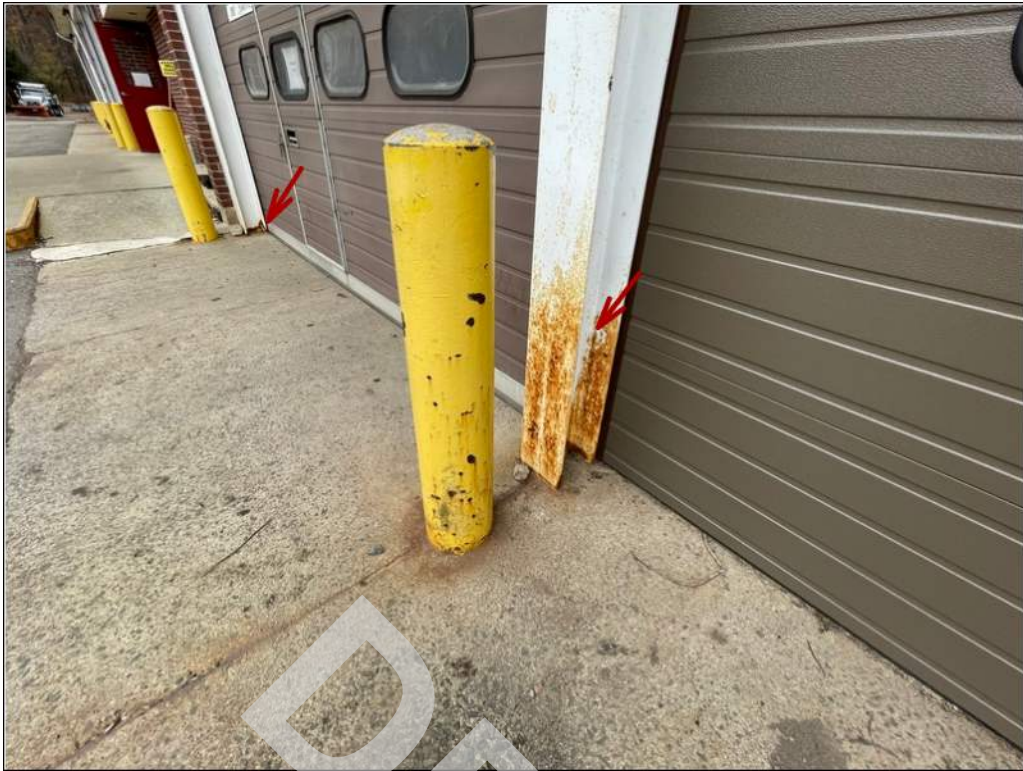
5 - Steel column surfaces have corroded.
