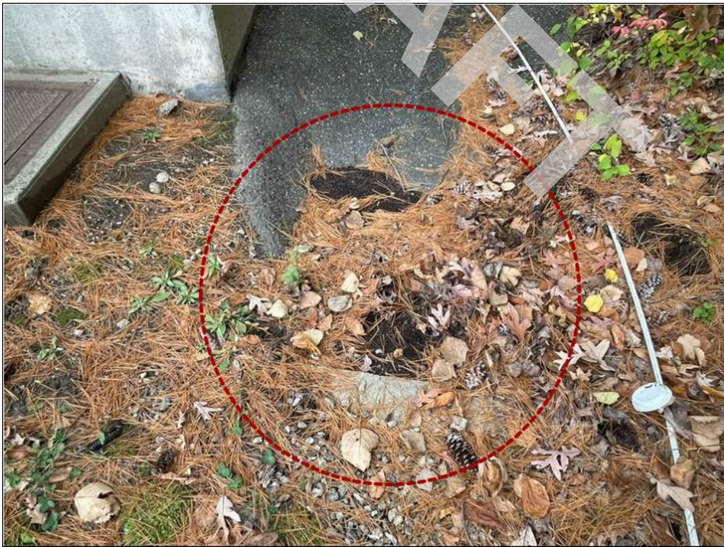
2 - Debris from the adjacent vegetation has clogged the catch basin.
