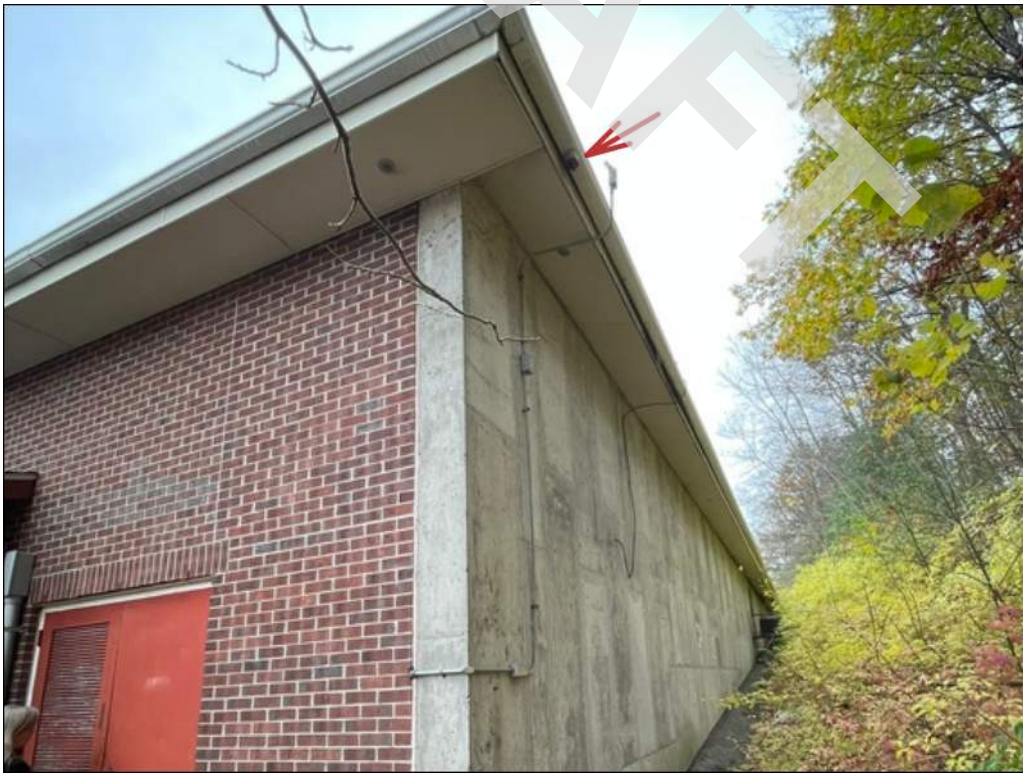
12 - A roof leader is missing along the south side of the building.
