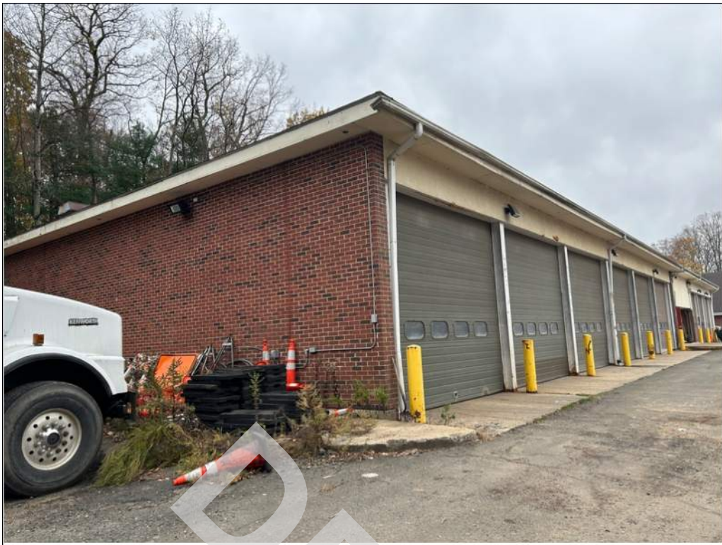
3 - Spalled concrete was observed at the concrete aprons and corrosion was noted as several bollards.
