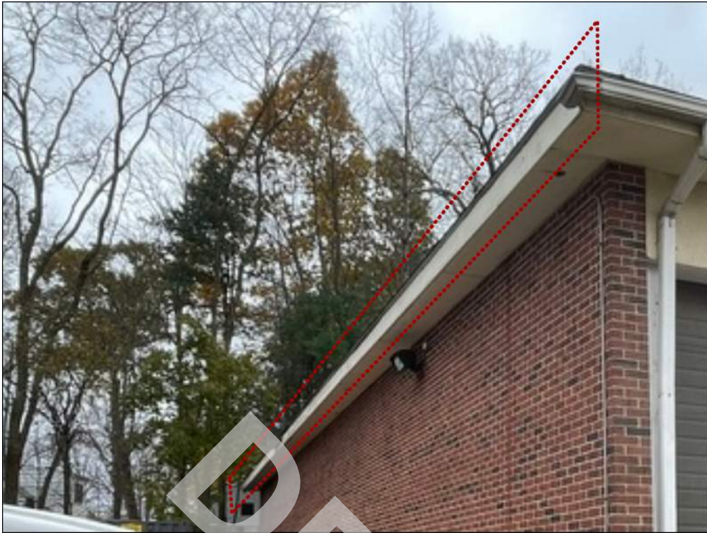
11 - Close up view of missing roof gutter along the east end of the building.
