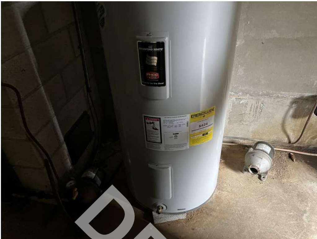
23 - An electric storage-type water heater is located in the mechanical room and provides hot water throughout the building.
