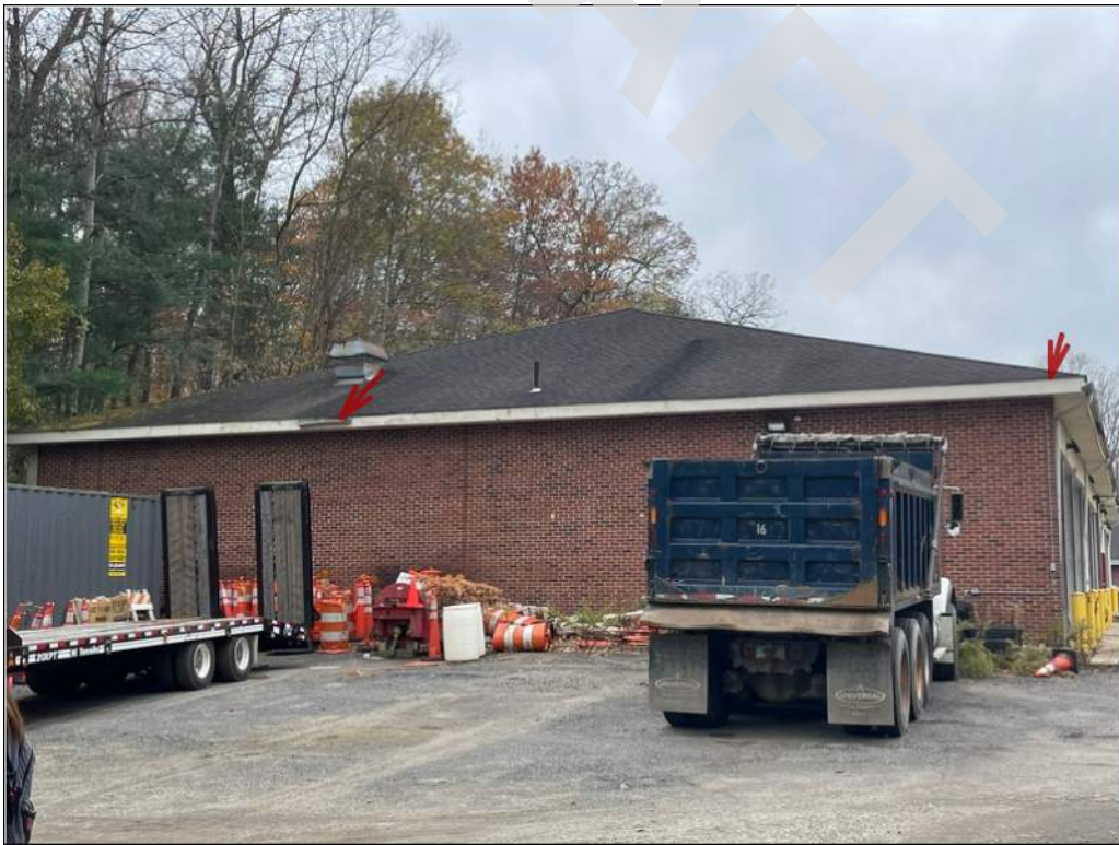
10 - Roof gutter is missing and fascia has damages along the east facade. Roof deficiencies include organic growth and stained asphalt shingles.
