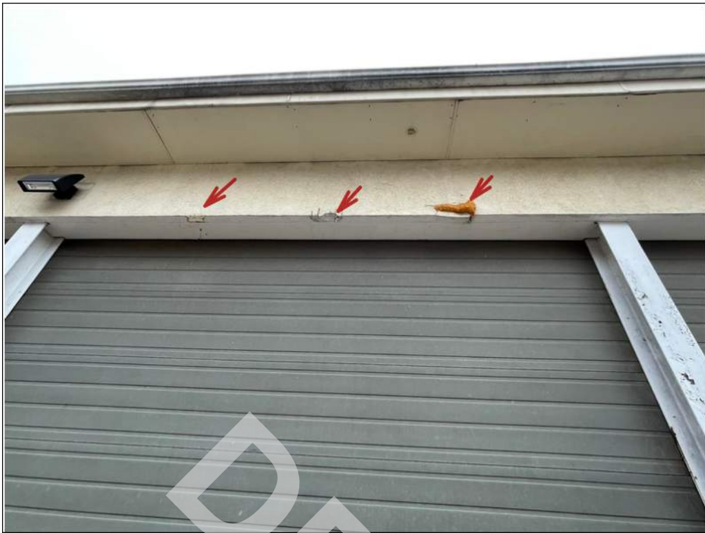
15 - Areas of the EIFS (exterior insulation finishing system) have been damaged.
