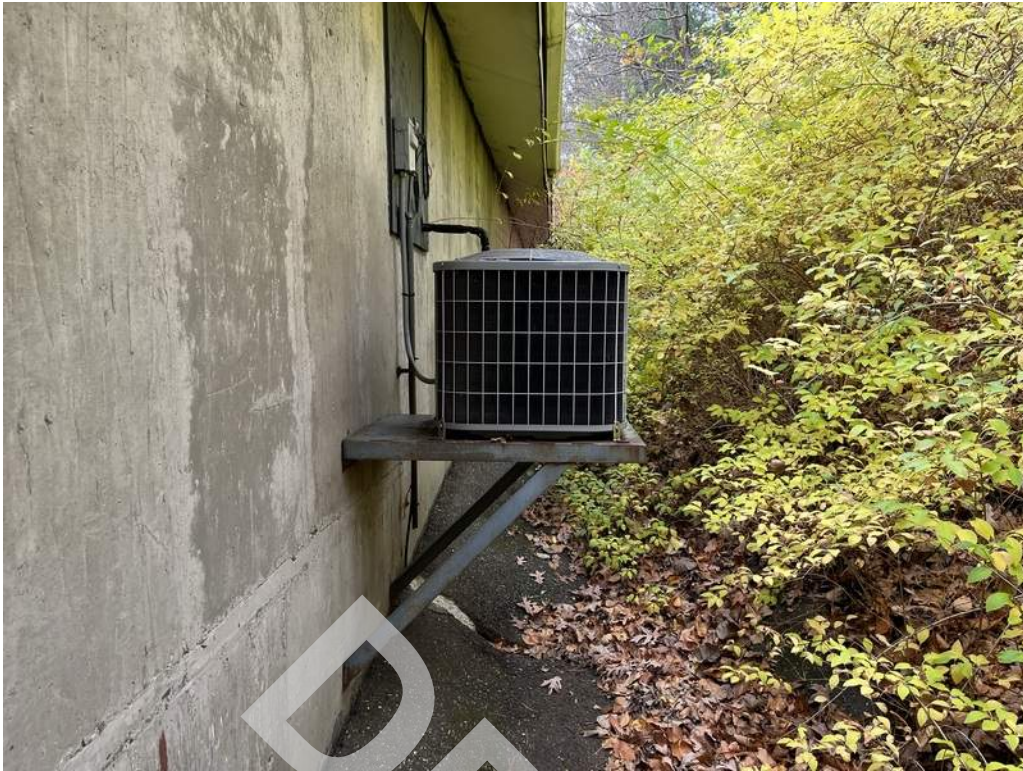
21 - A split system air conditioning unit located on the exterior of the building provides cooling to a portion of the building.
