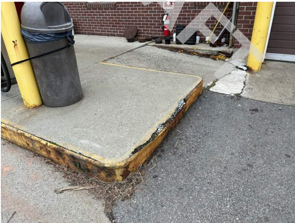
4 - Walkways exhibit concrete spalling and deterioration.
