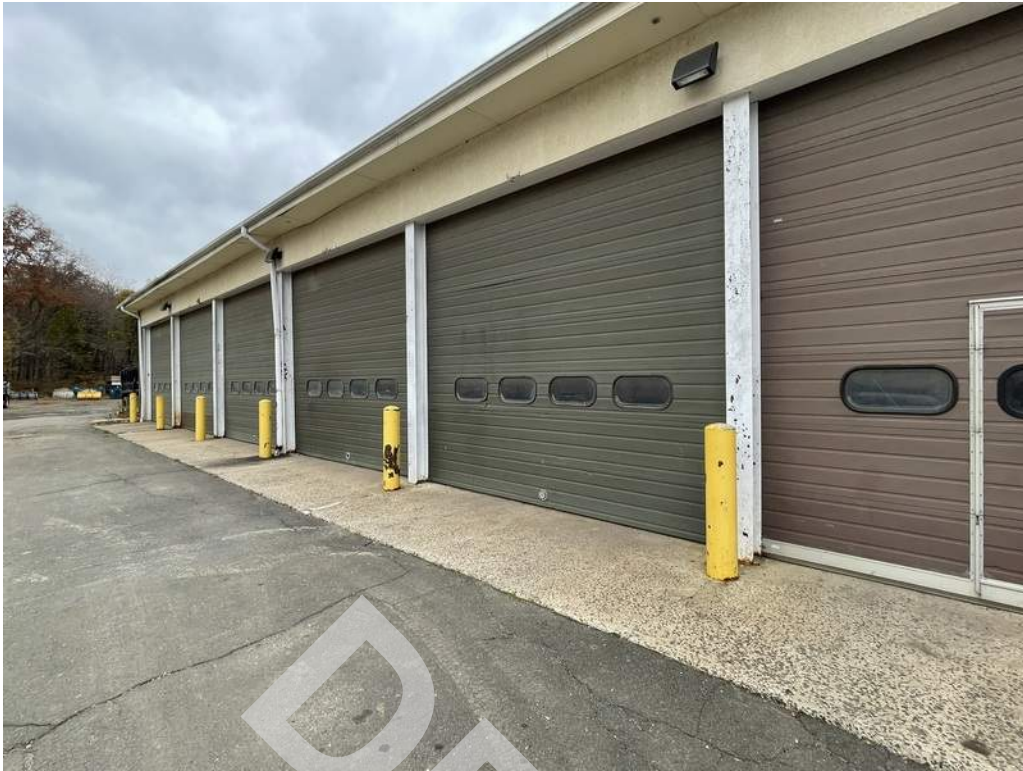
17 - Sectional overhead doors are provided at the garage.
