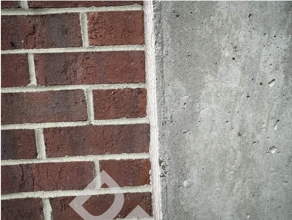
13 - The joint sealant between the brick masonry unit and concrete wall has failed.
