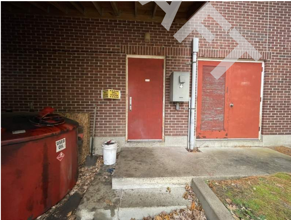
16 - Hollow metal frames and door surfaces are starting to corrode.
