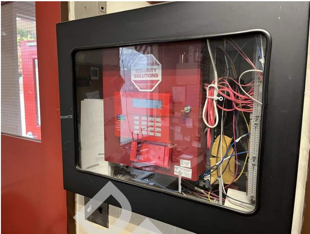
25 - The building is provided with a combination fire alarm/security alarm panel.
