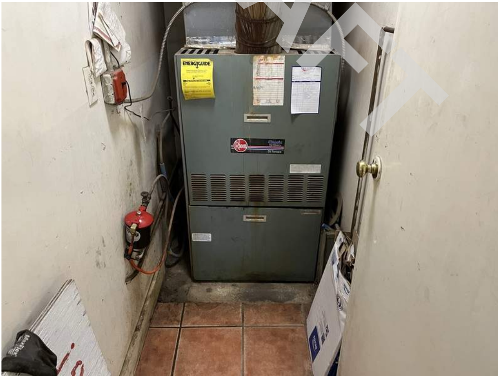
16 - Barn: An oil-fired furnace provides heating to the barn building.
