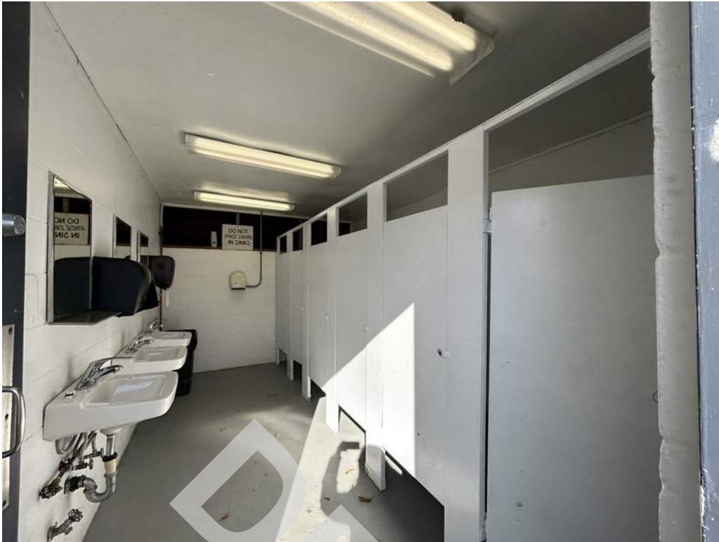
15 - Restrooms: Interior finishes consist of painted masonry walls, painted gypsum ceiling boards, and painted slabs.
