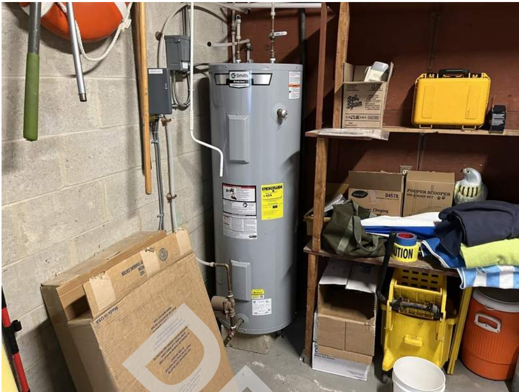
17 - The barn and restroom facility are each provided with an electric storage-type water heater which provides hot water to each building.
