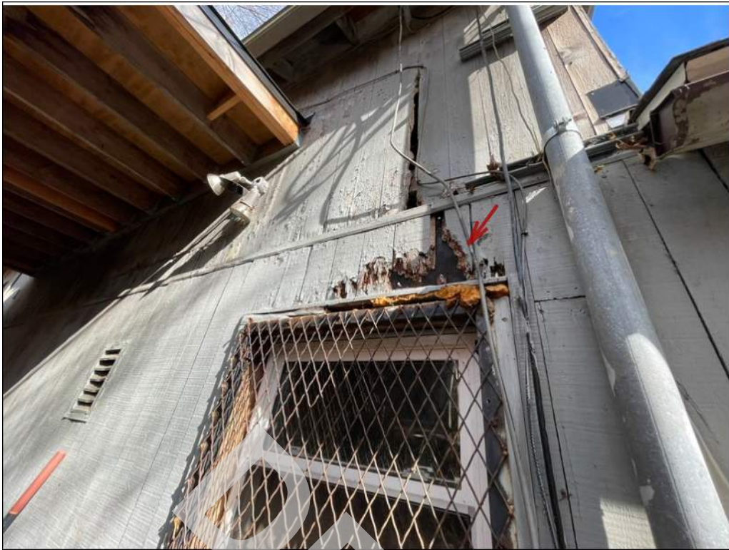
11 - Barn: Localized areas of the wood cladding are rotting.
