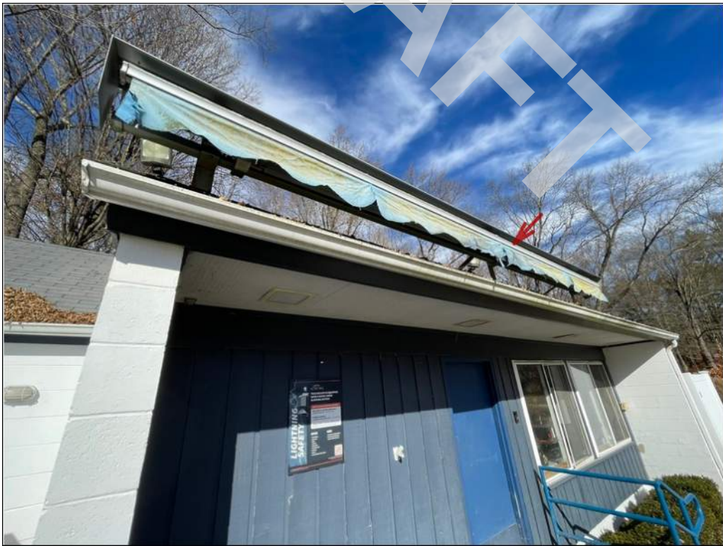
6 - Restrooms: A retractable fabric awning sits atop the asphalt shingles. Fabric is ripped.
