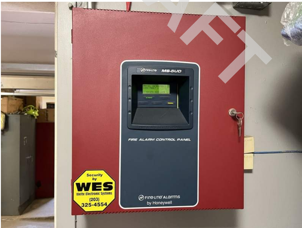
18 - Barn: The building is provided with a Fire-Lite MS-5UD fire alarm panel located in the main room of the building. The panel's "Trouble" light was on at the time of the site visit.
