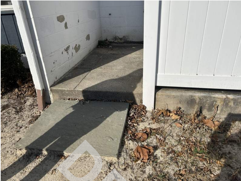
23 - Restrooms: An accessible route to the men's restroom is not provided.
