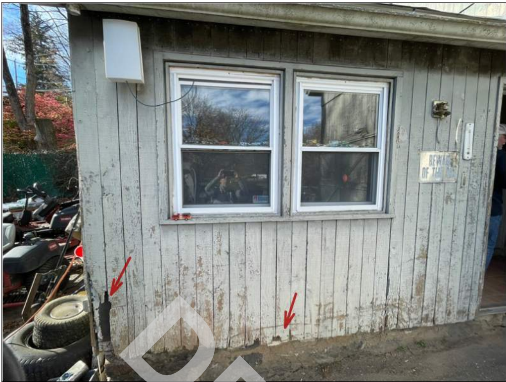
9 - Barn: Wood plank facade is in poor condition, including broken wood planks.
