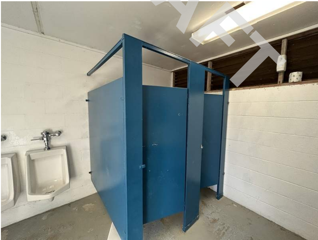
24 - Restrooms: Accessible stalls and urinals are not provided.
