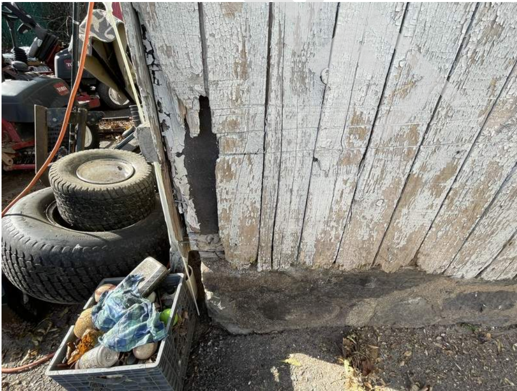
10 - Barn: Close up view of damaged wood and paint finish.
