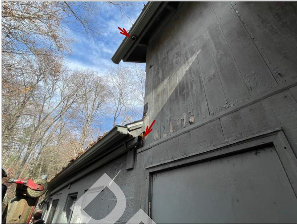
7 - Barn: A roof leader is missing along the west side of the barn.
