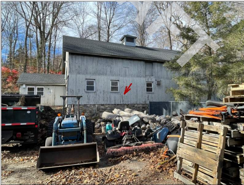
8 - Barn: Paint over, the wood cladding is peeling.
