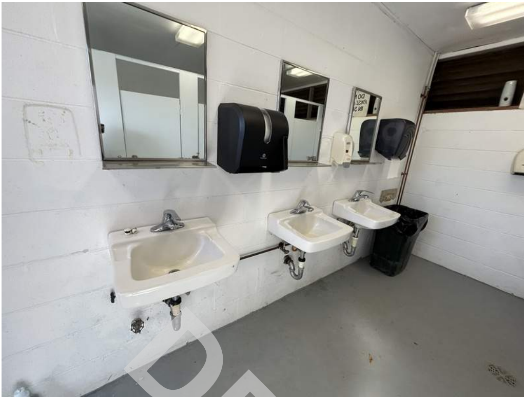
25 - Restrooms: Scald guard protection is not provided under the sinks.
