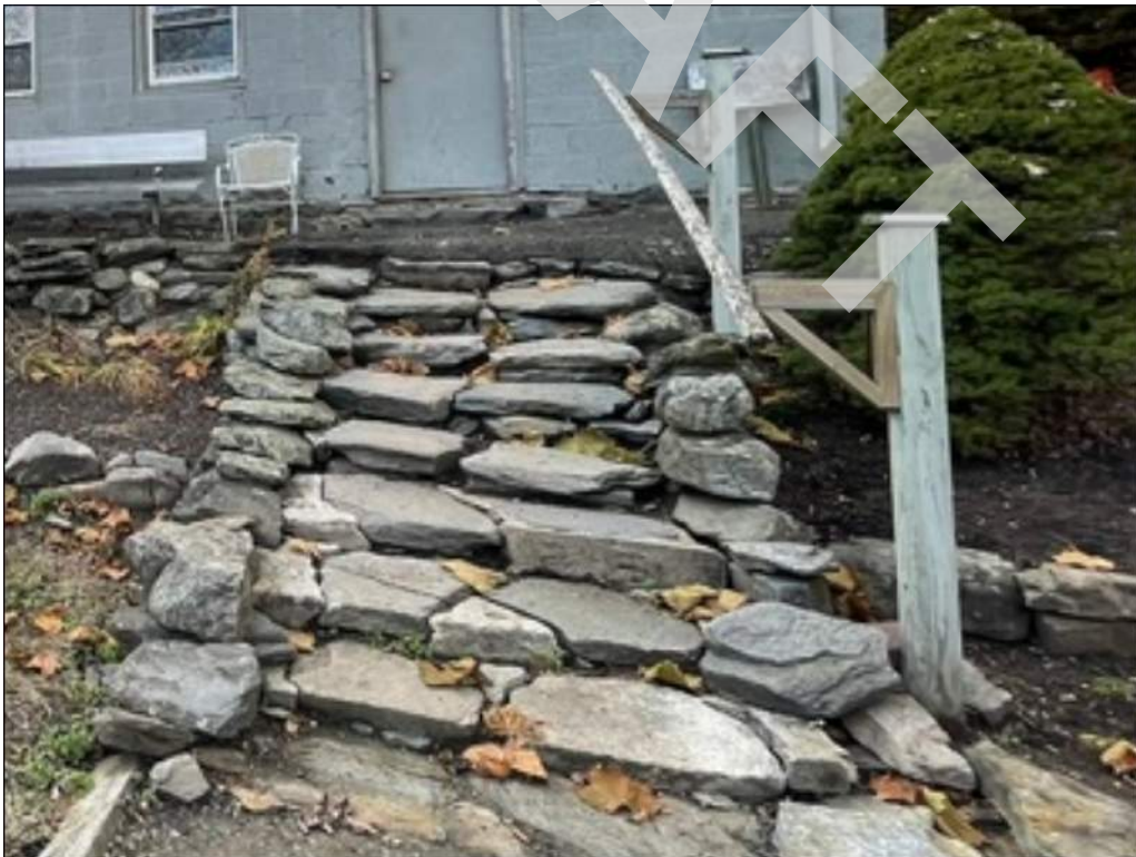
12 - Barn: Rock stair and landing are in poor condition; surfaces are uneven and a second handrail is not provided.
