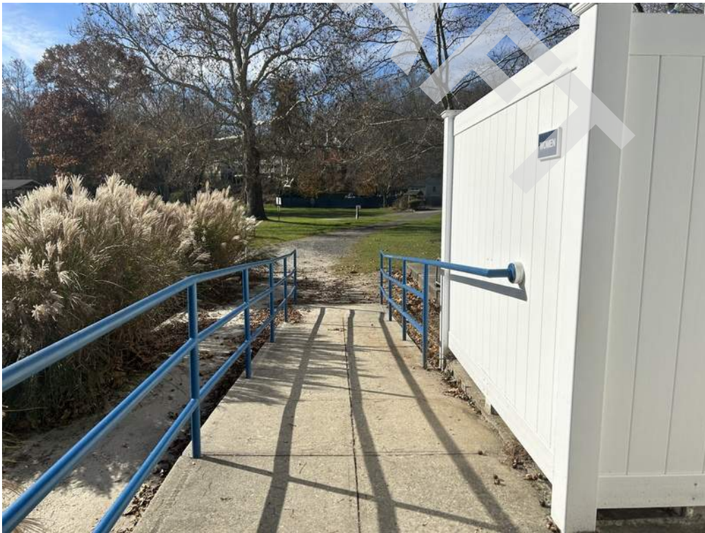
22 - Restrooms: The ramp at the Merwin Meadows Restroom does not provide edge protection on both sides, handrail extension at the bottom of the ramp, and a compliant bottom landing.
