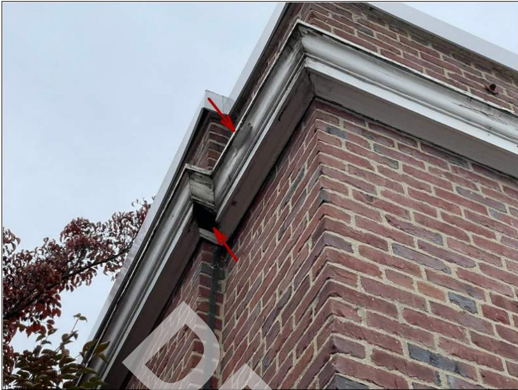
27 - Decorative wood trim cornices have rotted and have peeling finishes.
