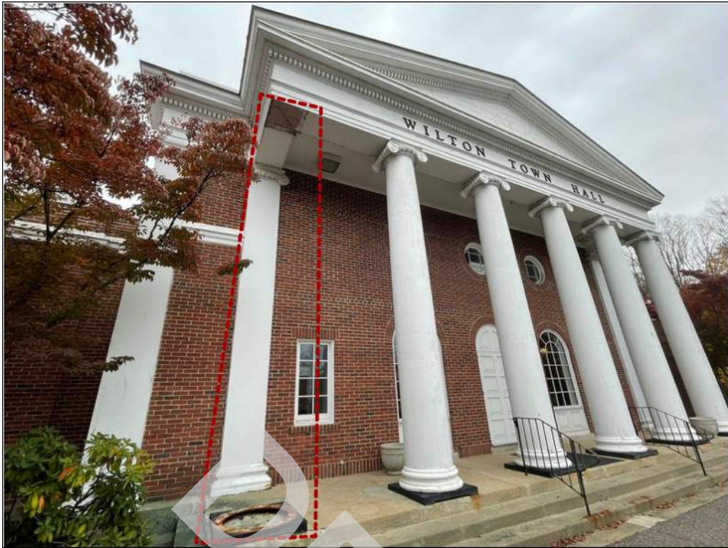
9 - Missing column along the front facade.
