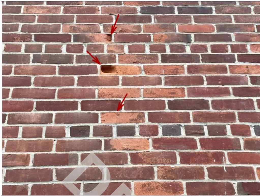
17 - Localized areas of the brick masonry unit facade have spalled units.
