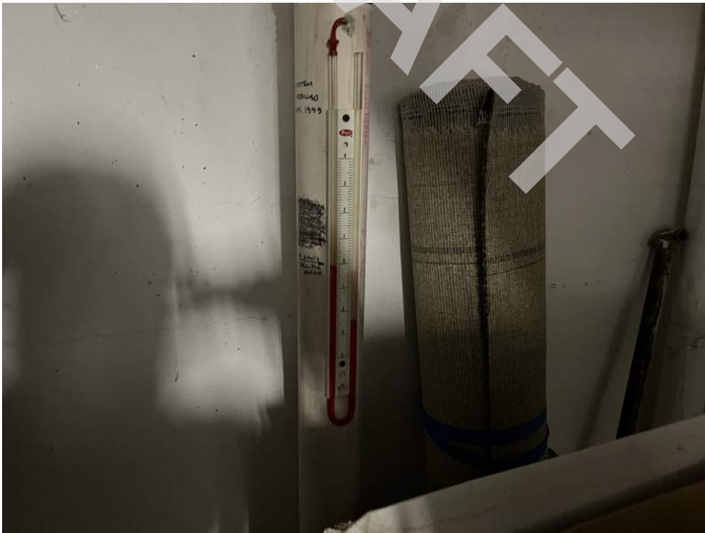
46 - A radon mitigation system is provided within the building.
