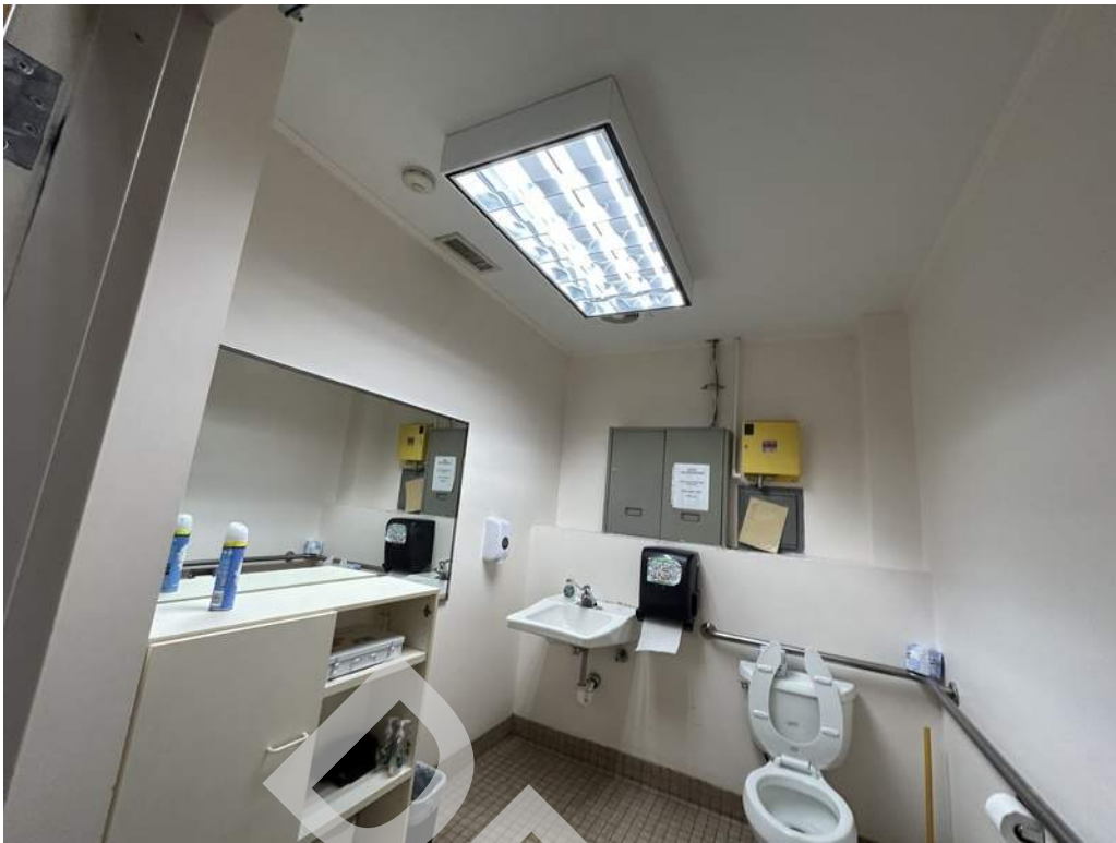
59 - The single user restroom on the ground floor was noted to have various non-compliant items. Items include center of toilet mounted above the the range tolerance from the side wall, inadequate sink depth and clear floor space, and missing scald guard protection beneath the lavatory.
