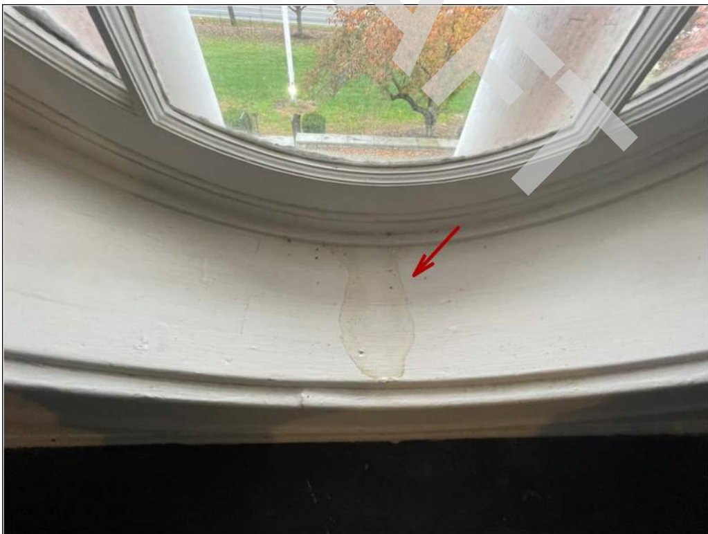
22 - Signs of water intrusion through the round windows along the main facade. Windows are single pane glass units with no safety glazing.
