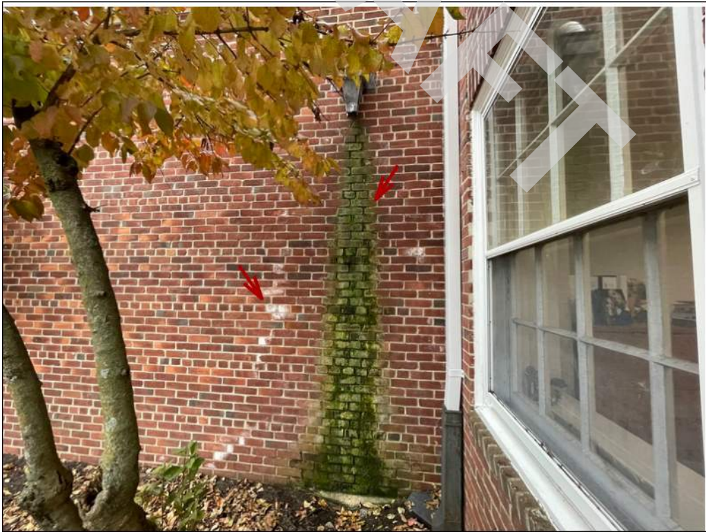
18 - Areas of the brick masonry facade have efflorescence and organic growth. Roof leader is missing.
