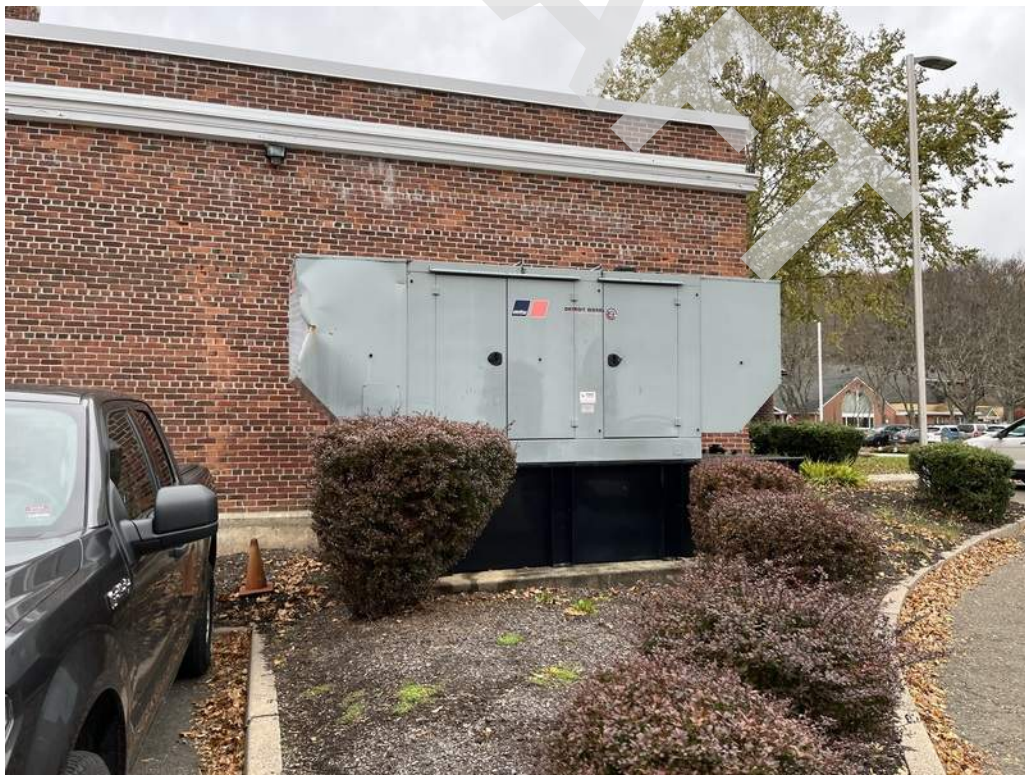
50 - A diesel-fired emergency generator located on the exterior of the building provides emergency power to the Town Hall and Annex buildings.
