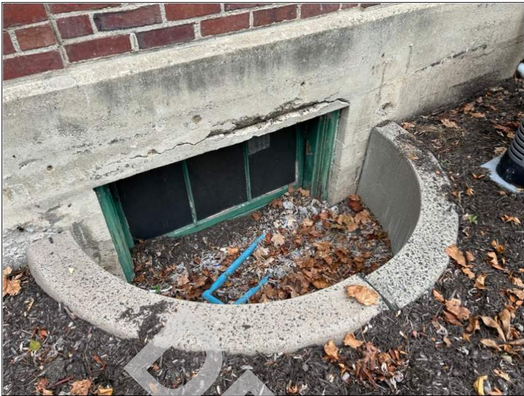
7 - Reinforced concrete foundation wall has spalled and has exposed steel reinforcement.
