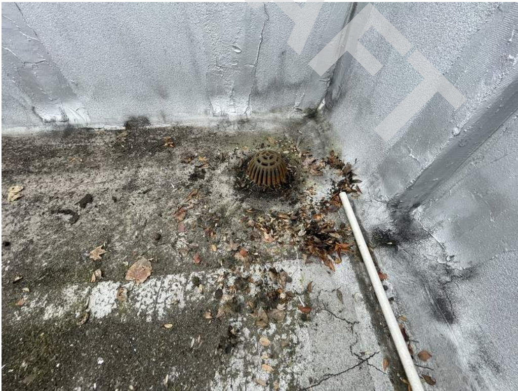
16 - Debris accumulation and organic growth around the lower roof.
