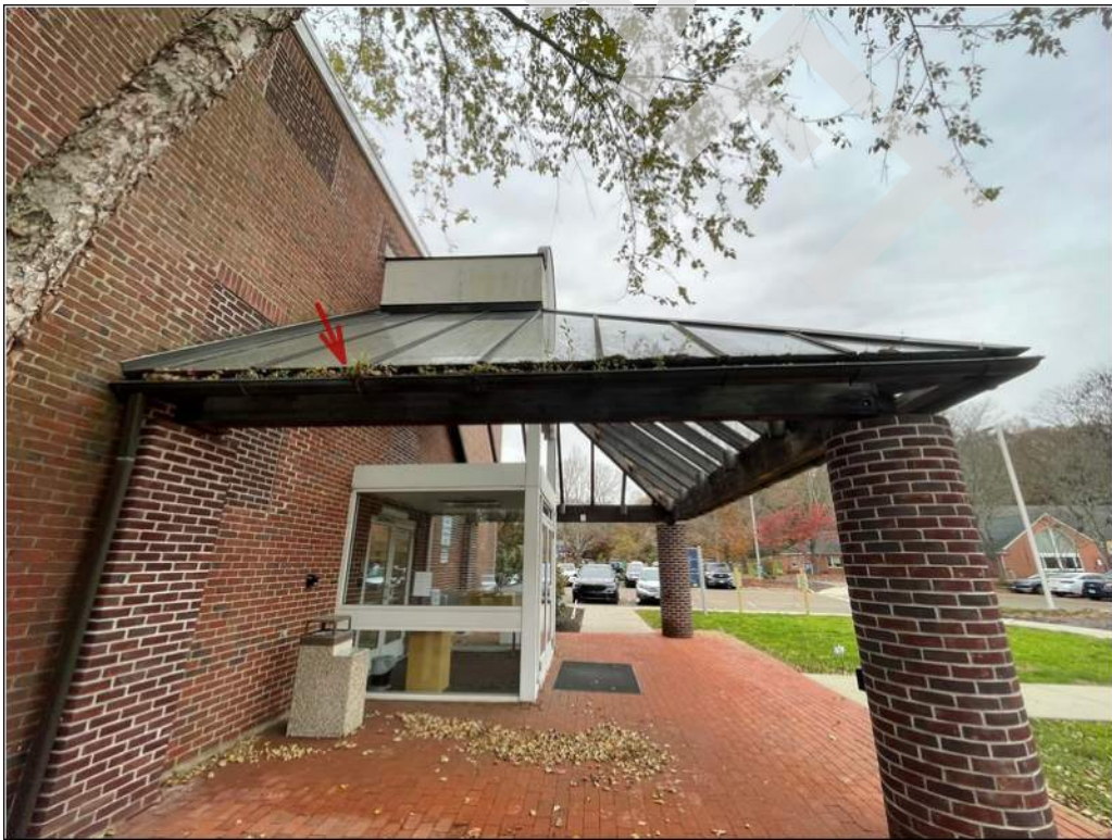
14 - Vegetation and debris accumulation at the roof gutters.
