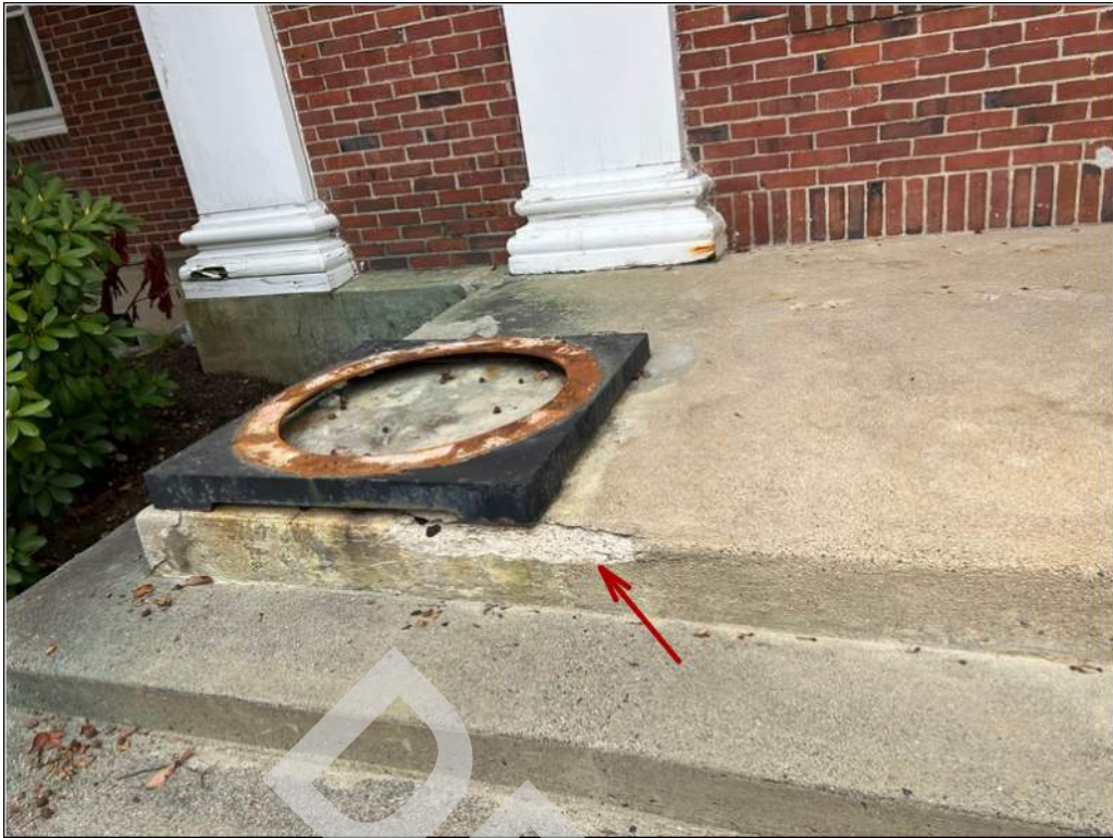
11 - Reinforced concrete at the main entrance plinth has spalled.
