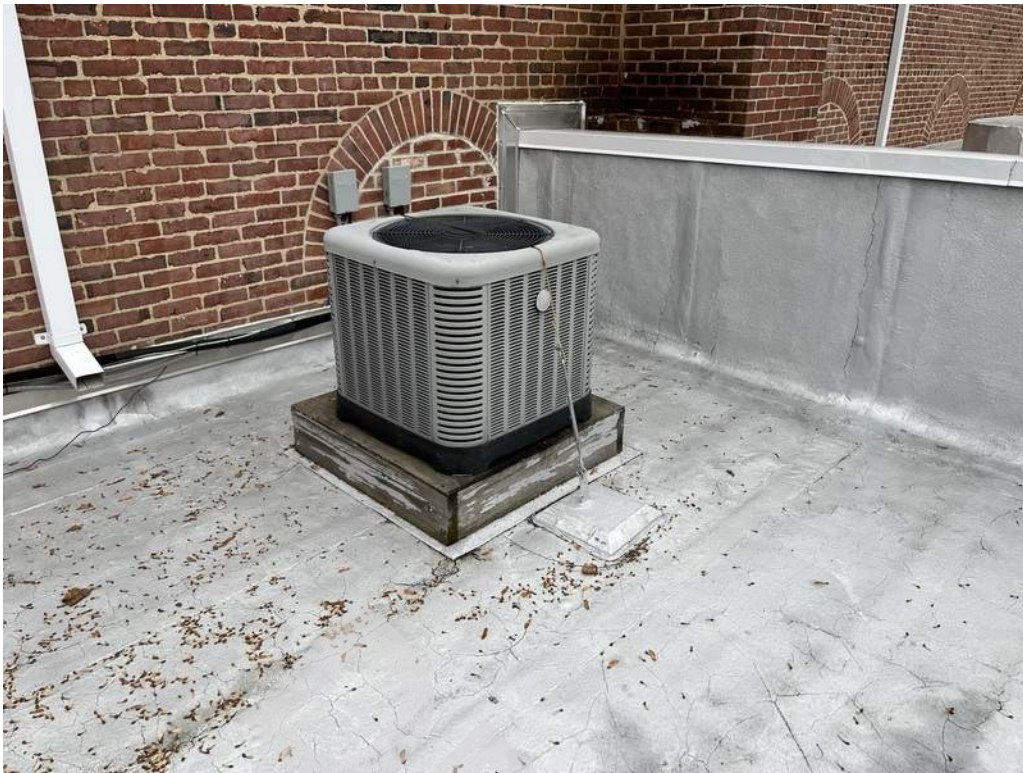
43 - Split system air conditioning units are located on the roof and provide cooling to the office areas of the building.
