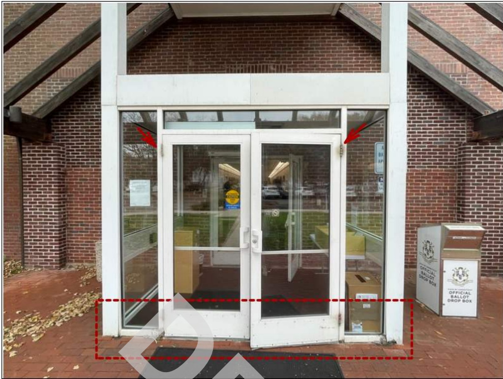
23 - The rear entrance storefront system has deteriorated. Damages include corrosion at the hinges and storefront framing along the base.
