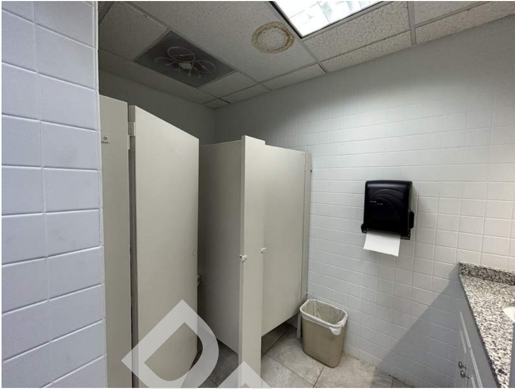
61 - An accessible stall is not provided at the multi-user restroom on the first floor.
