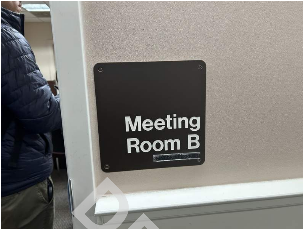
57 - Signage is mounted below the required height and is non compliant.
