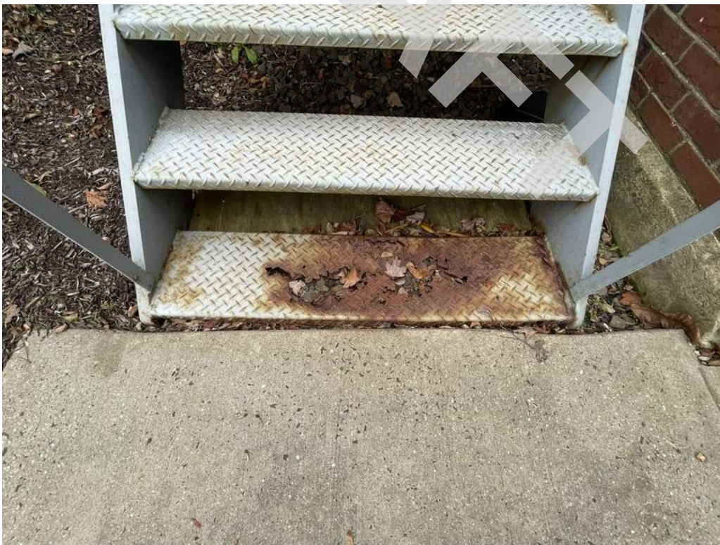
32 - Pitting corrosion at the lowest metal riser.
