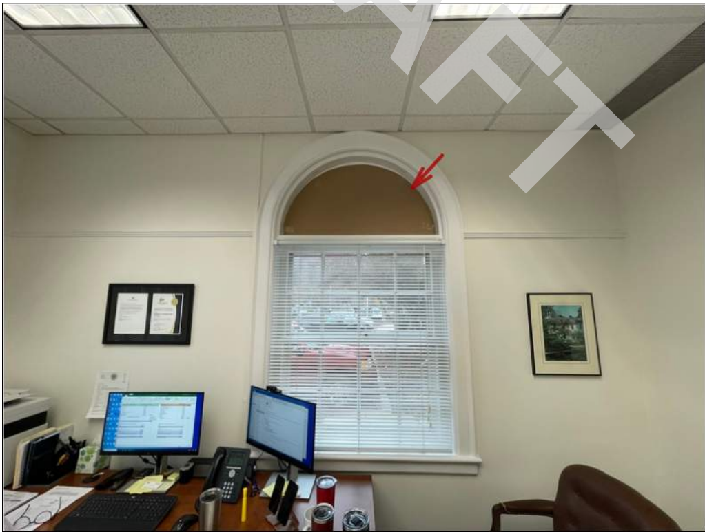
20 - A portion of the window units have been covered with cardboard.
