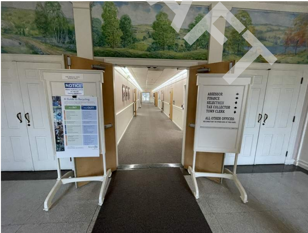
52 - Fire rated doors are held open by signage.
