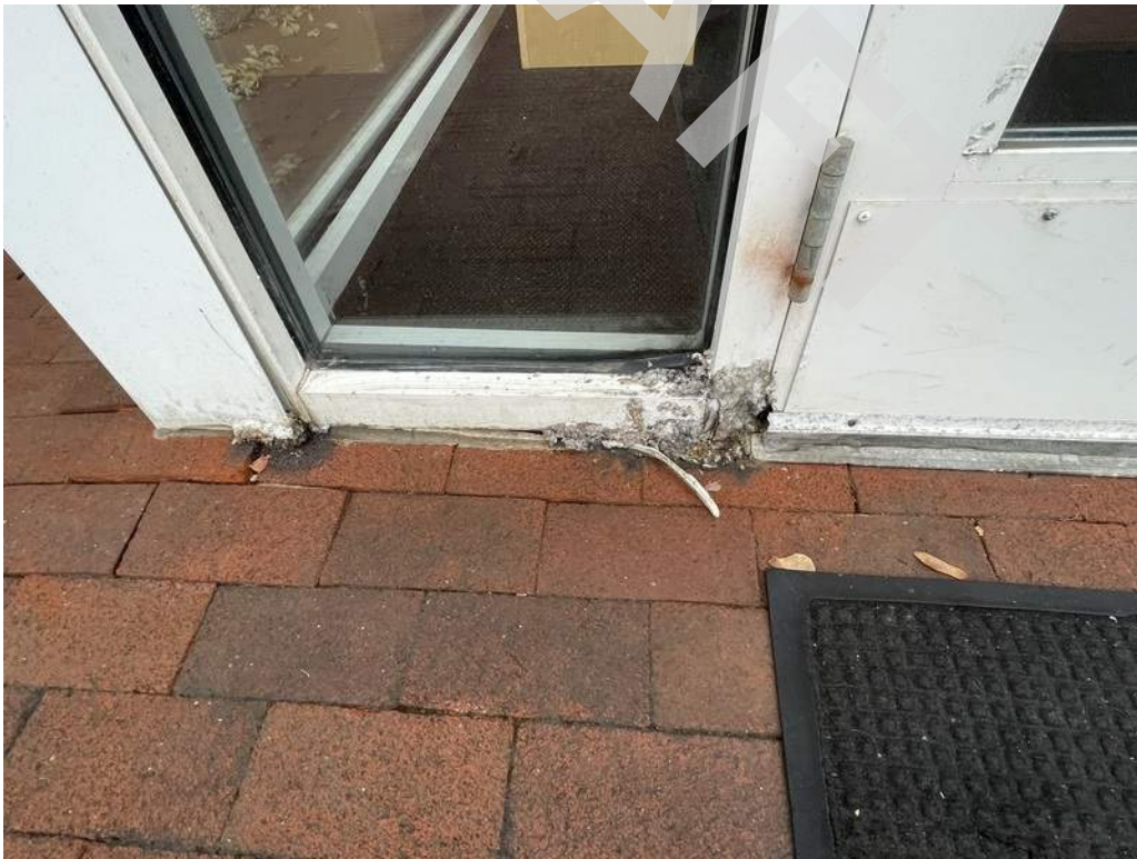
24 - Close up view of the corroded storefront framing components.
