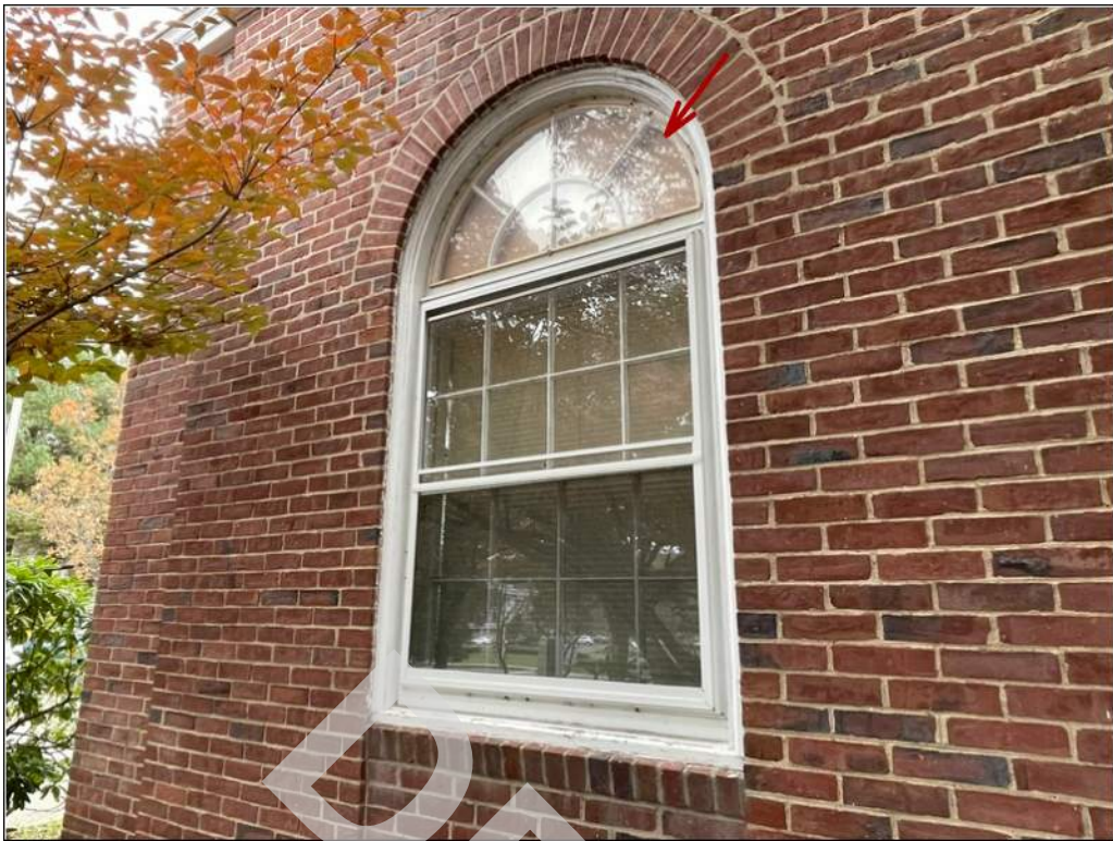
19 - Most of the window units have been covered with a plastic screen on the exterior.
