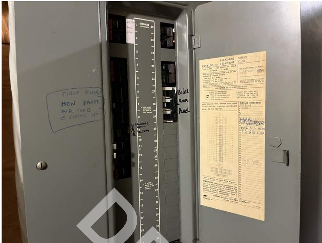
49 - Two electric panels located in the electric service room are Stab-Lok model Federal Pacific panels.
