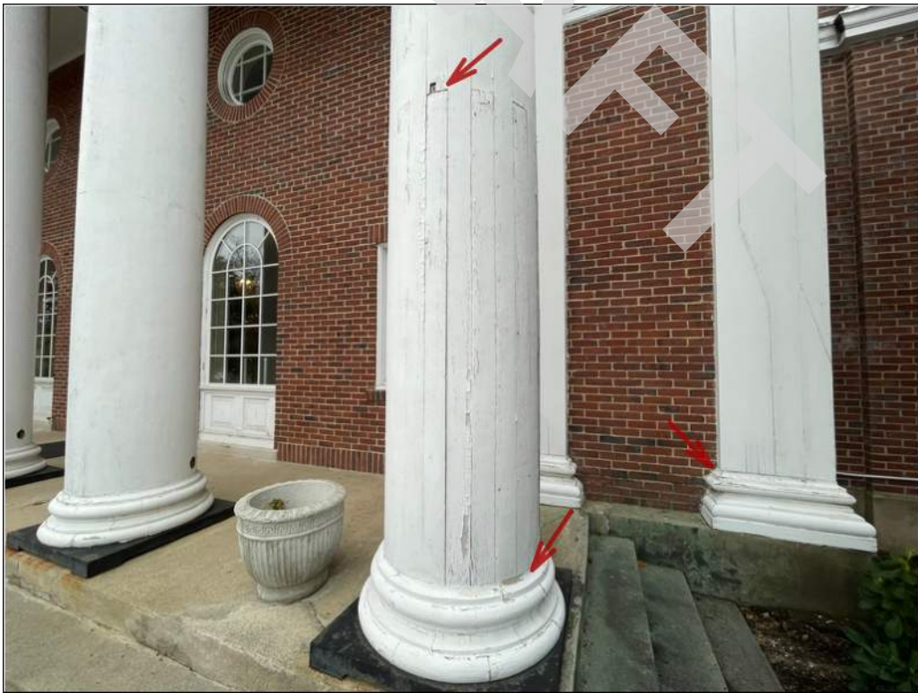
10 - Front facade wood column surface has localized damages and damaged finishes.
