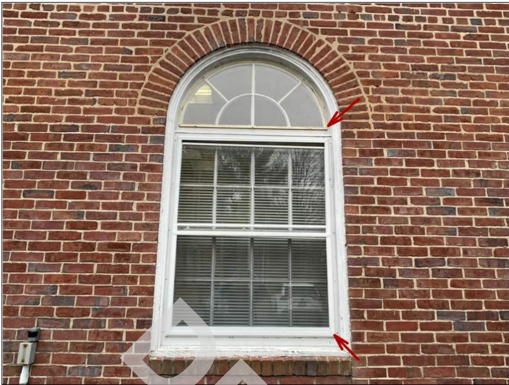
29 - Window assemblies consist of wood framed single pane units. Windows are provided with plastic coverings.
