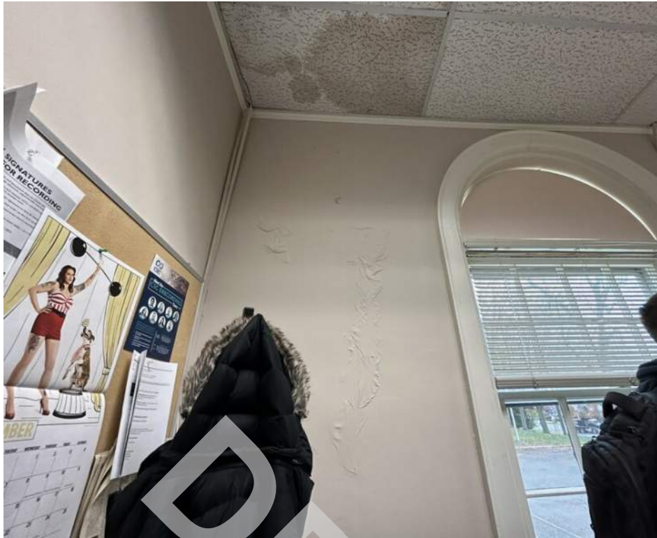
39 - Stained ceiling tiles and paint blisters were observed on the first floor.
