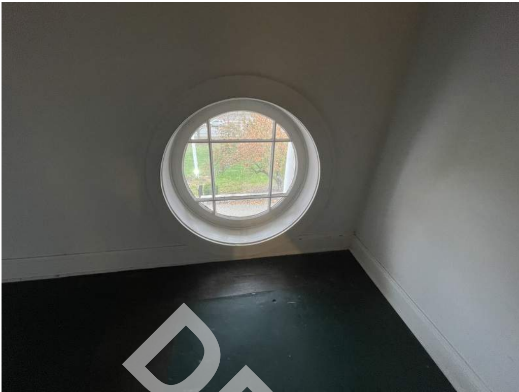
21 - Round windows along the front facade do not appear to include safety glazing.
