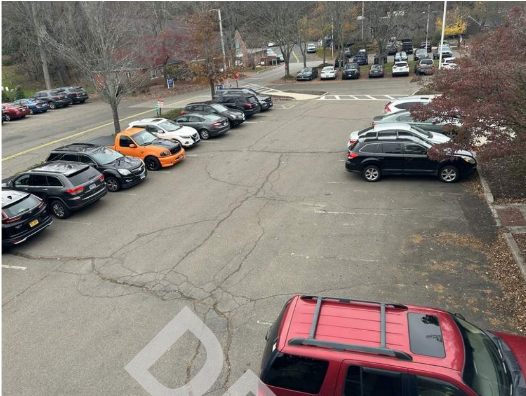
5 - Parking is provided along the north side of the building. Faded striping and alligator and longitudinal cracking was observed throughout the paved parking areas and drive lanes.
