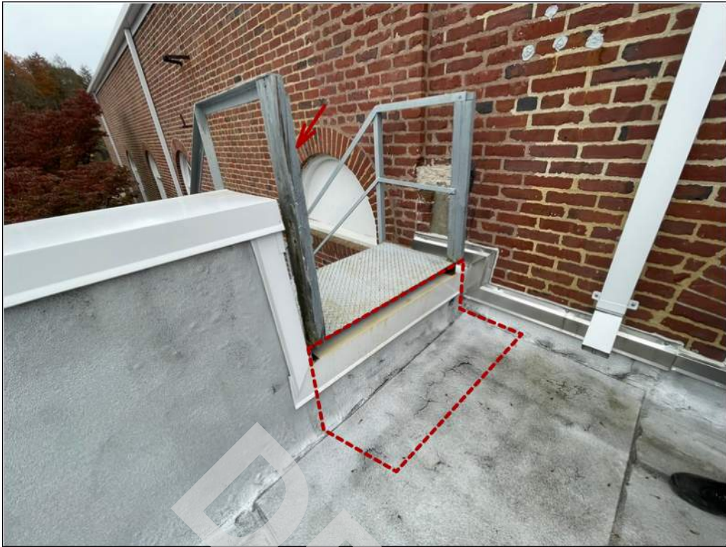
33 - Height of the riser in the path of egress is above the code requirement. Previously repaired handrail support.
