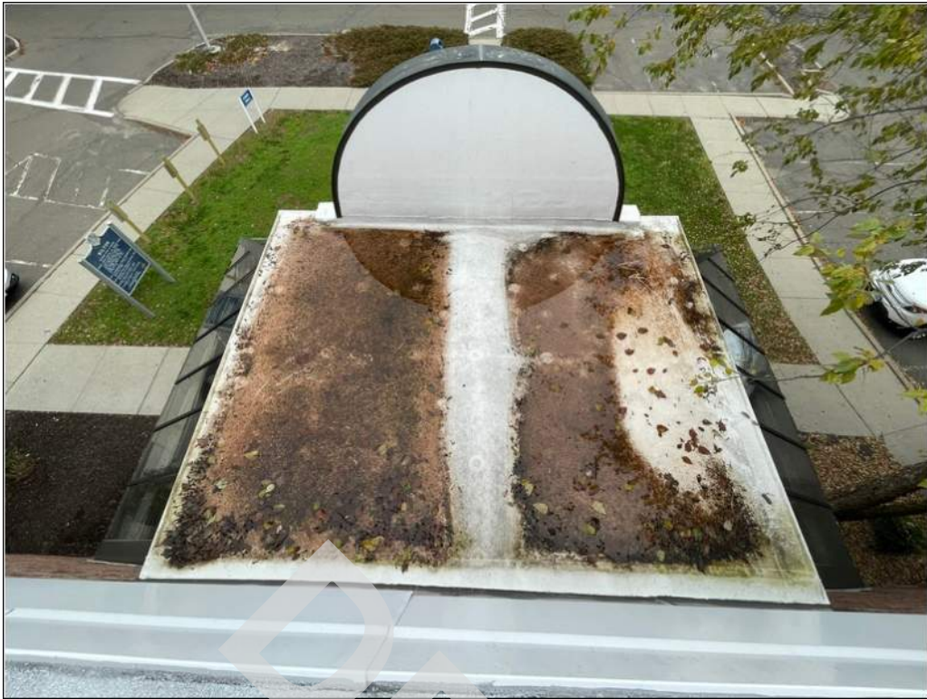
15 - Debris accumulation and water ponding at the low roof over the secondary building entrance.
