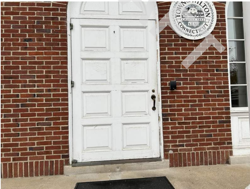
26 - Main entry wood door is in poor condition. Deficiencies include deteriorated door hardware and peeling finish surface.
