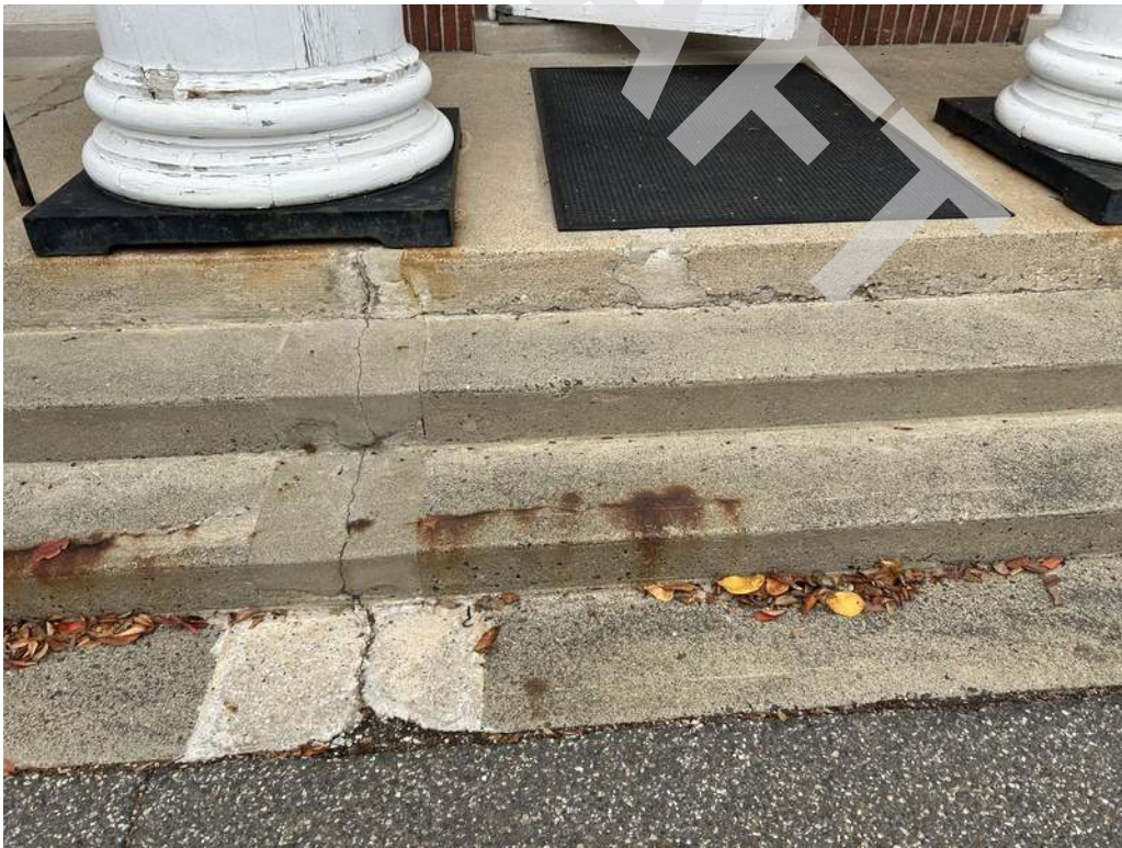
12 - Evidence of prior patching along with additional cracking and corrosion are present at the front concrete porch.
