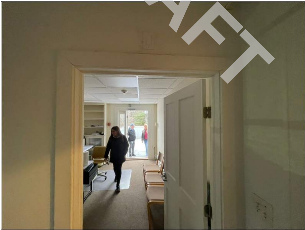
54 - Exit signage is not provided at the second floor.
