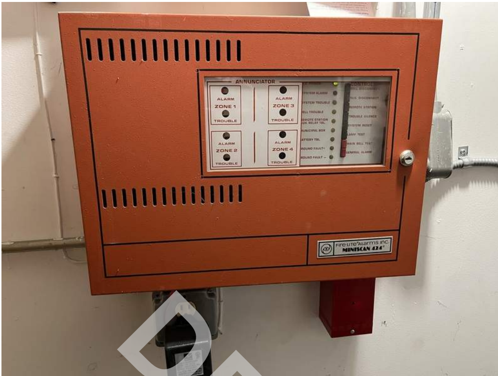
51 - The building is provided with a Miniscan 424 Fire Alarm Panel.
