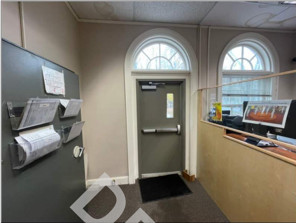
53 - Exit signage and pull alarm are not provided at the egress door.
