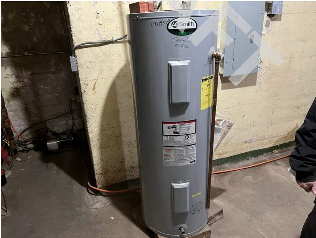
48 - An electric storage-type water heater is located in the basement and provides hot water throughout the building.
