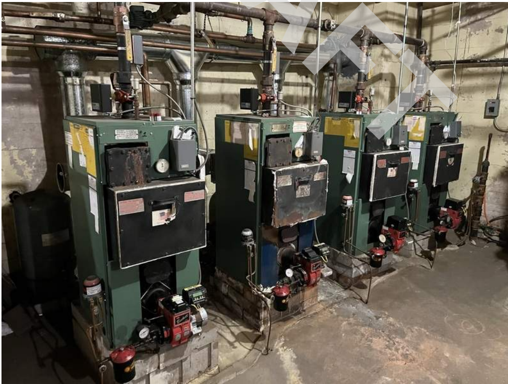
42 - Four propane fired boilers located in the basement provide heating hot water throughout the building. All four are currently operational. Insulation is not provided on the associated piping.
