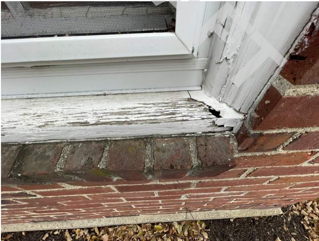
30 - Wood and brick sills are in poor condition. Wood is rotted and brick sill has organic growth, spalled brick units, and deteriorated mortar joints.
