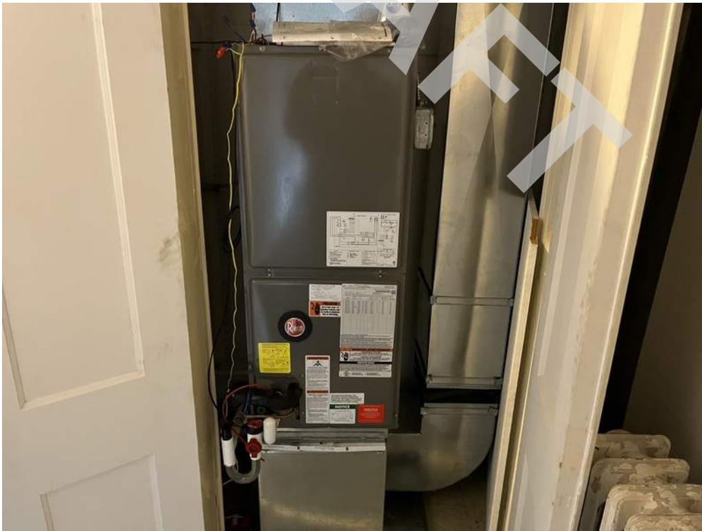
44 - Split system indoor air handling units with auxiliary electric heaters are located within the building and provide air conditioning through ductwork throughout the building.
