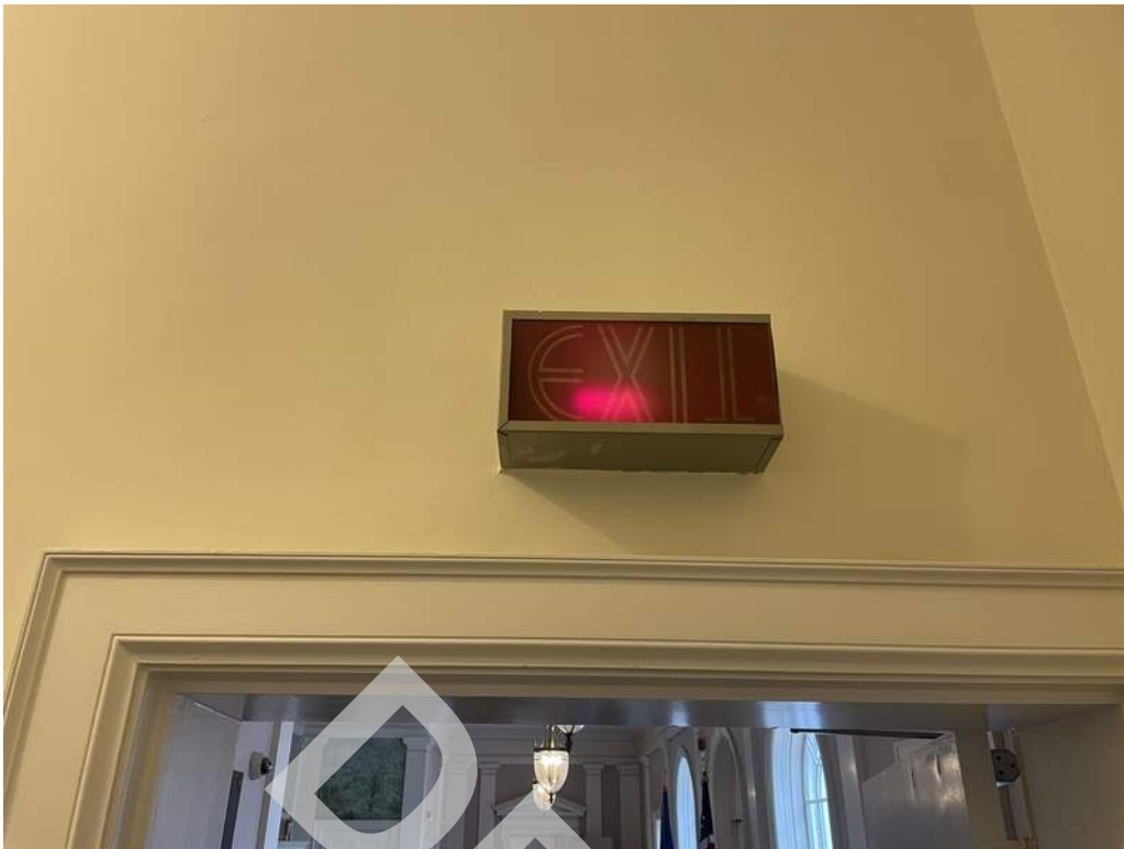
55 - Illuminated exit signage is outdated.
