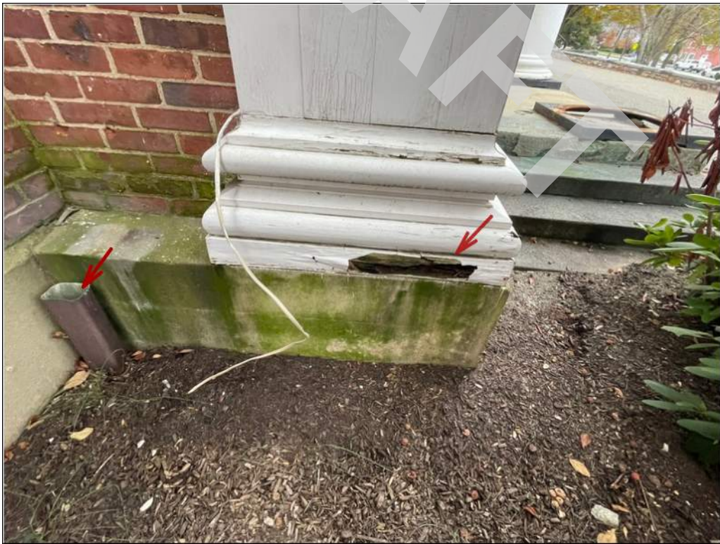
28 - Wood pilaster surfaces have rotted and have peeling finishes. Roof leader is missing.
