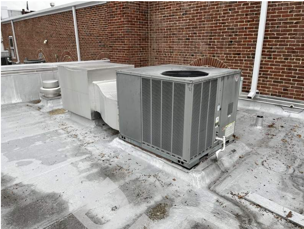
45 - A rooftop packaged unit provides cooling to the vault room on the first floor.
