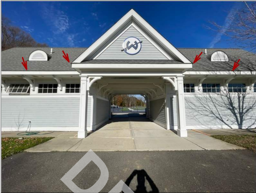
3 - No gutters or leaders are provided throughout the building.
