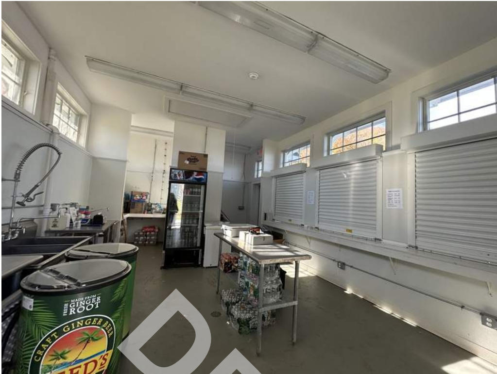
7 - Interior kitchen finishes consist of painted gypsum board ceiling and boards and painted concrete slabs.
