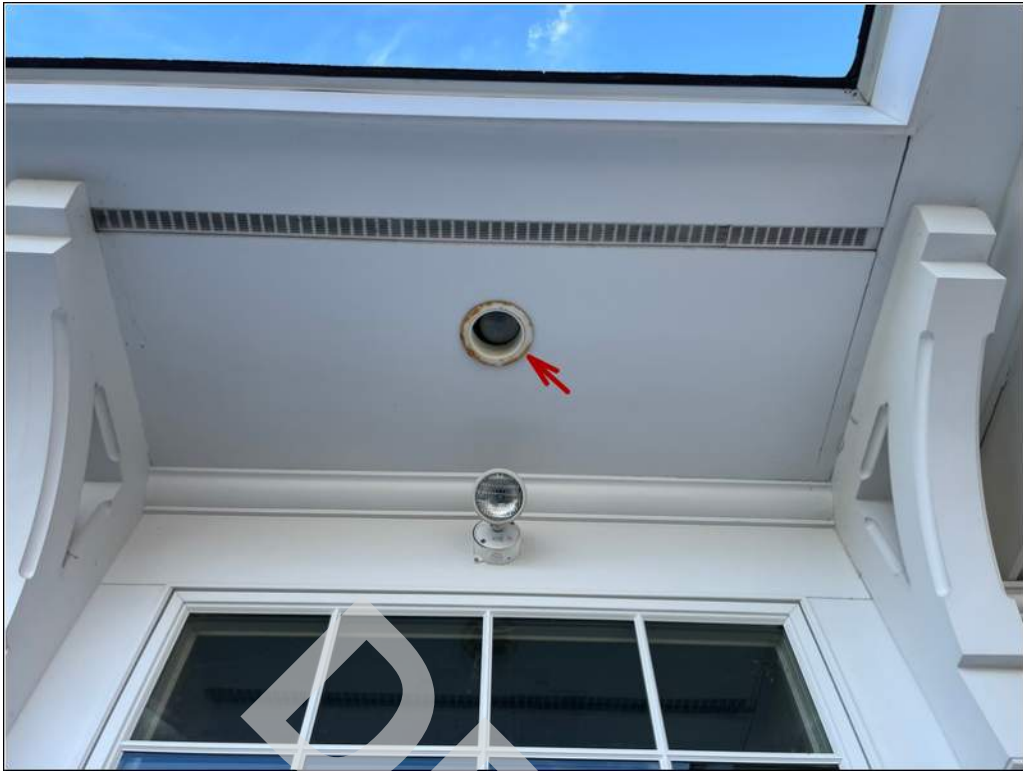
5 - Recessed lighting metal rings have corroded due to water and moisture exposure.
