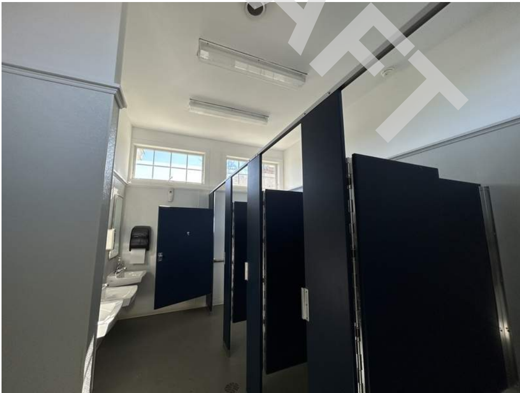
8 - Interior restroom finishes consist of painted gypsum board ceiling and boards and painted concrete slabs.
