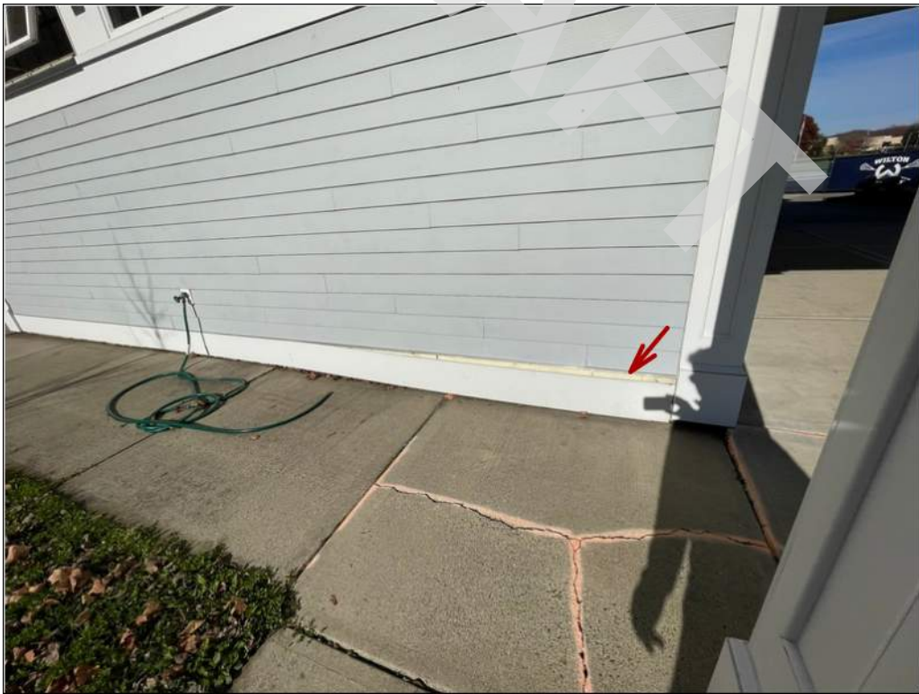
6 - Fiber cement base has displaced and detached from the facade.
