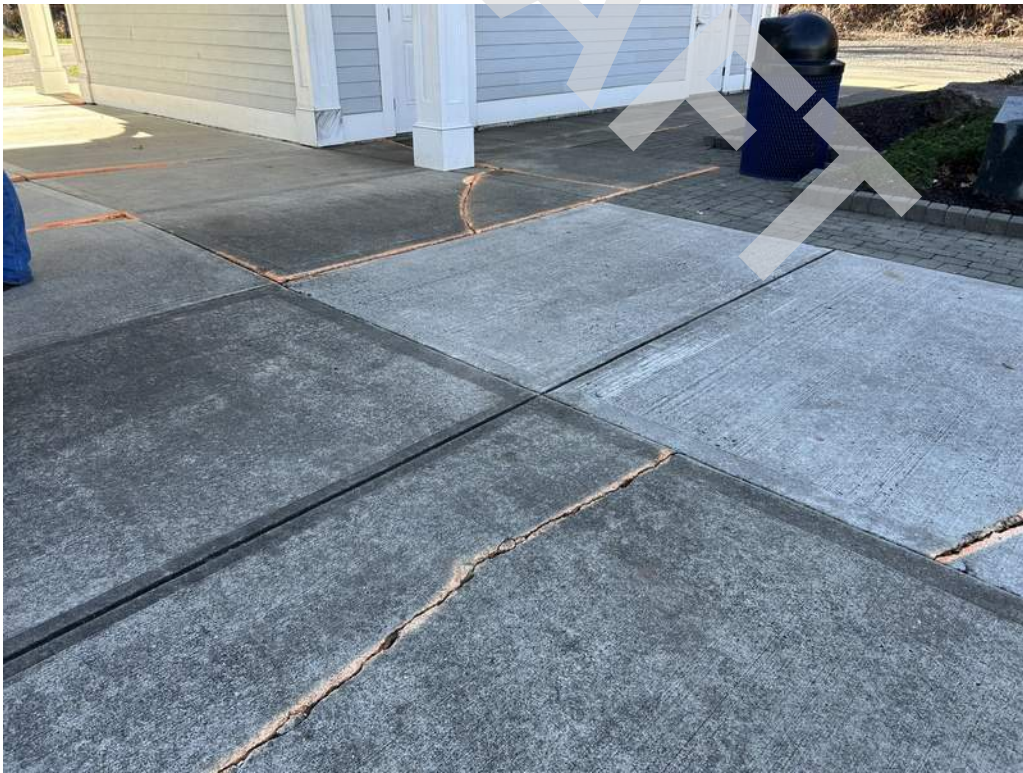
2 - Extensive cracking and vertical displacement was observed throughout the cast-in-place concrete paths.
