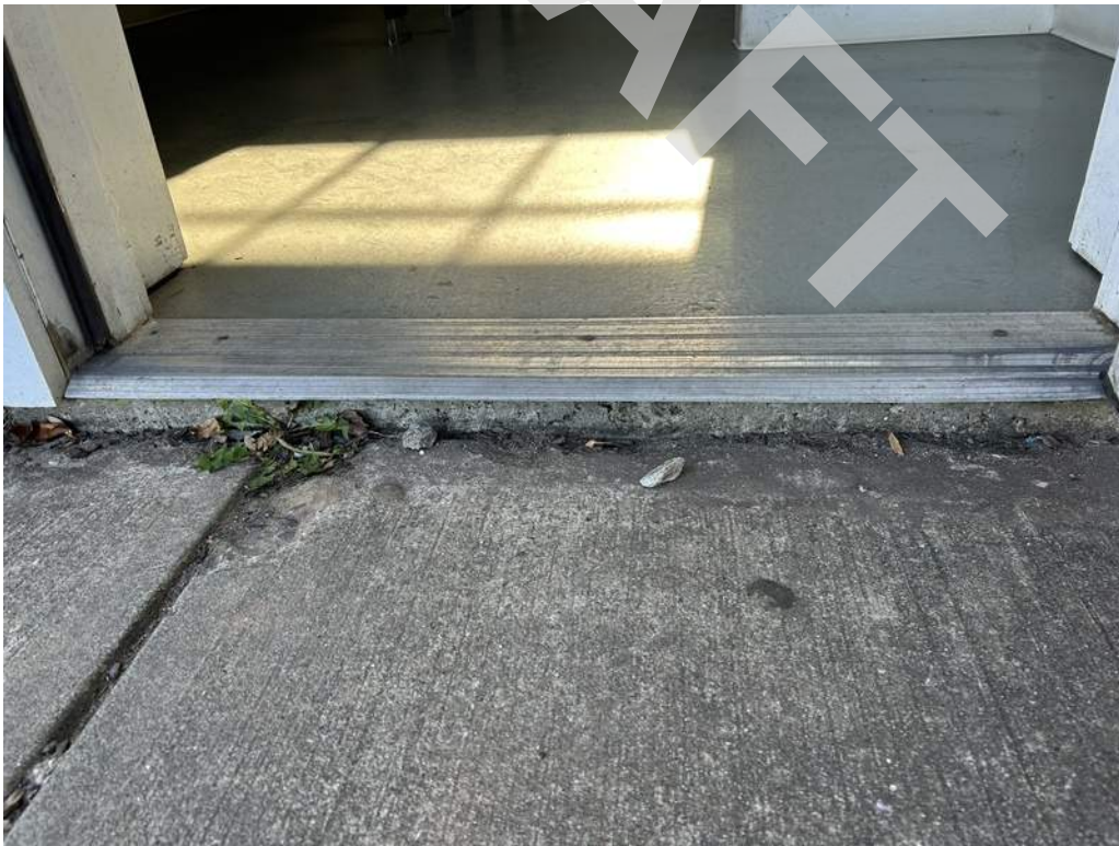
10 - The restroom door threshold exceeds the allowable height.
