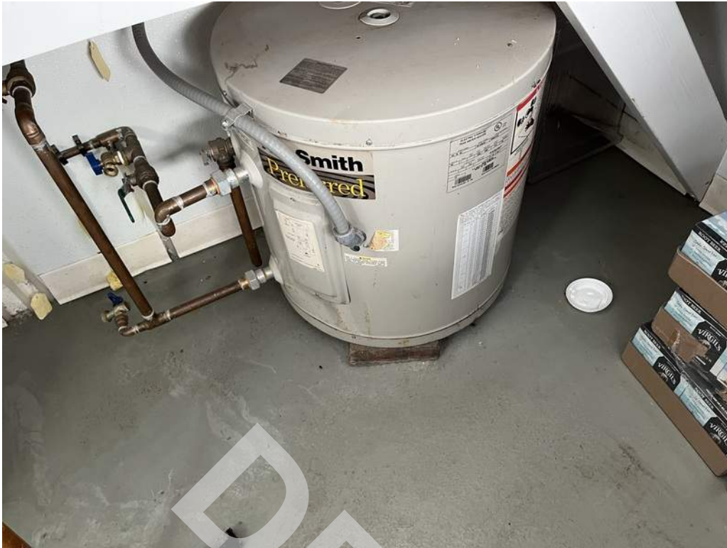
9 - Two electric storage-type water heaters provide hot water to the building.
