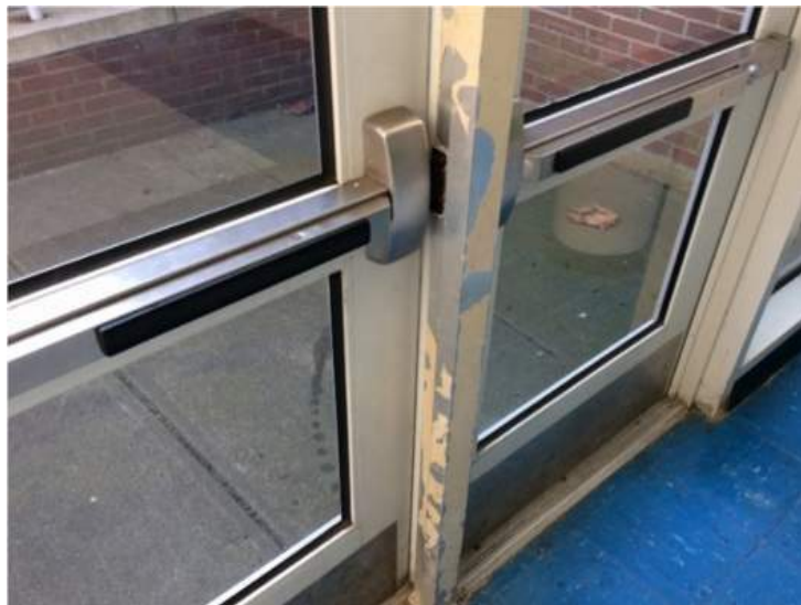
Poor functioning exterior doors
