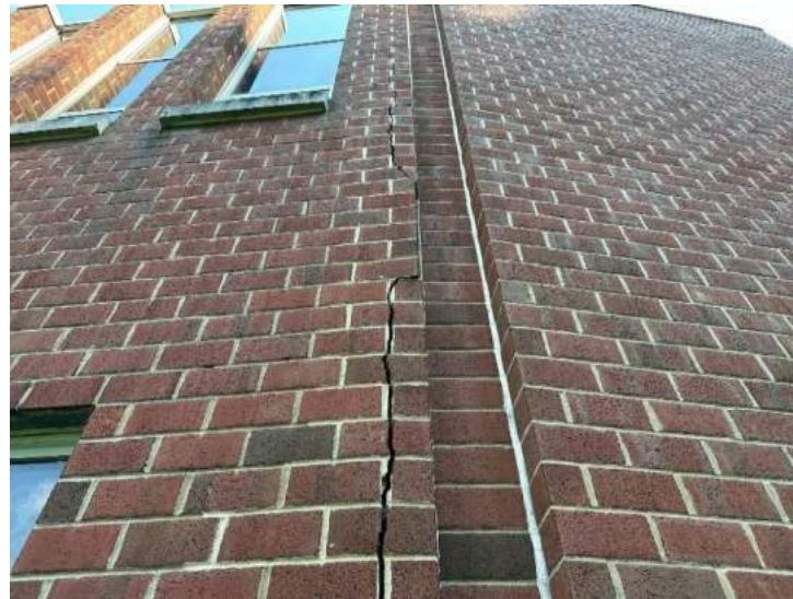
Water penetration/cracked brick
