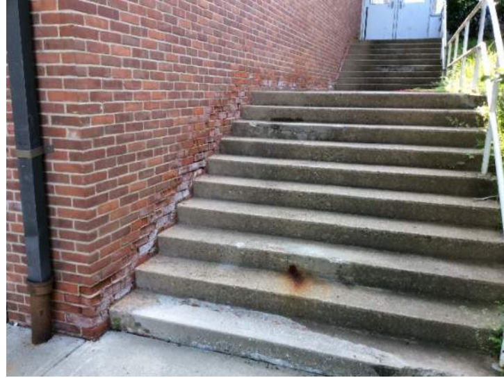
Spalling brick, exterior Steps/railing
