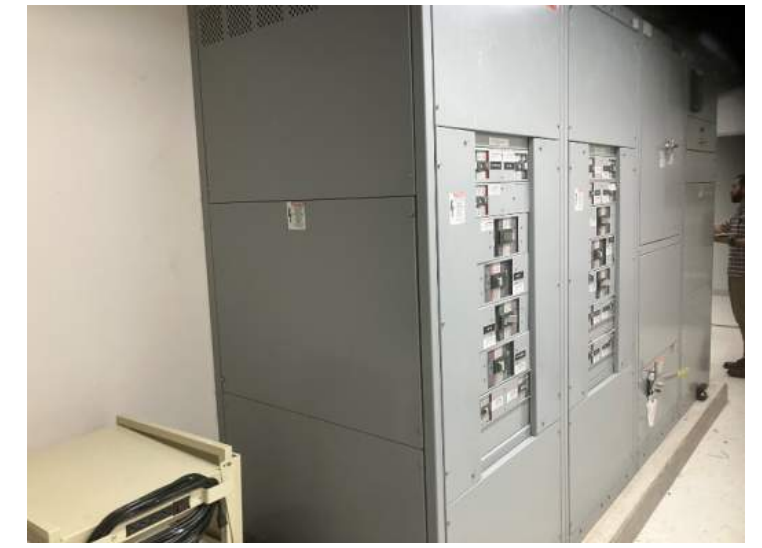
Old Electrical Mains
