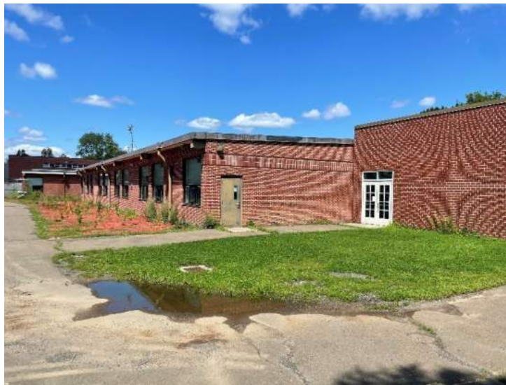
Poor site drainage
