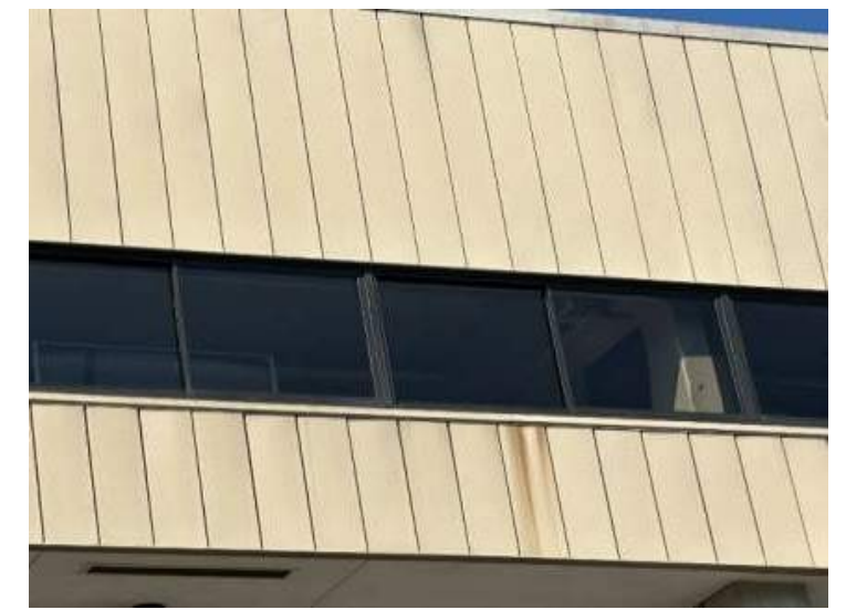
Aged-out siding and windows
