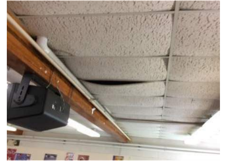
Acoustic tiles affected by humidity
