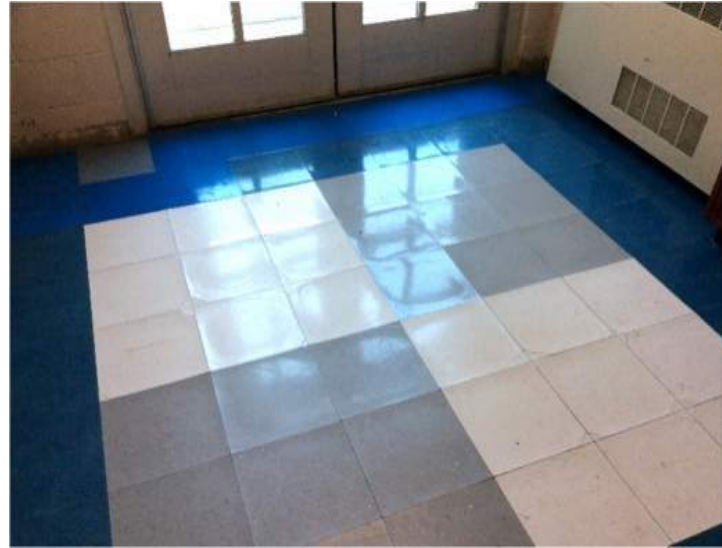
Vinyl tile affected by moisture
