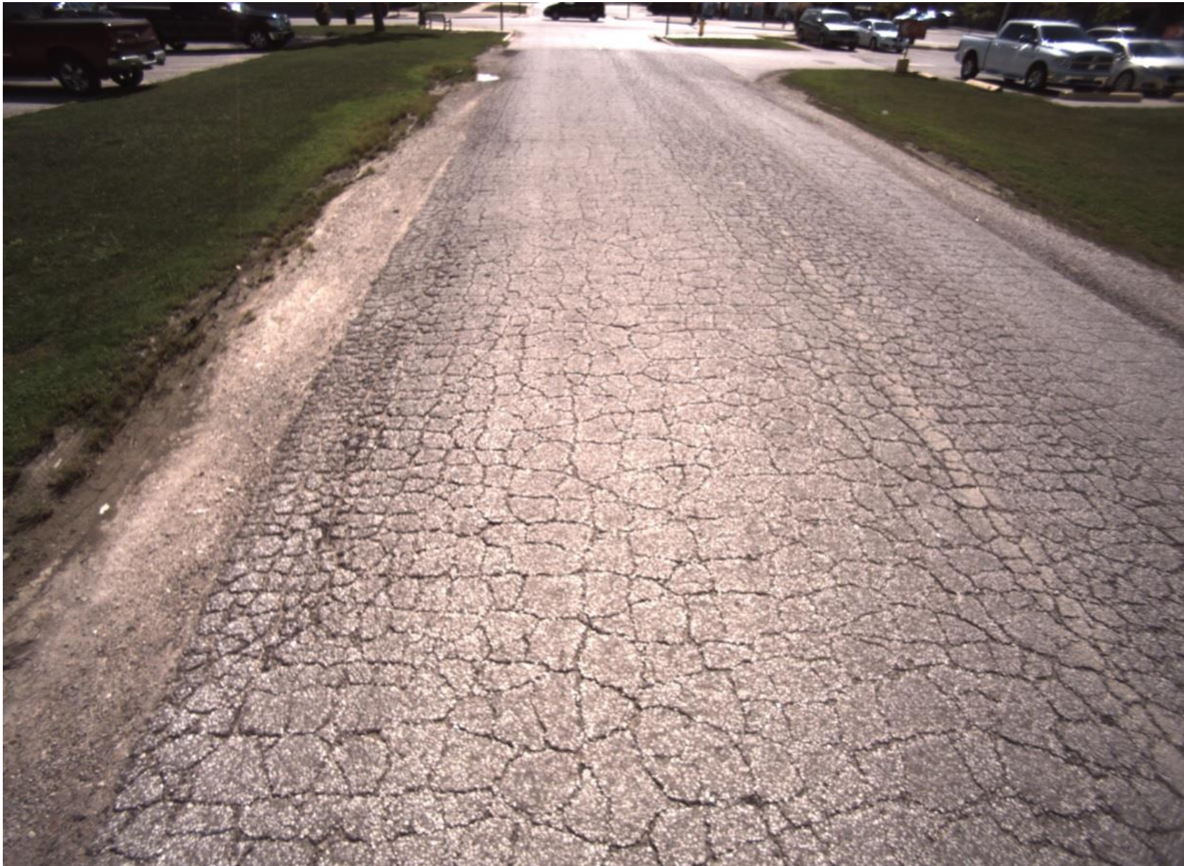
Sample serious/failed road – (0-25) (Dark Red & Gray)
