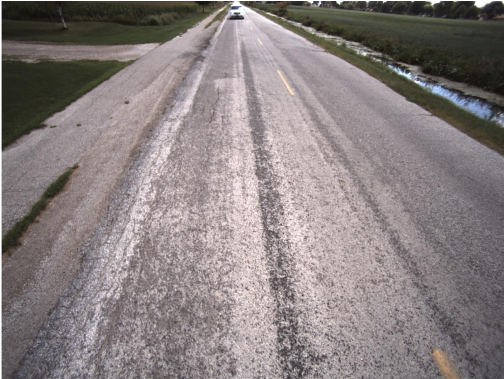
Sample poor road – (41-55) (Orange)
